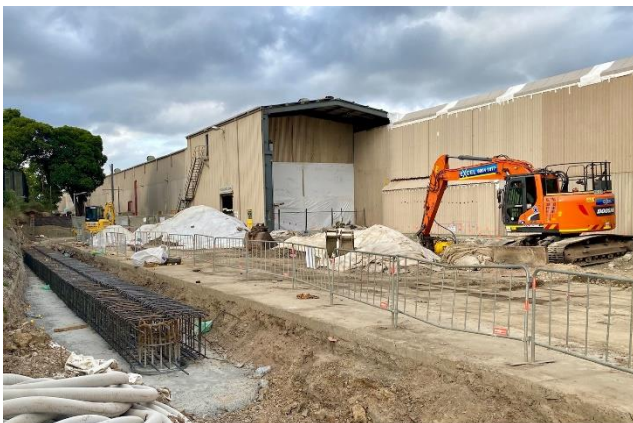
Installation of reinforcement cage in preparation for the capping beam concrete pour.
