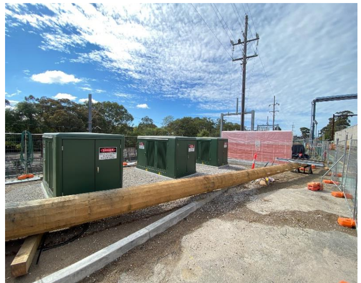
New substation equipment installed in the Maintenance Centre.
