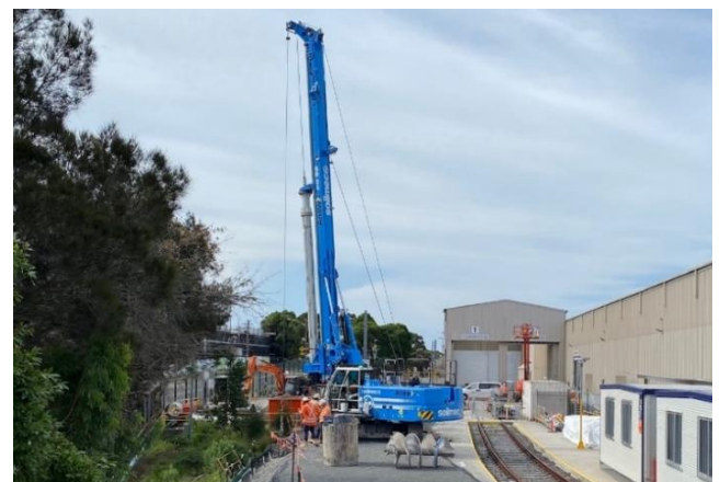
A new piling rig arrived from Europe to assist in construction of retaining walls and building foundations inside the centre.
