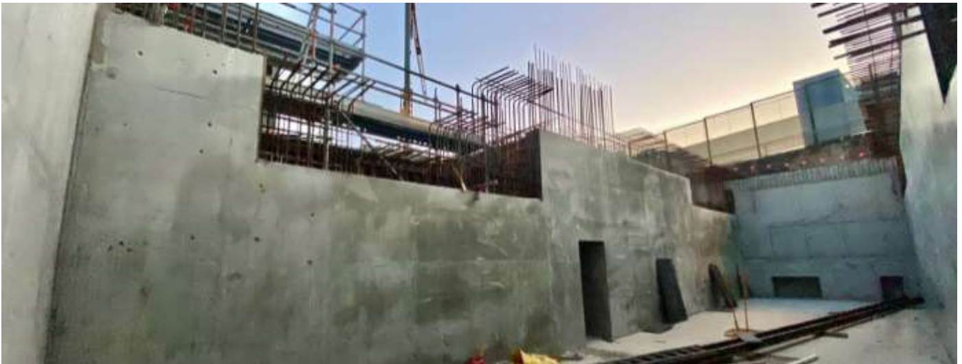
Photo taken from inside the tunnels constructed for the new bogie exchange system – Mortdale Maintenance Centre – September 2021
