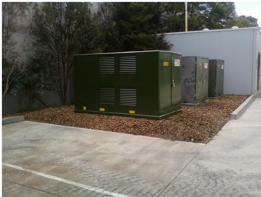
Figure 3.2 Example of padmount substations. The new padmount substations would be similar in size to this example.
