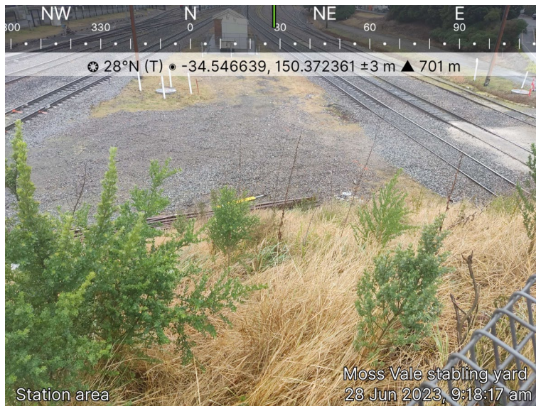
Figure 6-16 Vegetation on the track embankment looking north from the Lackey Road bridge
