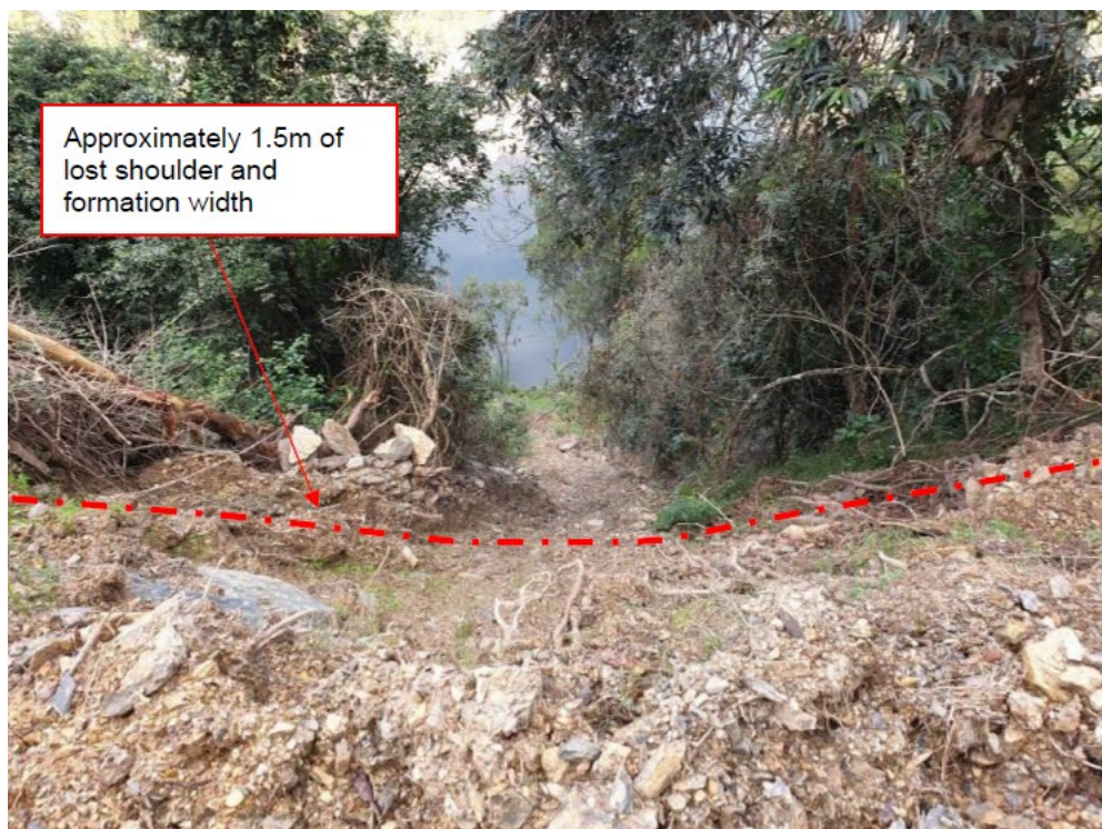
Figure 4.1 DM00231 – Downslope failure extends >100m downslope
