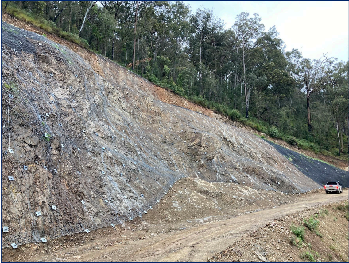
Big Hill Slip - Photo of rock bolts and mesh as well as bolts and matting (far right)
