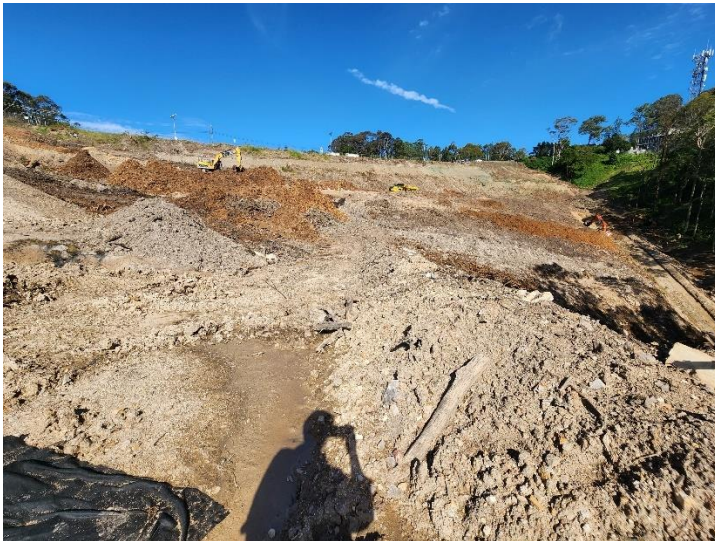
Image 7: Southern end. Clearing area to be filled showing soil contour banks, bunds and soil binder
