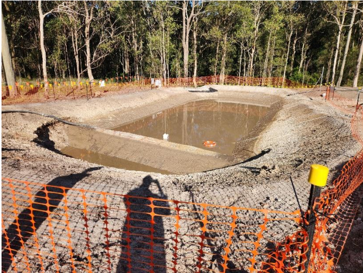
Image 5: Sediment basin located in the main clearing areas between Newcastle road and McCaffery Drive.
