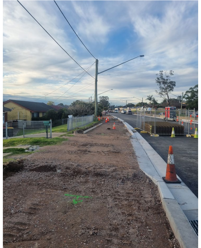
Preparation work for new shared user path between Keyworth Drive and Tudor Avenue
