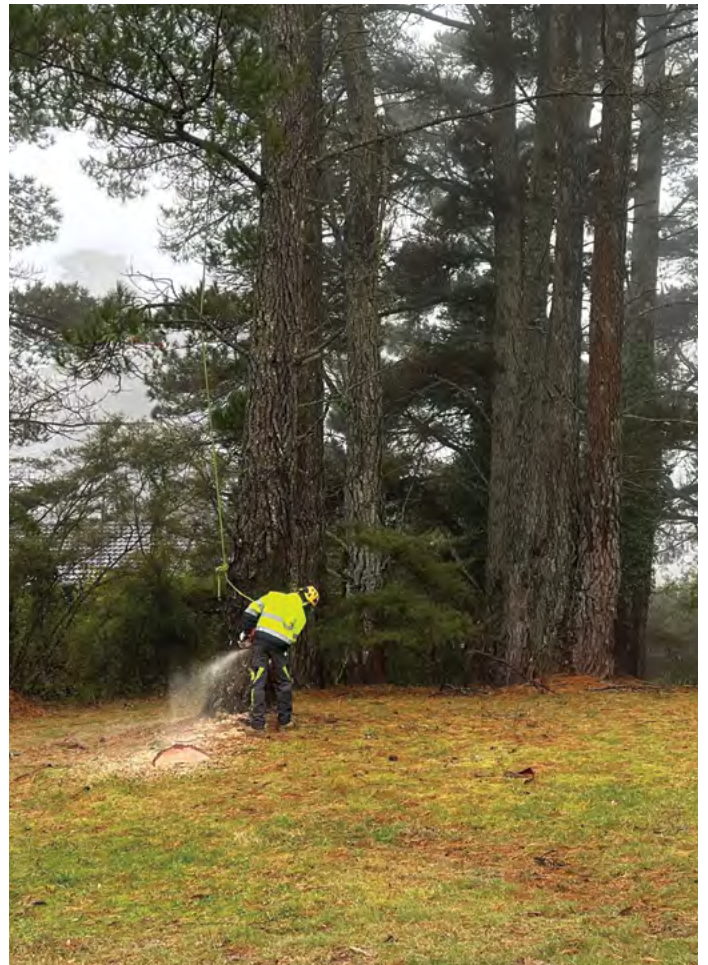
Pine tree removal underway to improve access for properties on the highway
