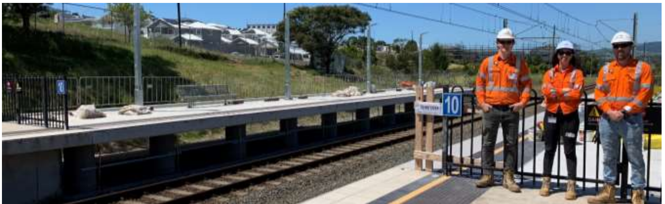
Staff standing at the end of the existing platform, with the extension progress shown behind the black fencing - Shellharbour Junction Station in November 2022.
