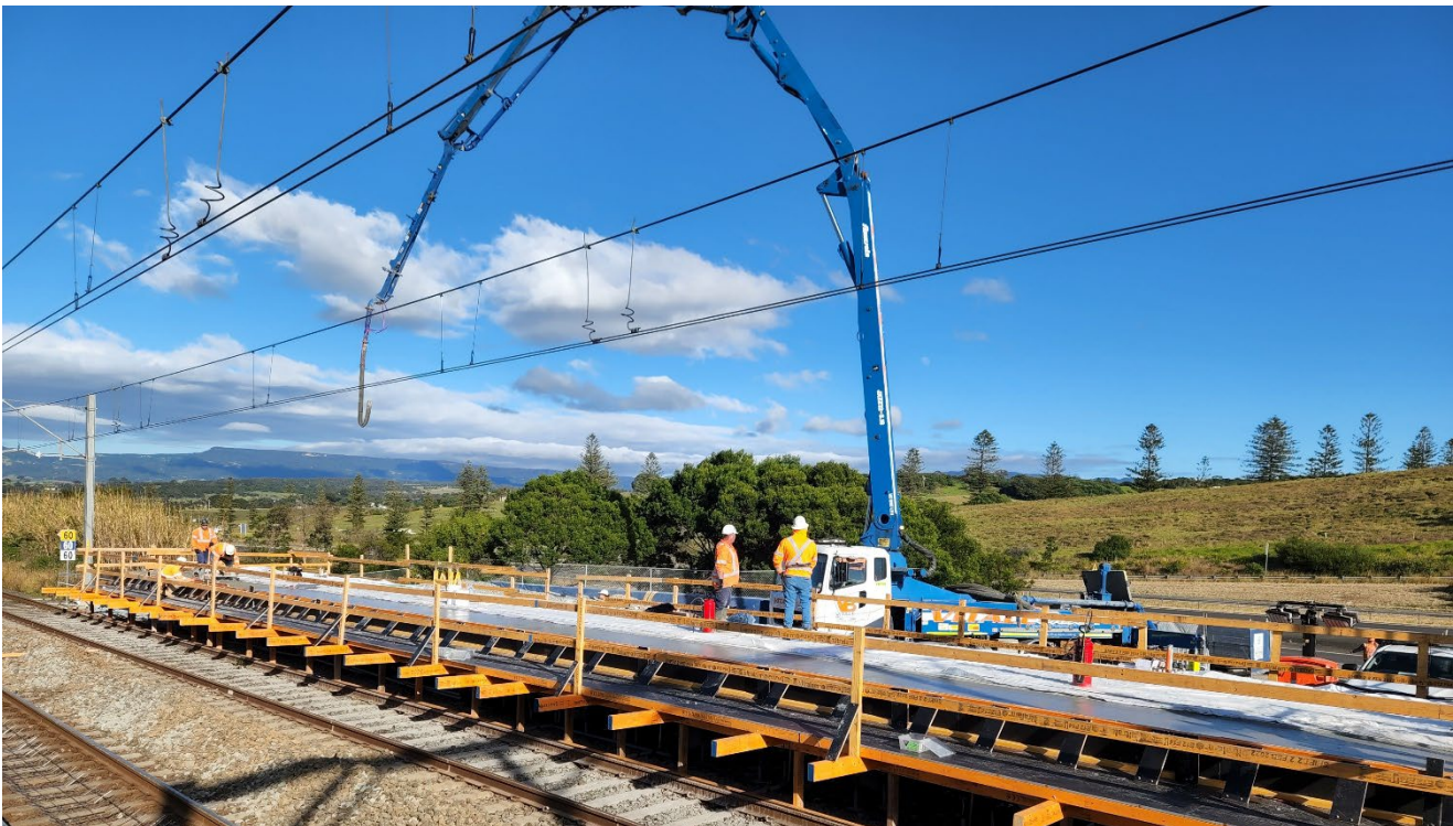
Concrete pour being undertaken at Shellharbour Junction Station for platform extension work in June 2022
