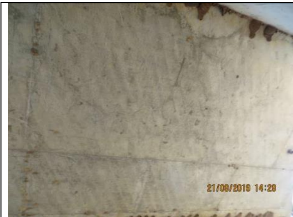
Photo 73 (257)_Cell 8_Deck soffit with longitudinal cracks
