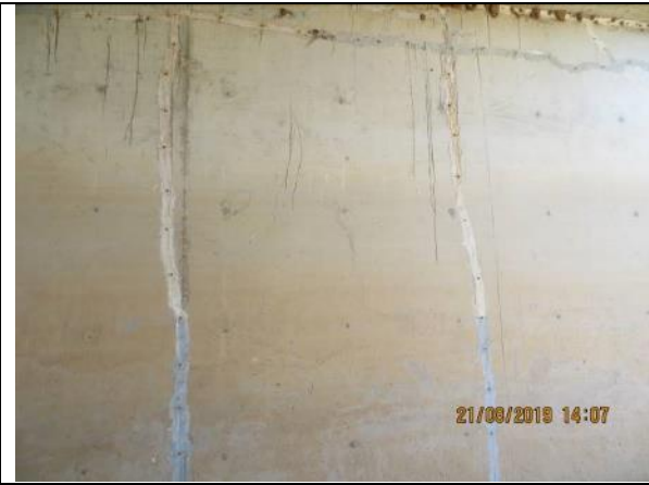
Photo 56 (191)_Cell 5_Wall B vertical cracks sealed and intact
