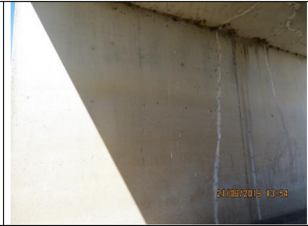
Photo 44 (155)_Cell 4_Wall A vertical cracks sealed and still intact
