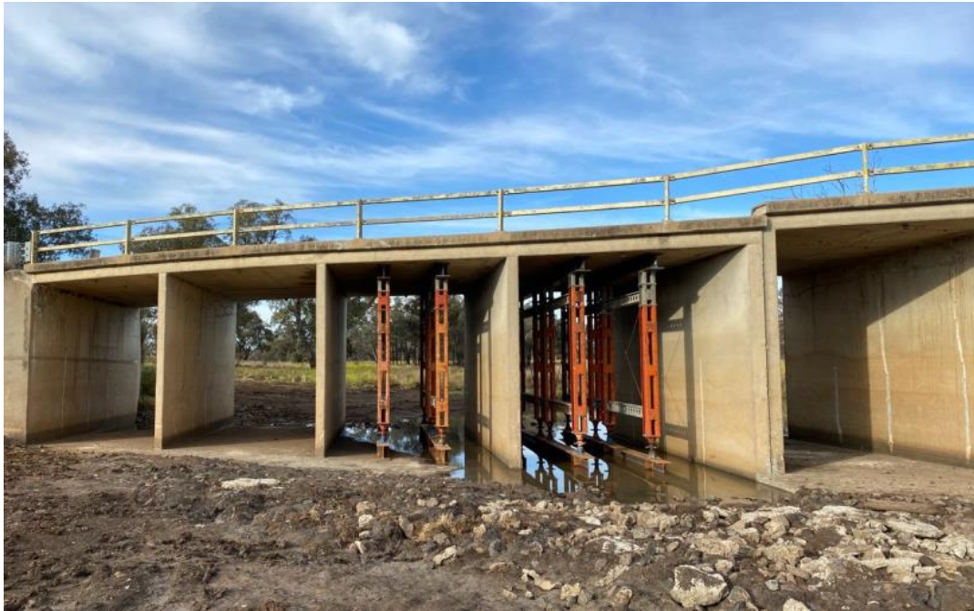
Figure 3-5: Temporary steel propping in cells 3 and 4 of the Spring Creek culvert structure (Transport, August 2021)
