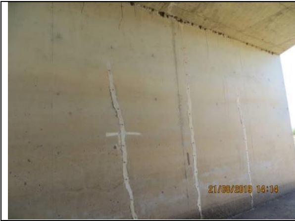
Photo 61 (213)_Cell 6_Wall B vertical crack sealed
