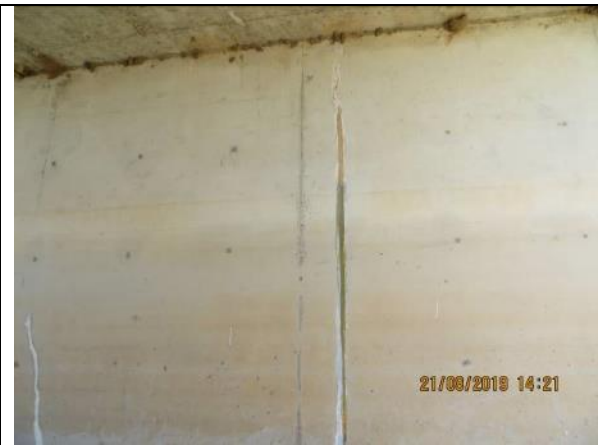
Photo 68 (232)_Cell 7_Wall B vertical cracks sealed and still intact
