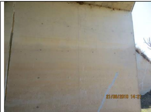
Photo 67 (231)_Cell 7_Wall B vertical cracks sealed and still intact
