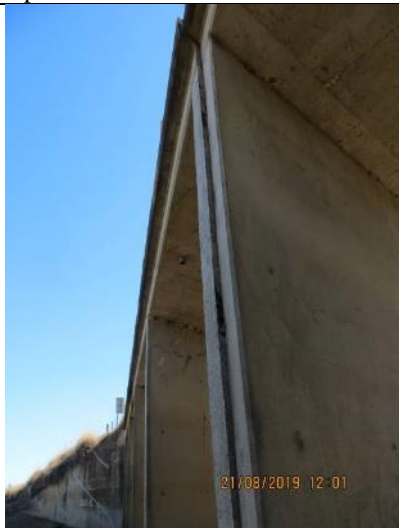
Photo 11 (68) Close up view of misalignment on Upstream side
