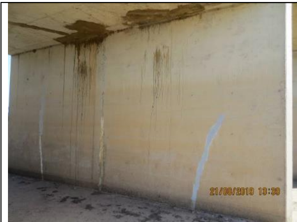
Photo 31(120)_Cell 2_Wall B vertical cracks sealed and still intact
