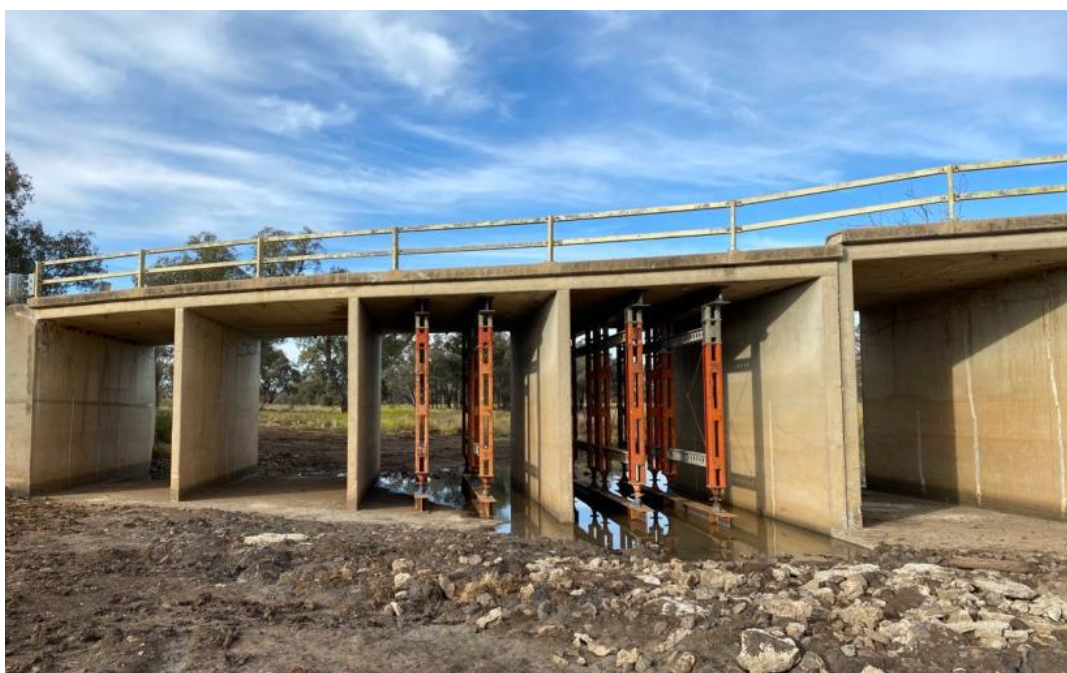
Figure 2-3: Temporary steel propping in cells 3 and 4 of the Spring Creek culvert structure (Transport)
