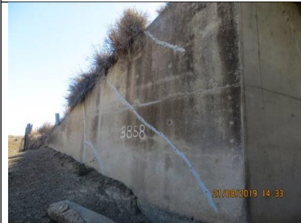
Photo 75 (277)_Abt B DS wing wall with cracks and crack at interface with deck
