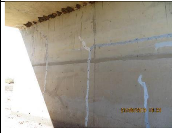
Photo 17 (86)_Cell1_Wall A_Abt A previous cracks sealed and still intact_new fine horizontal cracks
