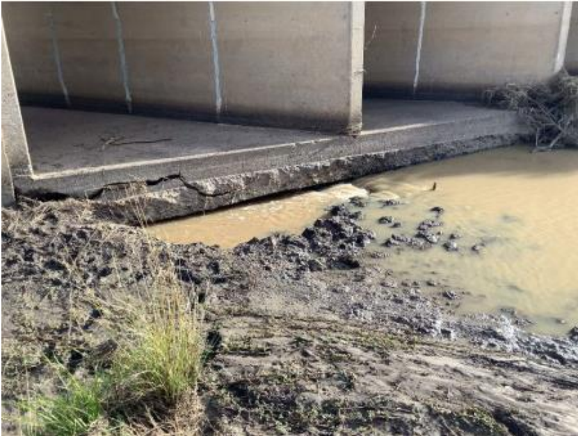
Figure 3-4: Water penetrating underneath the concrete base slab of the Spring Creek culvert structure (Transport, June 2021)
