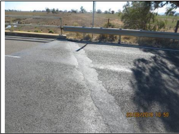
Photo 79 (285)_Above deck joint A, hump in Abt A joint
