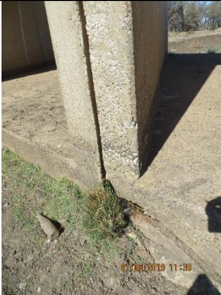
Photo 7(27) Misalignment is visible between the walls of Cell 4 & 5 due to rotational movement of the cells by flood
