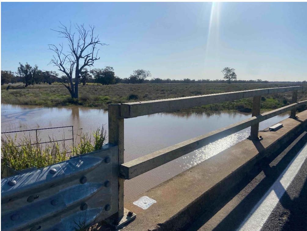
Photo 8 Spring Creek Bridge B3858 over Spring Creek. Yellow paint to metal rails on both ends of the bridge. Due to the homogenous nature of the paint, all yellow paint should be assumed to contain lead content exceeding the assessment criteria of 0.1%w/w. Paint was found in fair condition.
