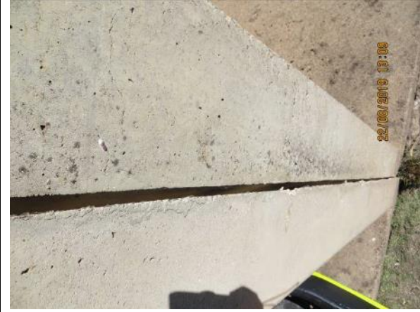
Photo 90 (356)_Wall between Cell 4 and Cell 5_Gap decreasing down towards_Fine cracks on face of US wall
