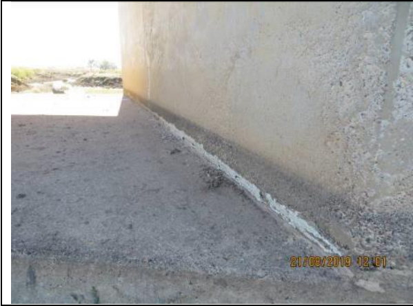
Photo 13 (73) Cell 5 invert slab and wall interface with crack reappear after sealing
