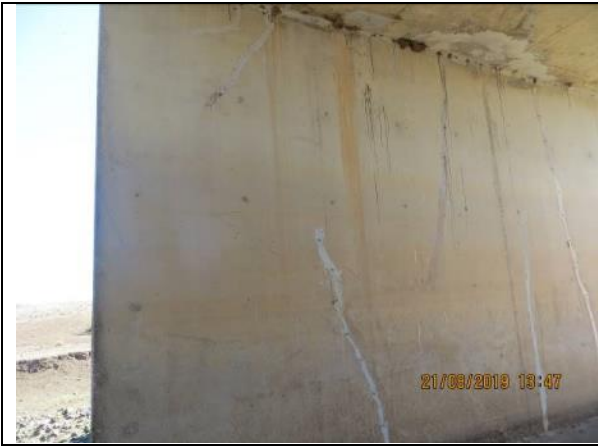
Photo 37 (136)_Cell3_Wall B cracks sealed and still intact
