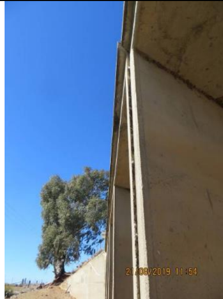
Photo 8 (28) Misalignment is visible between the walls of Cell 4 & 5 due to rotational movement of the cells by flood
