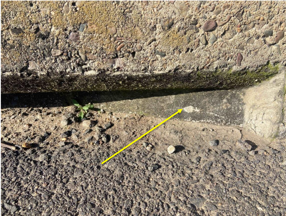
Photo 3 Spring Creek Bridge B3858 over Spring Creek. Sample location A1 – Moulded fibre cement to the surrounds of the scuppers (throughout).
