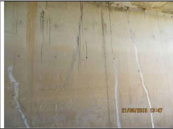
Photo 38 (137)_Cell 3_Wall B cracks sealed and still intact
