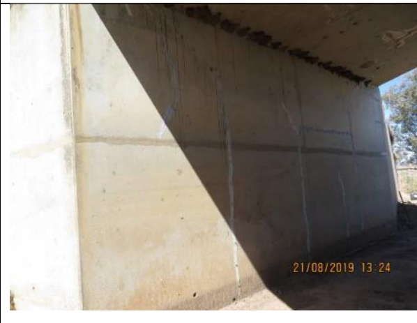
Photo 18 (87)_Cell1A_AbtA previous cracks sealed intact_new fine horizontal cracks
