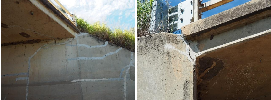
Figure 3-2 Abutment and wing wall cracks (Source: FBE)
