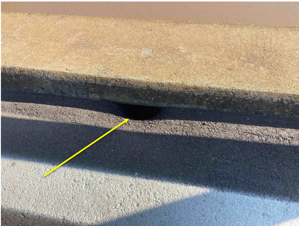
Photo 4 Spring Creek Bridge B3858 over Spring Creek. Some of the fibre cement surrounds to the scuppers were hard to access. These were completely sealed off with new bitumen layer. All moulded fibre cement surrounding of the scuppers, including areas where it has been sealed off be removed prior to any demolition works.
