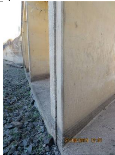
Photo 12 (69) Close up view of misalignment on Upstream side
