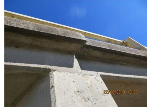
Photo 89 (0348)_Wall between Cell 4 and Cell 5_Gap decreasing down towards_Fine cracks on face of US wall
