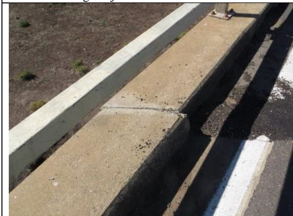
Photo 87 (344) Kerbs misalignment at joint between Cell 4 & 5
