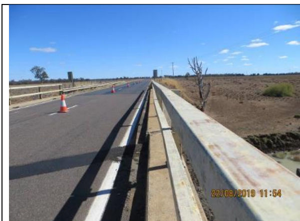
Photo 85 (327)_US handrail deviation towards DS at middle of bridge at joint
