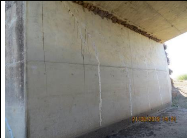
Photo 77 (270)_Cell8_AbtB_wall with vertical cracks sealed
