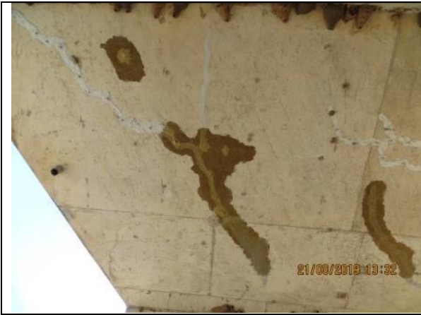
Photo 25 (107)_Cell 1_Deck Soffit mesh/ transverse and irregular cracks
