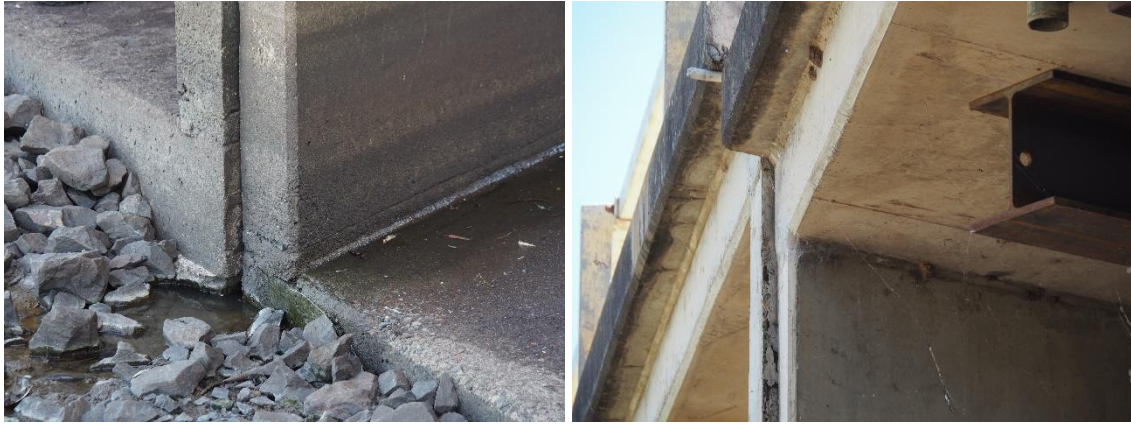
Figure 3-4 Segment misalignment (Source: FBE)
