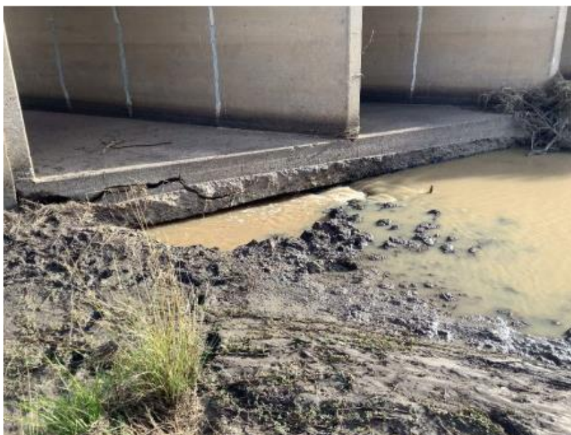
Figure 2-2: Water penetrating underneath the concrete base slab of the Spring Creek culvert structure (June 2021) (Transport)
