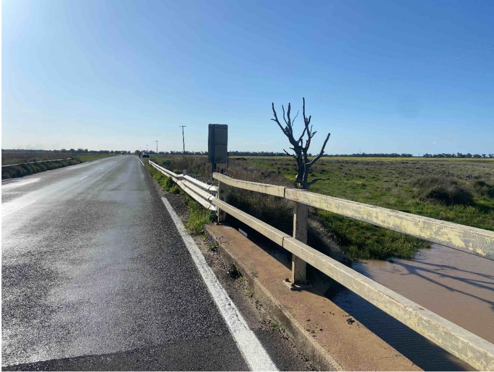
Photo 7 Spring Creek Bridge B3858 over Spring Creek. Yellow paint to metal rails on both ends of the bridge. Due to the homogenous nature of the paint, all yellow paint should be assumed to contain lead content exceeding the assessment criteria of 0.1%w/w. Paint was found in fair condition.
