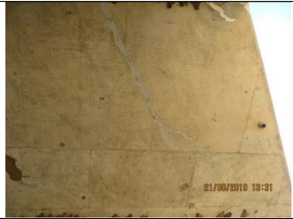
Photo 26 (105)_Cell 1_Deck Soffit mesh/ transverse and irregular cracks
