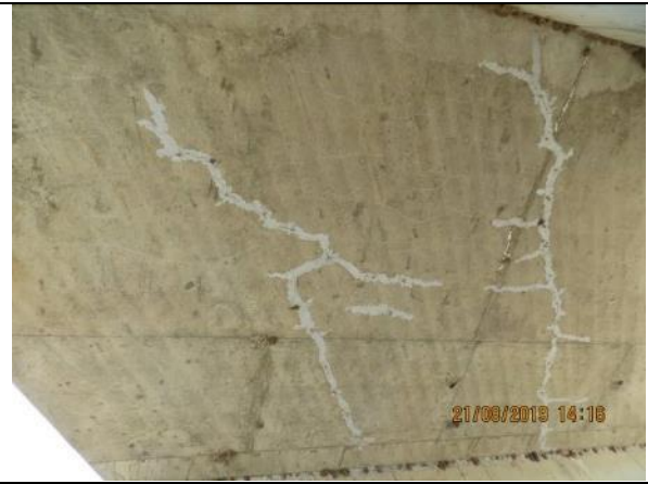
Photo 62 (221)_Cell 6_Deck soffit, longitudinal cracks primarily sealed and still intact, traverse cracks appear in mesh pattern
