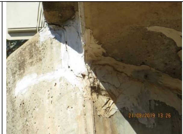
Photo 20 (95)_Crack at deck soffit interface with wing wall
