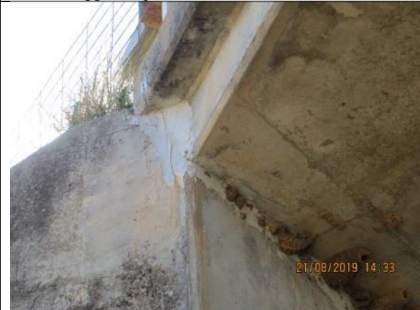
Photo 78 (279)_AbtB DS wingwall with cracks and crack at interface with deck
