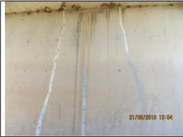
Photo 43 (153)_Cell 4_Wall A vertical cracks sealed and still intact
