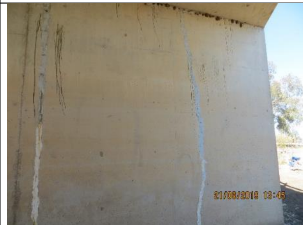
Photo 36 (128)_Cell 3_Wall A cracks_sealed and still intact
