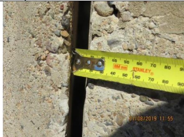
Photo 10 (63) Close up view of misalignment on Upstream side
