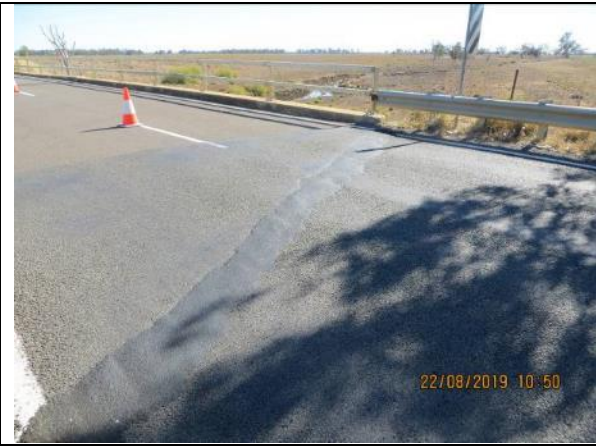
Photo 80 (287)_Above deck joint A, hump in Abt A joint
