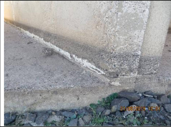
Photo14 (74) Cell 5 invert slab and wall interface with crack reappear after sealing
