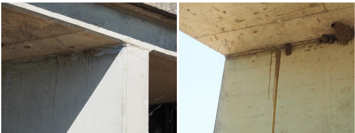
Figure 3-3 Cell wall cracks (Source: FBE)
