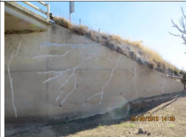
Photo 76 (264)_Cell 8_Abt B US wing wall with some cracks reappearing
