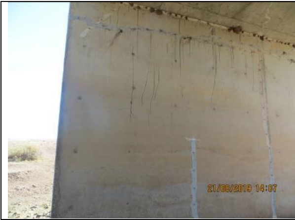
Photo 55 (189)_Cell 5_Wall B vertical cracks sealed and intact
