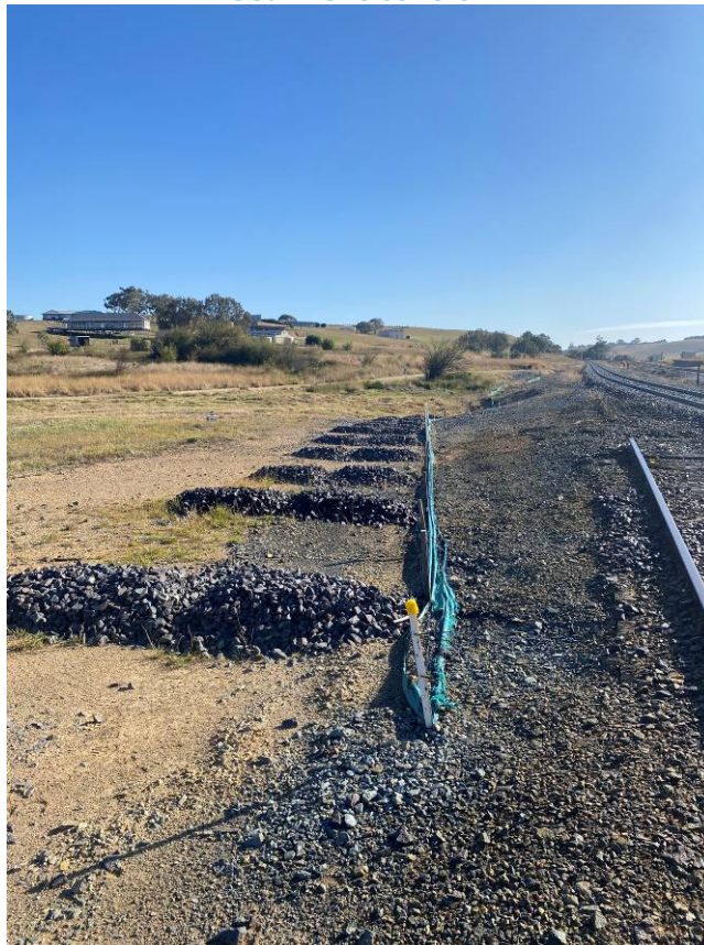
Photo 8: Rock checks and silt fences running alongside former Woodlawn siding towards the middle culvert. No sediment build up on rock checks or fencing.
