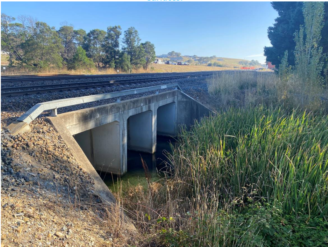
Photo 2: Immediately downgradient of southernmost culvert showing pooled water, not flowing off site. High reeds and vegetation adding natural filters for sediment.
