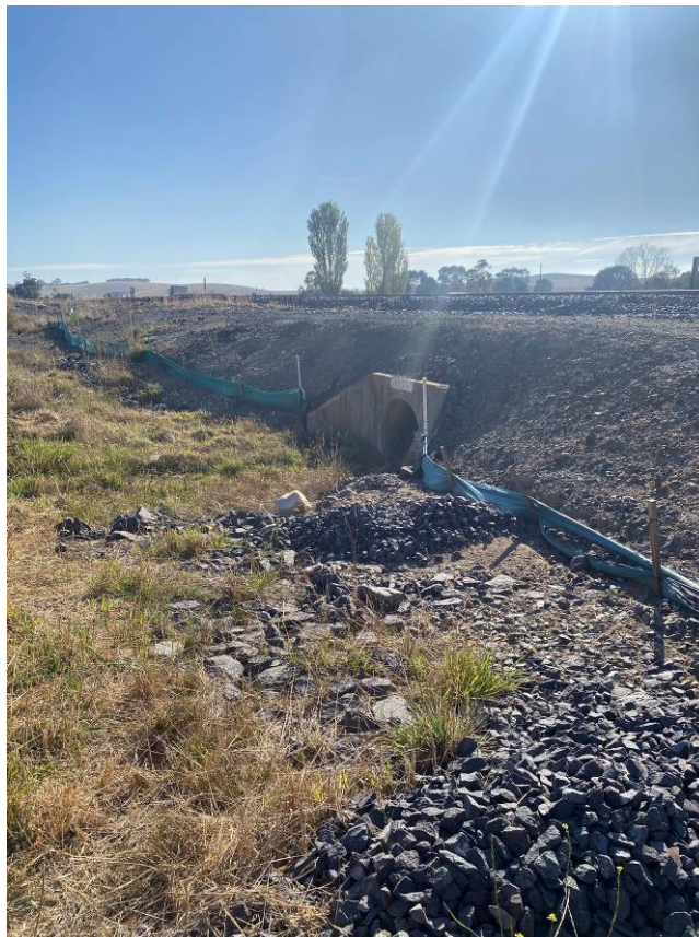
Photo 9: Upgradient of middle culvert, showing sediment control measures of rock checks and silt fencing.
