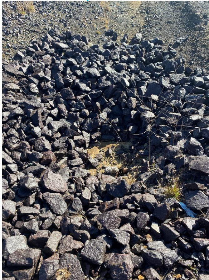
Photo 20: Inlet of drain from centre of railroad tracks showing minor signs of sediment.
