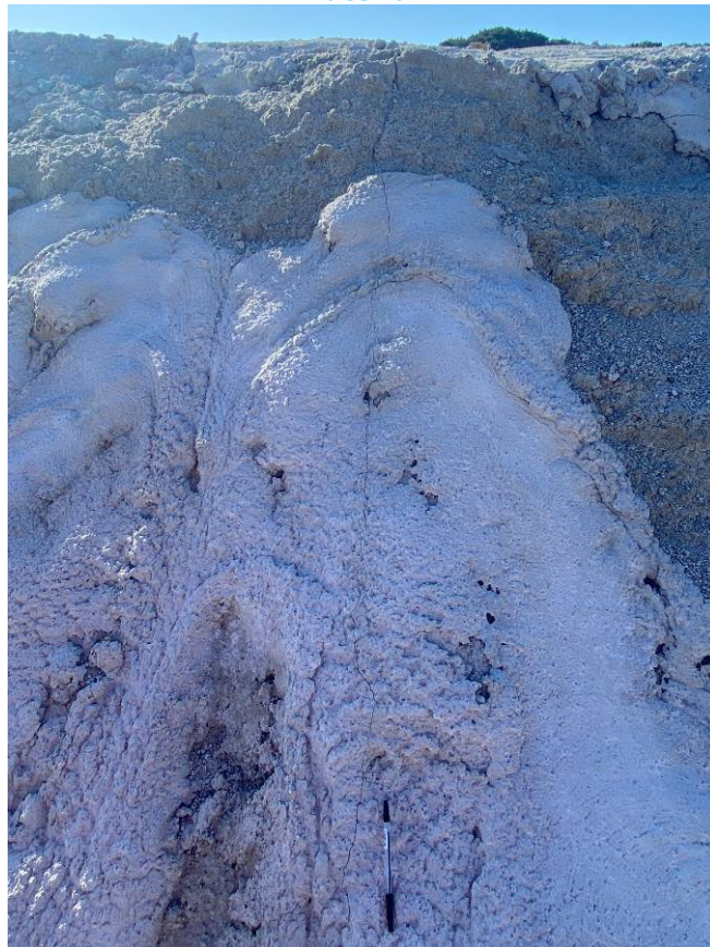
Photo 14 Hairline cracking in stabilised sand applied to the stockpile for capping. Pen used for sizing reference.
