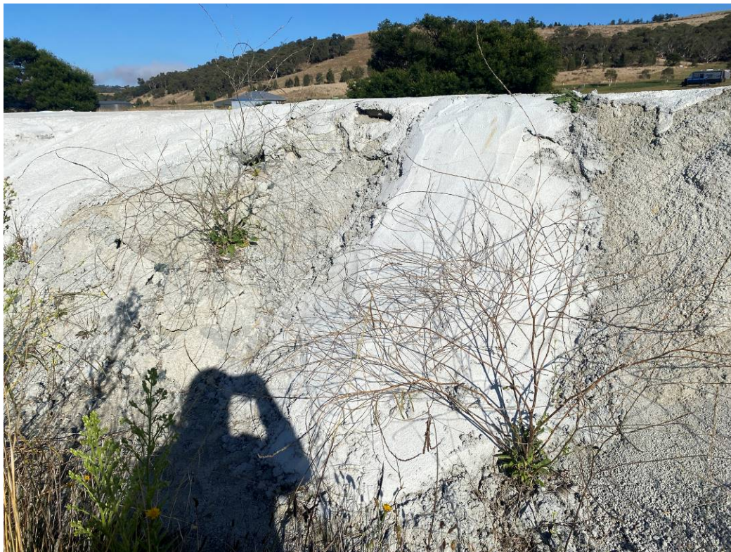
Photo 15: Vegetation (weeds) growing out of stockpile capping. No marker layer visible.
