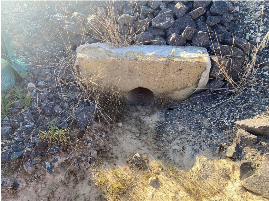
Photo 19: Outlet of drain from centre of railroad tracks showing minor signs of sediment. Water would flow through drain pipe to upgradient of the railway culverts and then through sediment controls in place at the culverts.
