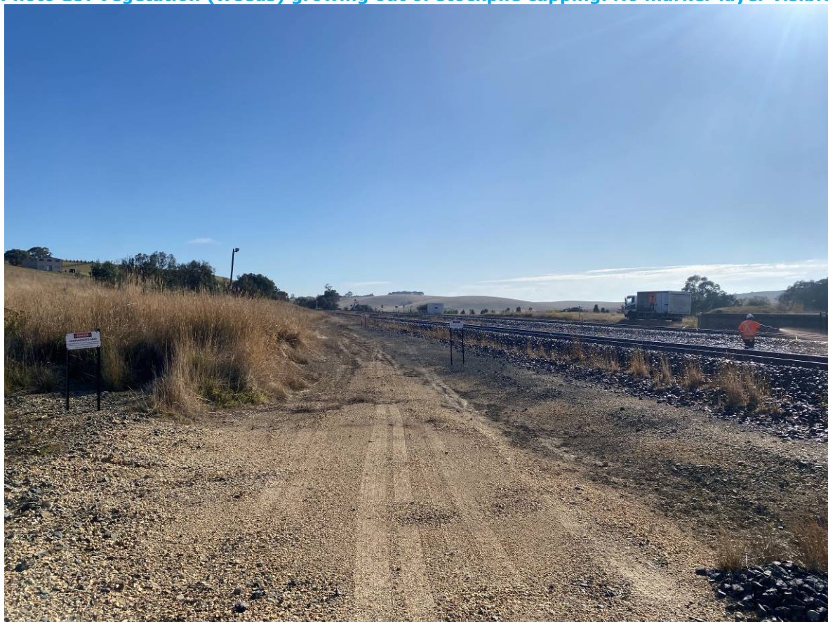
Photo 16: Polymer Sealant application in progress. Sprayed through hose by contractors onto railways and surrounding areas.
