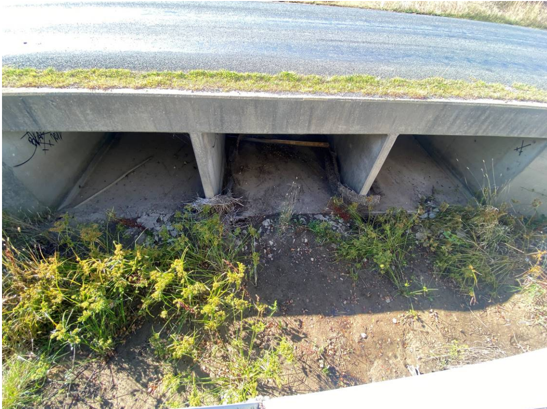
Photo 3: Culvert under Golburn street, downgradient of southernmost culvert on site, showing no evidence of surface water run off on site and no evidence of sediment from previous surface water on site.
