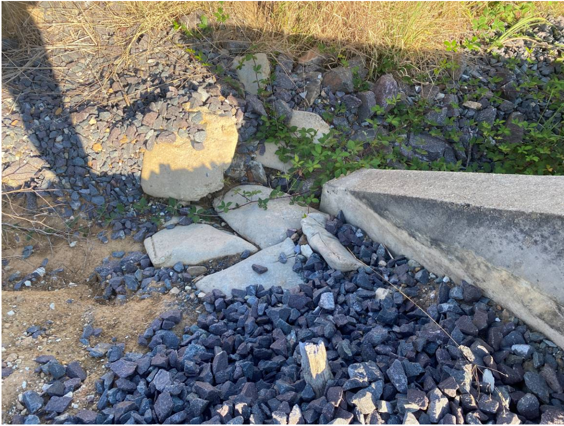
Photo 7: Upgradient of southernmost culvert showing rock armour used as control measures for sediment control.
