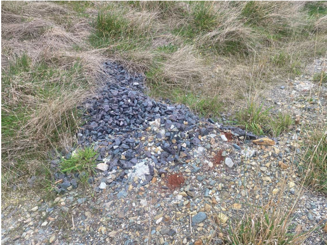
Photo 27. Build-up of sediment in rock armoury. Ramboll recommends replacing new rock armoury.
