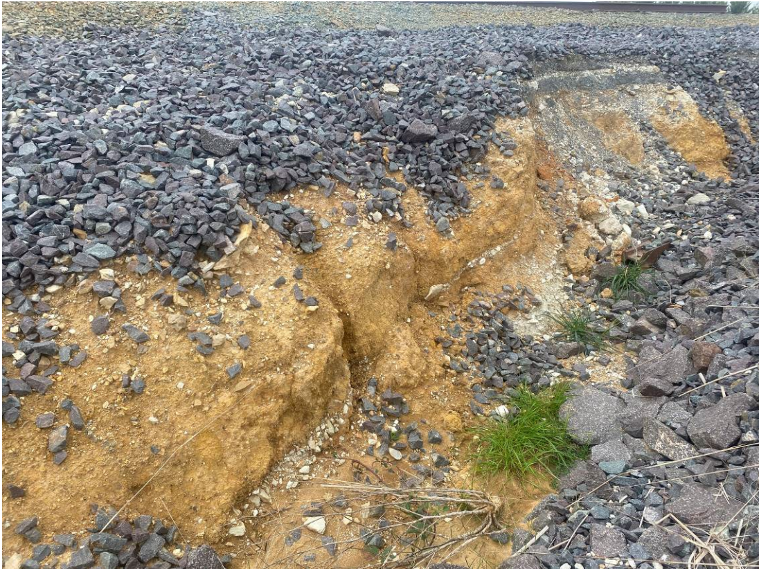
Photo 25. Visible evidence of erosion created by loss of ground cover (ballast material on top) upgradient of southernmost culvert. No visible evidence of sediment in water downstream of culvert despite erosion evidence.
