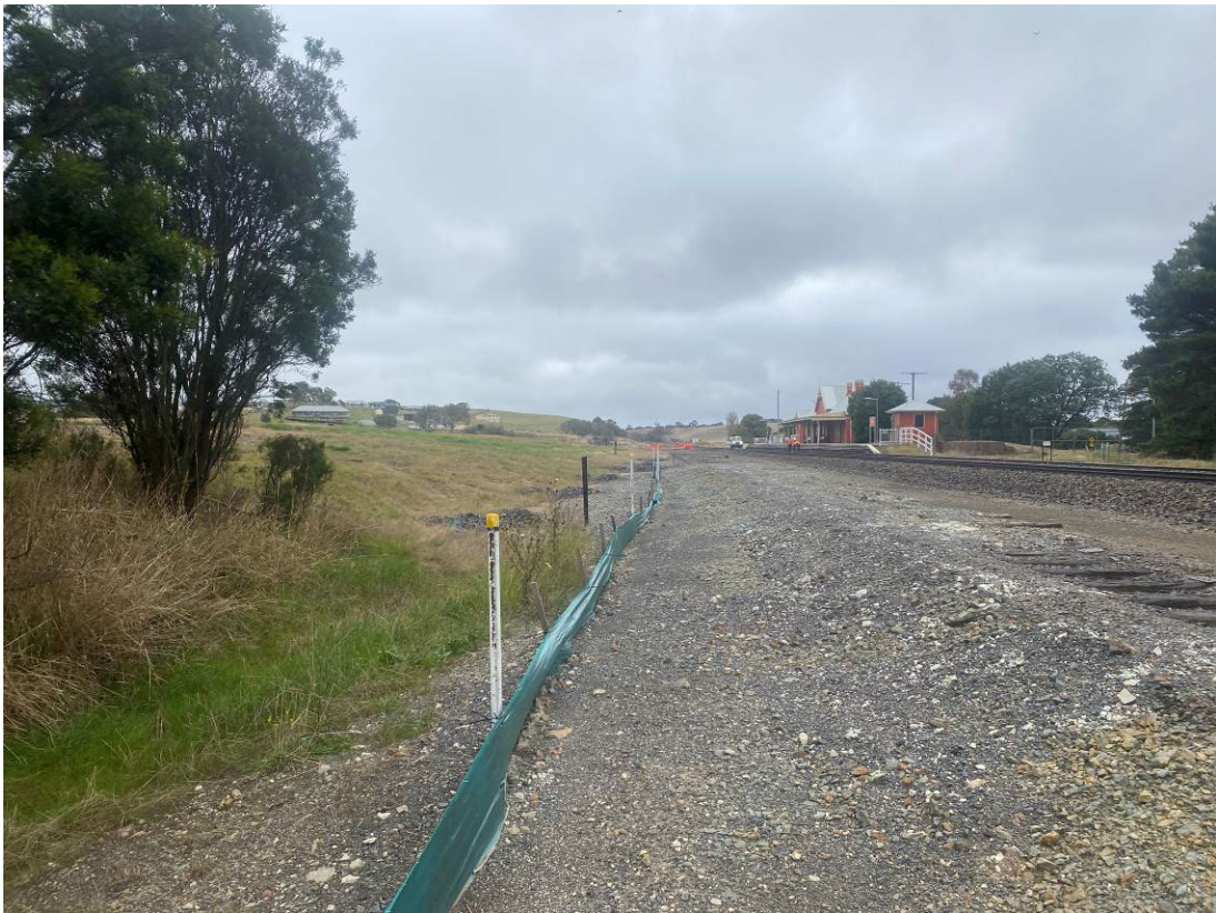
Photo 10: Rock checks and silt fences running alongside former Woodlawn siding towards the middle culvert. Moderate sediment build up on rock checks or fencing.
