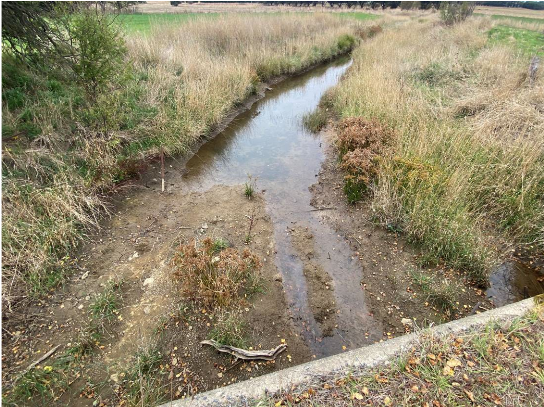
Photo 4: Outlet of culvert under Golburn street, downgradient of southernmost culvert on site, showing evidence of minor surface water run off on site. Water remains clear with no observable sediment.
