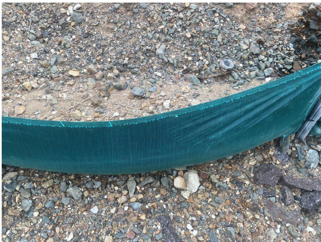
Photo 30. Build-up of sediment in silt fencing armoury. Ramboll recommends removing silt above fencing using a shovel.
