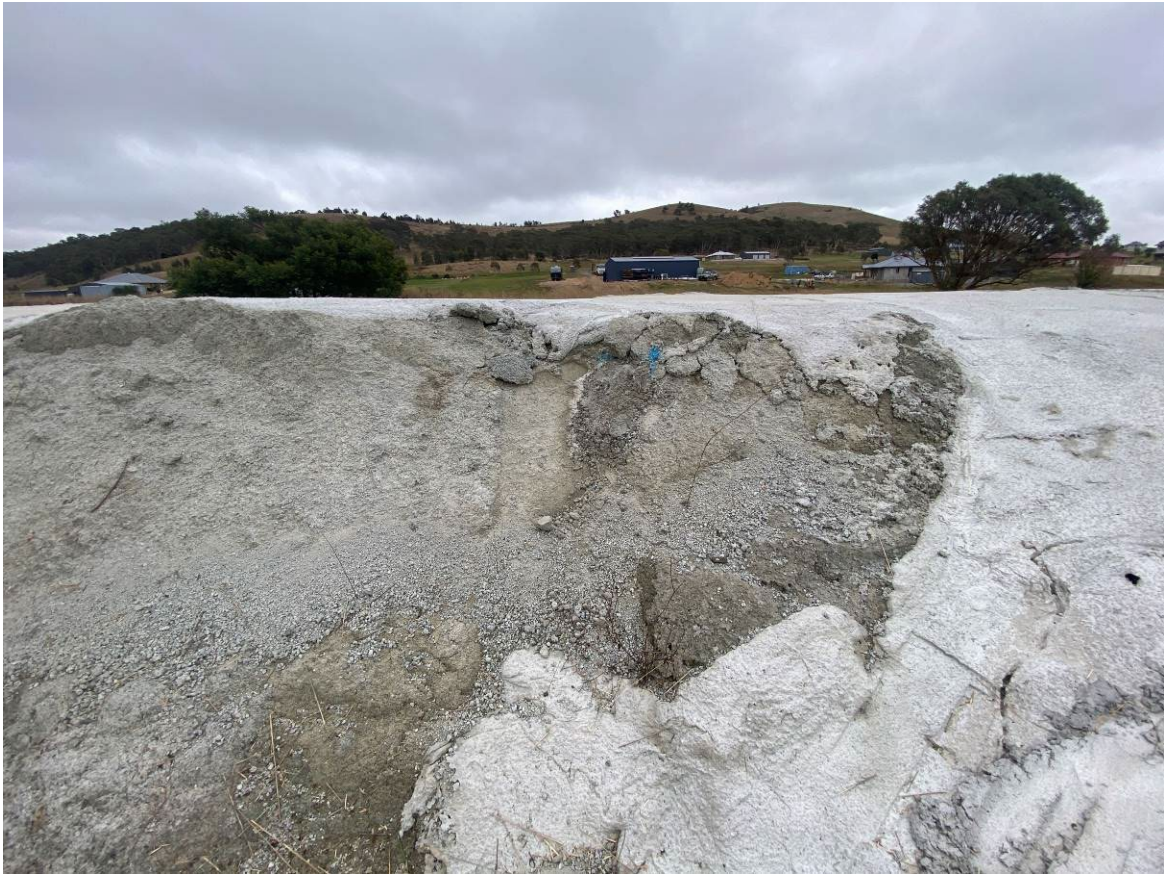
Photo 23. Geofabric marker layer previously visible has been patched as per recommendations from Inspection Checklist dated 28-Mar-23.
