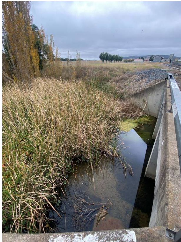
Photo 2: Immediately downgradient of southernmost culvert. Very slow surface water run off from site. Water was clear with no turbidity and no visible sediment. High reeds and vegetation adding natural filters for sediment.
