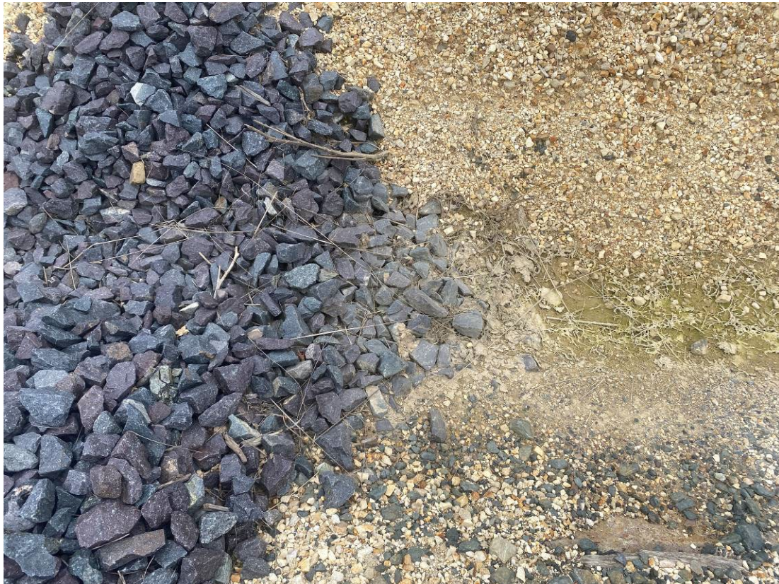
Photo 28. Build-up of sediment in rock armoury. Ramboll recommends adding additional rocks to armoury.
