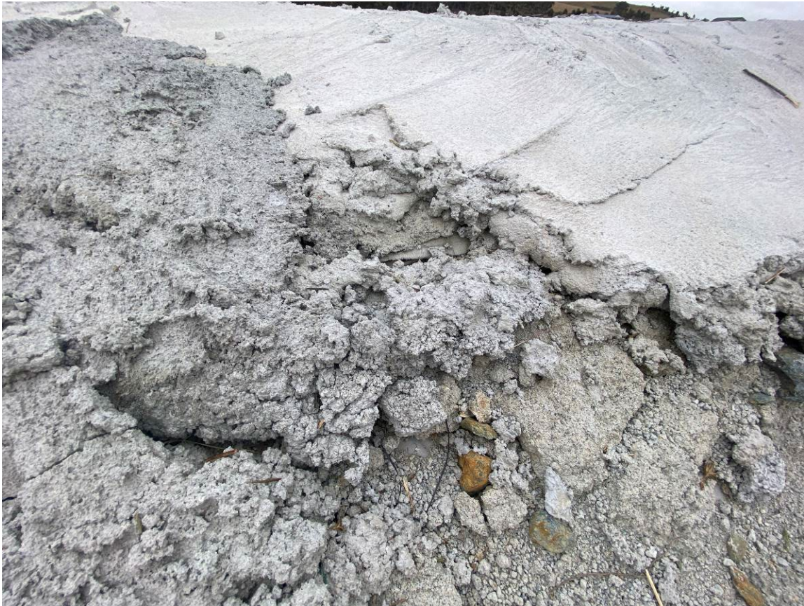
Photo 21. Geofabric marker layer visible in stockpile capping UGL on site representative was notified and marked this with spray paint. Approximately 8cm x 1.5cm.
