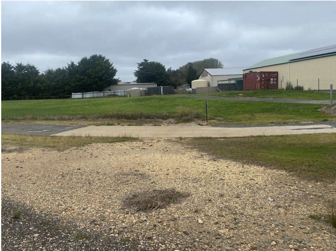
Photo 7: Causeway downgradient of middle culvert showing no evidence of current surface water run off on site. No visible sediment on road or vegetation nearby.
