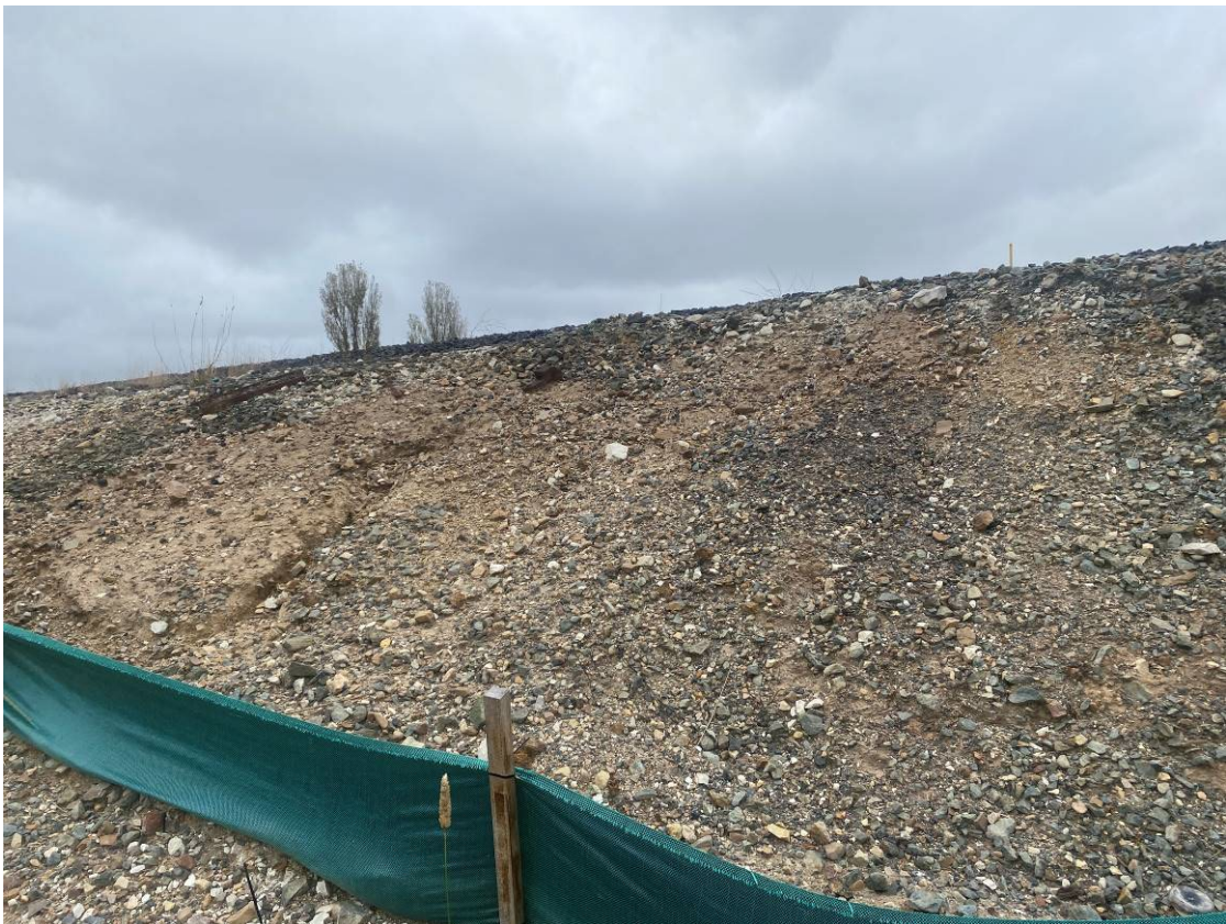
Photo 14: Silt fencing north of the middle culvert. Some erosion evidence of soil and build up of sediment on silt fencing.
