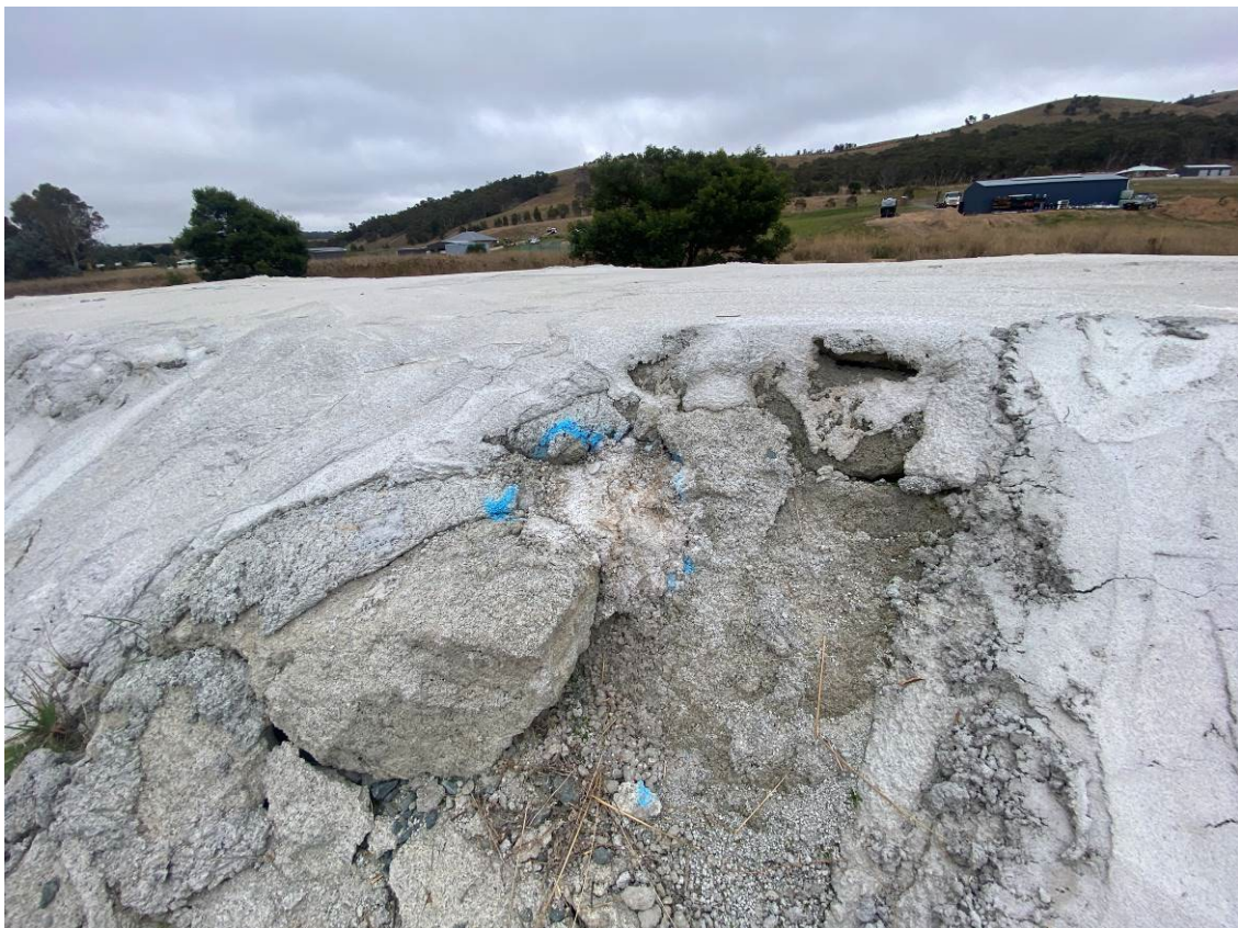
Photo 22. Geofabric marker layer previously visible has been patched as per recommendations from Inspection Checklist dated 28-Mar-23.
