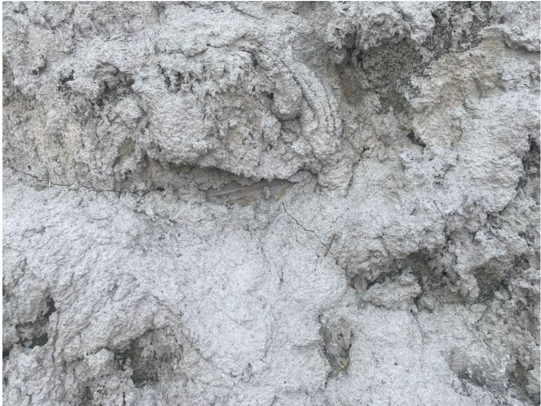
Photo 19 Hairline cracking in stabilised sand applied to the stockpile for capping. Geofabric marker layer visible. UGL on site representative was notified and marked this with spray paint. Approximately 10cm x 2cm.
