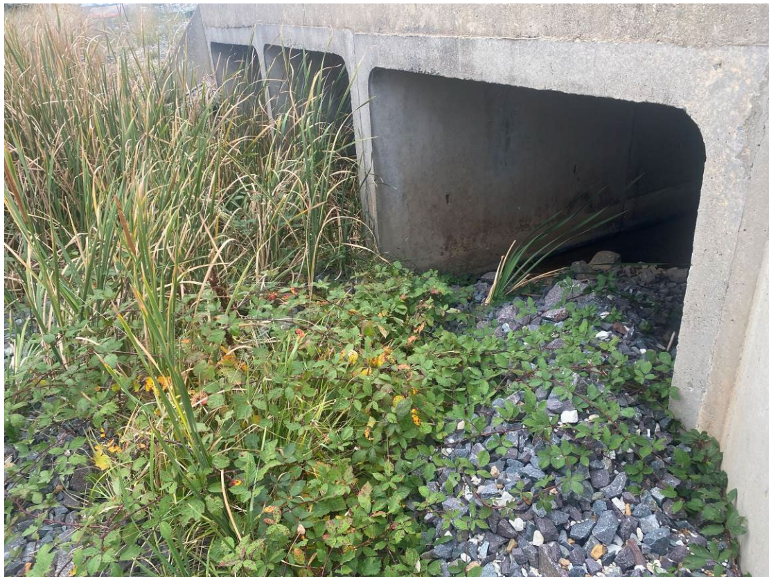
Photo 8: Upgradient of southernmost culvert showing evidence of minor surface water run off on site. No visible sediment observed beyond rock armoury.
