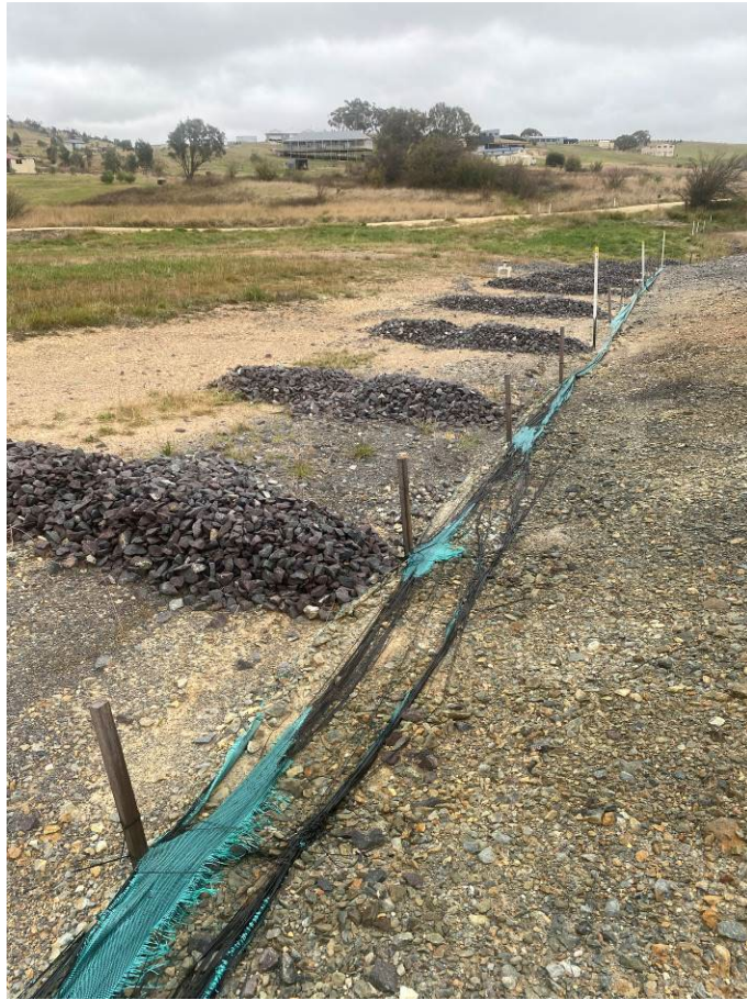
Photo 11: Rock checks and silt fences running alongside former Woodlawn siding towards the middle culvert. Major damage to silt fencing remaining on southern side. No evidence of sediment build-up in rock armoury.
