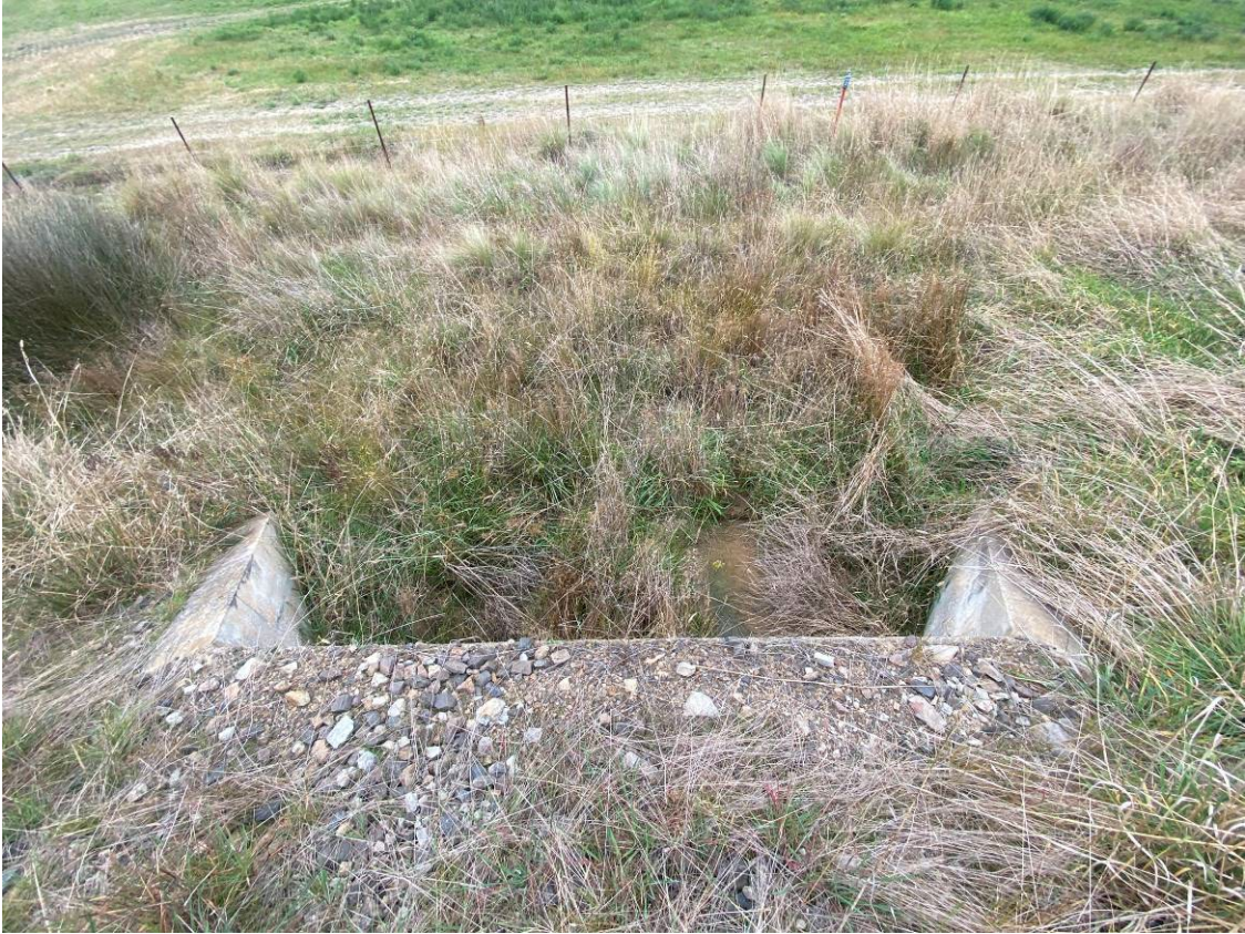
Photo 5: Downgradient of northernmost culvert facing private property, showing no evidence of surface water run off on site and no evidence of sediment from previous surface water on site.
