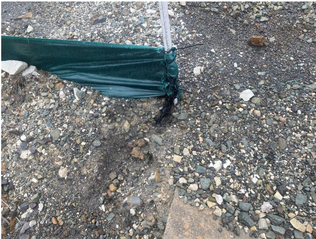
Photo 26. Visible evidence of erosion due to silt fencing diverting water. No visible evidence of sediment in water downstream of culvert despite erosion evidence. Ramboll recommends removal of silt above fencing to allow better water flow.
