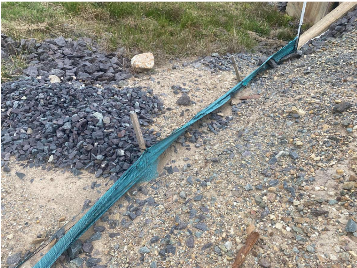
Photo 29. Build-up of sediment in silt fencing armoury. Ramboll recommends removing silt above fencing using a shovel.
