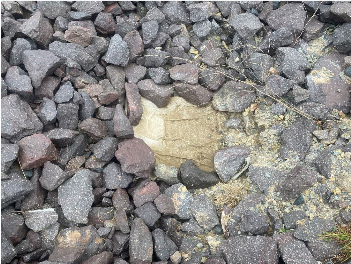
Photo 15: Geofabric filter over drain inlet between the main and loop lines as per recommendations from Inspection Checklist dated 15-Mar-23. Evidence of sediment capture.
