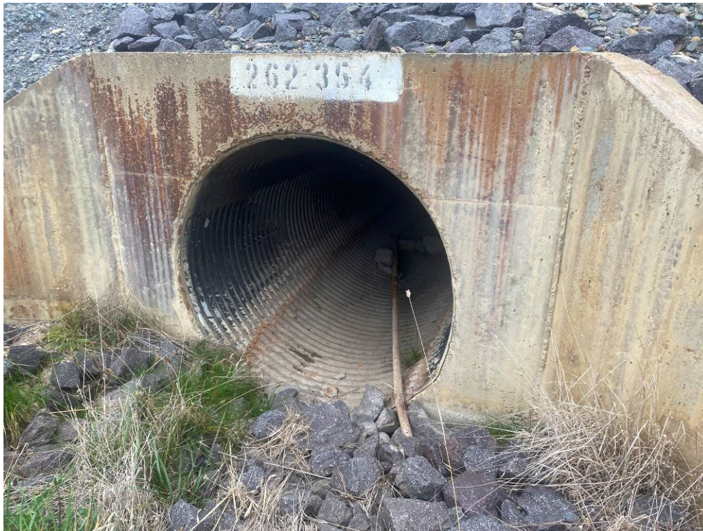
Photo 12: Upgradient of middle culvert showing minor signs of sediment in rock checks but no surface water discharge from site.
