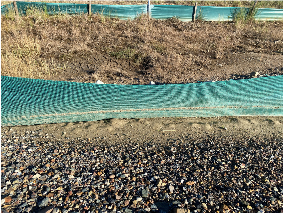
Photo 13: Sediment build up captured by silt fencing upgradient of middle culvert prior to drainage trench. Approximately 1cm build up.
