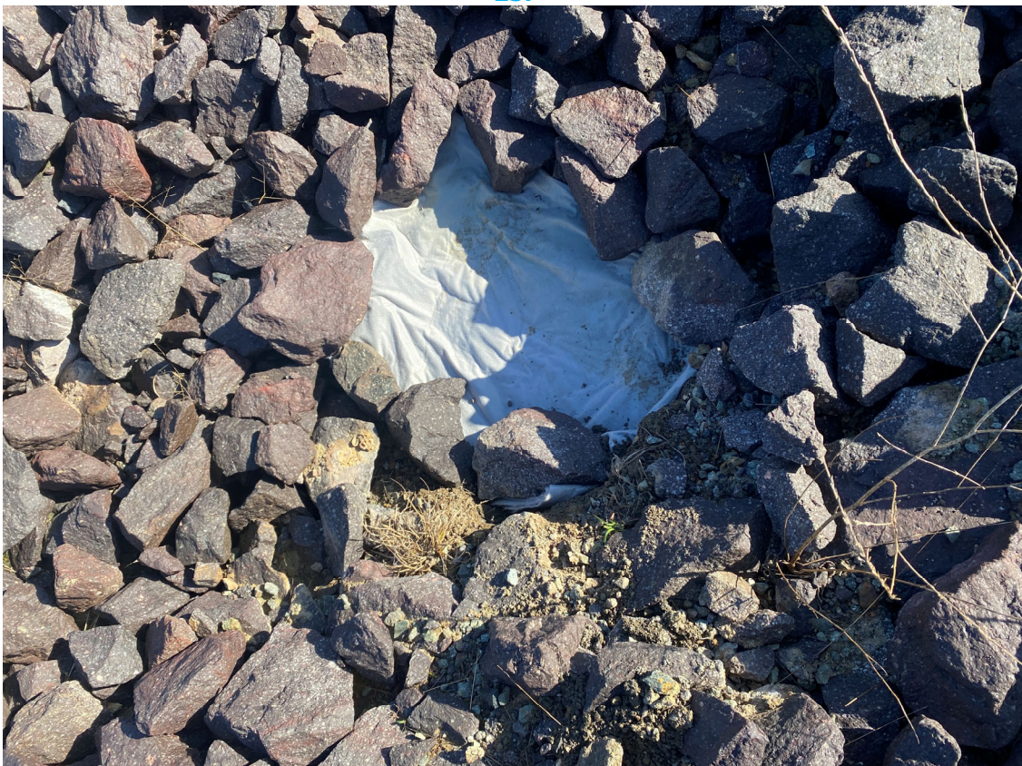
Photo 20: UGL on site. Placed geofabric filter over drain inlet between the main and loop lines as per recommendations from Inspection Checklist dated 15-Mar-23.
