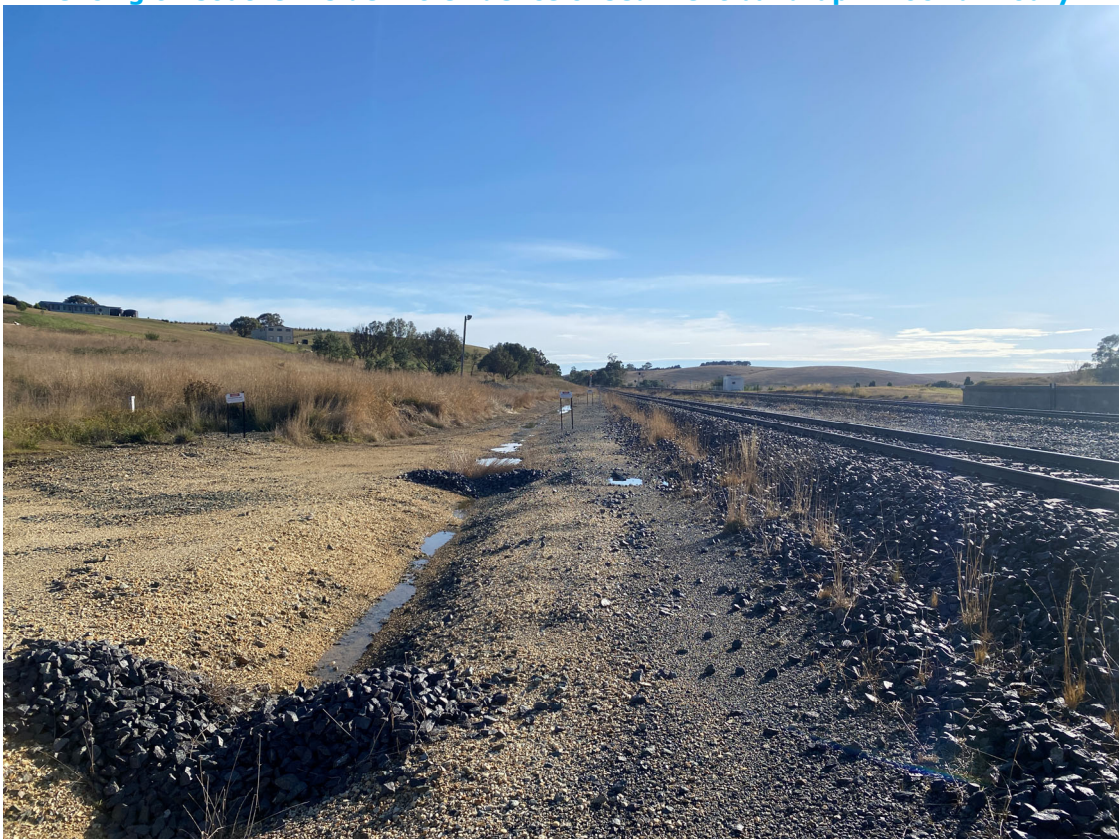
Photo 12: Pooled water with no sediment and sediment control measures of rock armoury within drainage trench towards northernmost culvert.
