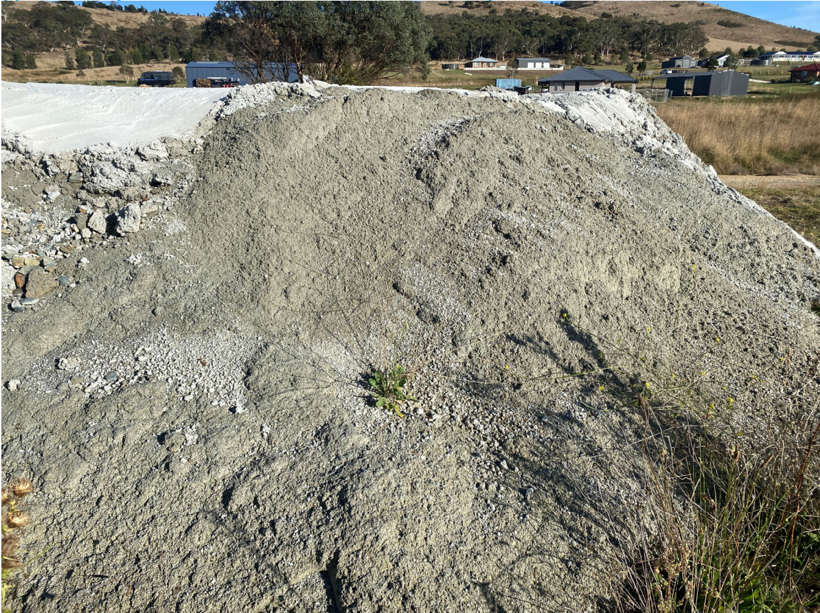
Photo 16: Minor vegetation (weeds) growing out of stockpile capping. No marker layer visible.
