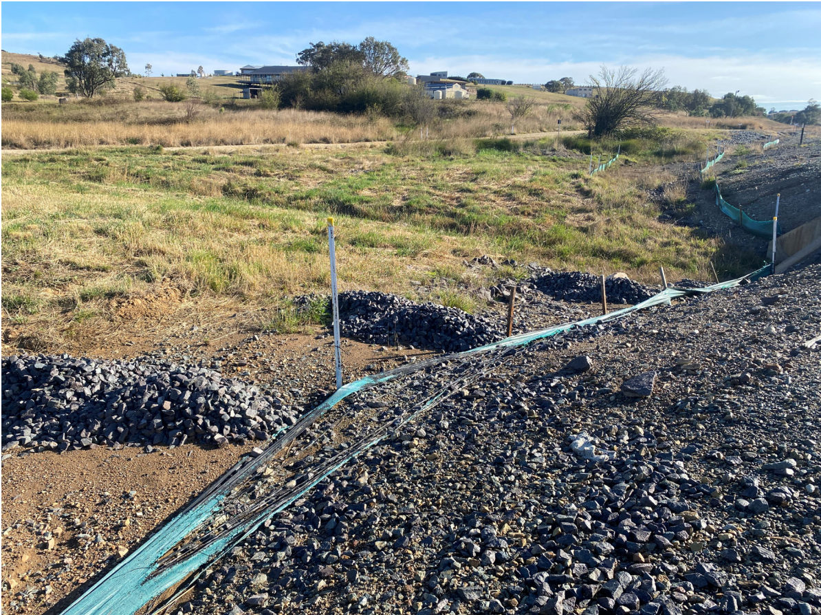
Photo 11: Rock checks and silt fences running towards the middle culvert. Major damage to silt fencing on southern side. No evidence of sediment build-up in rock armoury.
