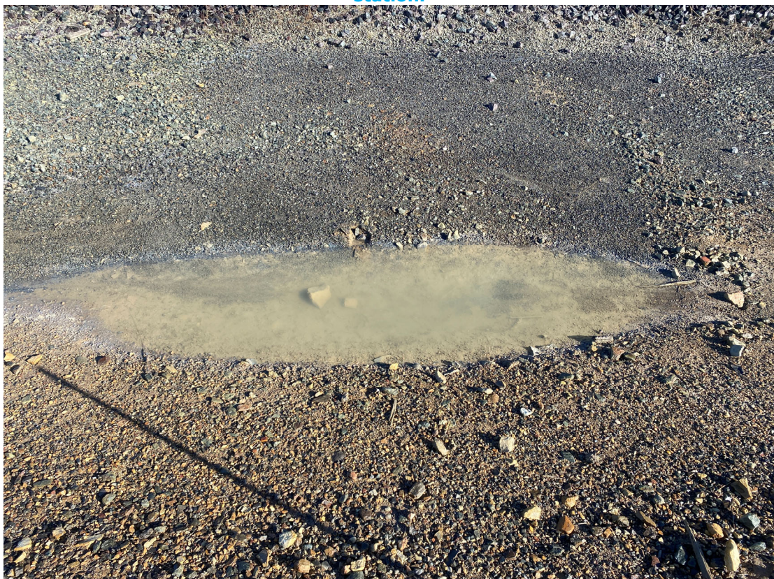
Photo 2: Minor sediment in pooled water between rail tracks. Not flowing off site and located prior to sediment controls such as rock checks and armoury. Not considered to be of concern.
