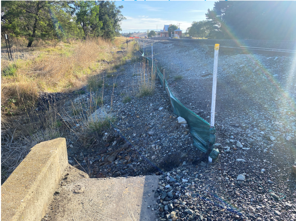
Photo 10: Upgradient of southernmost culvert showing rock armour within drainage line and silt fencing used as control measures for sediment control.
