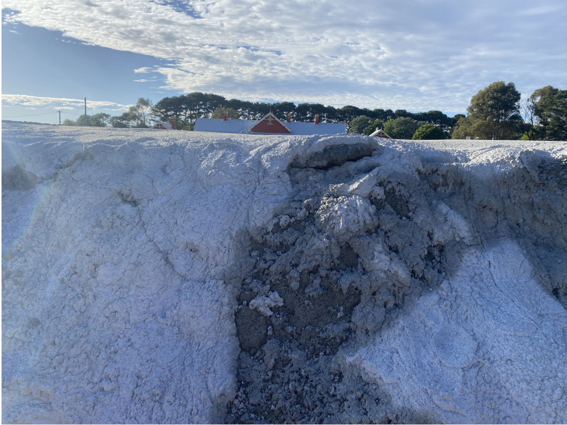
Photo 14: Minor hairline cracking on stabilised sand applied to the stockpile for capping running left to right on photo. Approximately 1-2mm x 3m.
