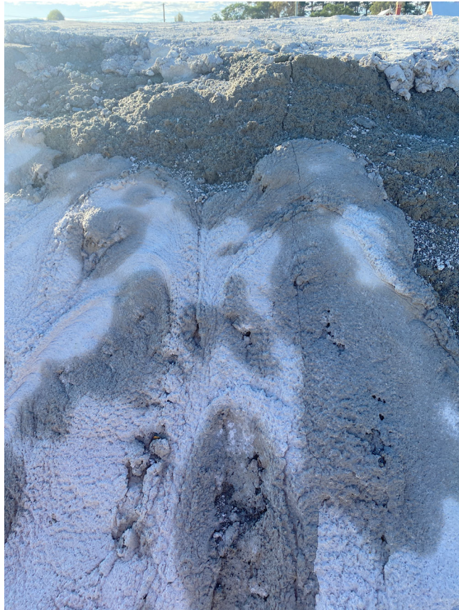
Photo 15: Minor hairline cracking in stabilised sand applied to the stockpile for capping. Approximately 1-2mm x 2m in size. Stable and not expected to allow for water infiltration.
