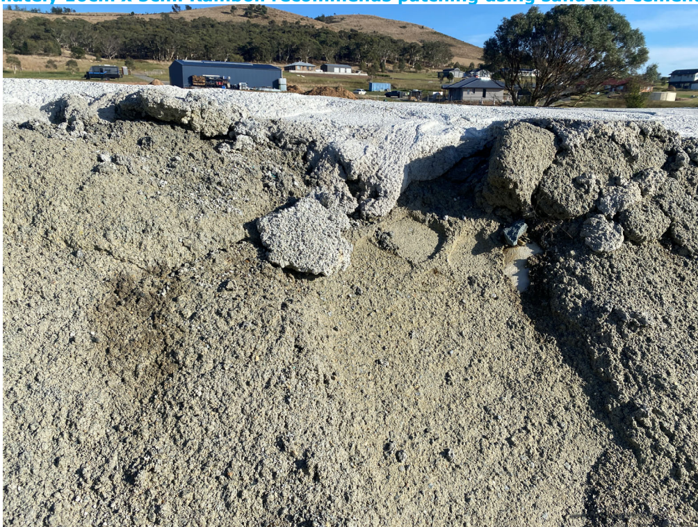
Photo 18: Stockpile marker layer exposure in capping (middle right in photo). Approximately 2cm x 3cm. Ramboll recommends patching using sand and cement mixture.
