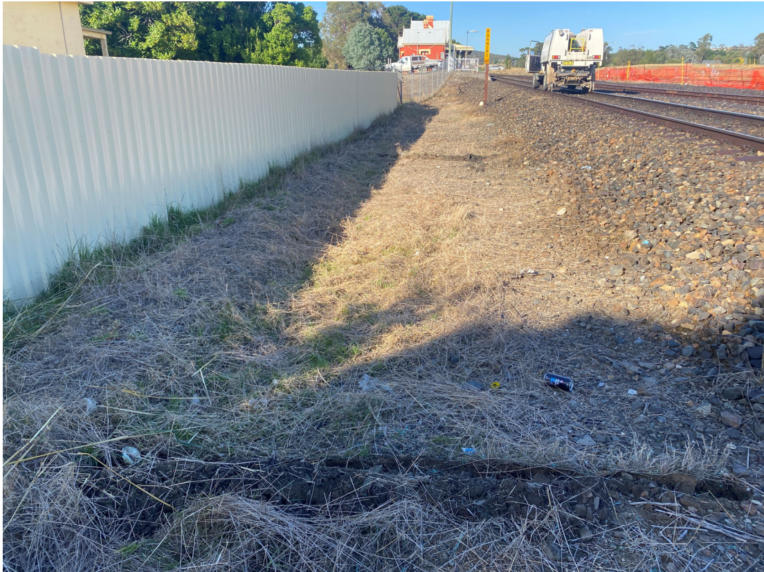
Photo 19: UGL on site. Removed damaged redundant silt fencing adjacent to the boundary of the Station Masters Cottage as per recommendations from Inspection Checklist dated 15-Mar-23.
