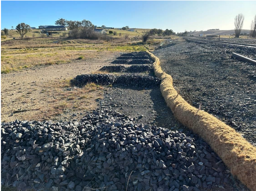
Photo 12: Rock checks running alongside former Woodlawn siding towards the middle culvert. Previous silt fencing with major damage replaced by Coir sediment control logs as recommended in previous inspections. No evidence of sediment build-up in rock armoury.
