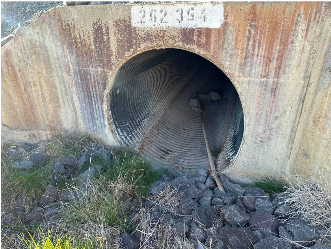
Photo 13: Middle culvert showing no flowing or pooled water. No evidence of sediment build-up in culvert.
