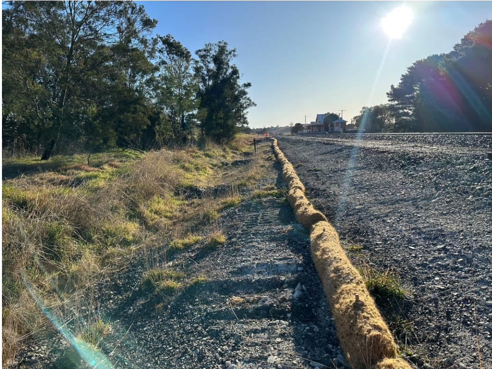
Photo 10: Upgradient of southernmost culvert showing previous silt fencing replaced by Coir sediment control logs, used as control measures for sediment control. Facing north.
