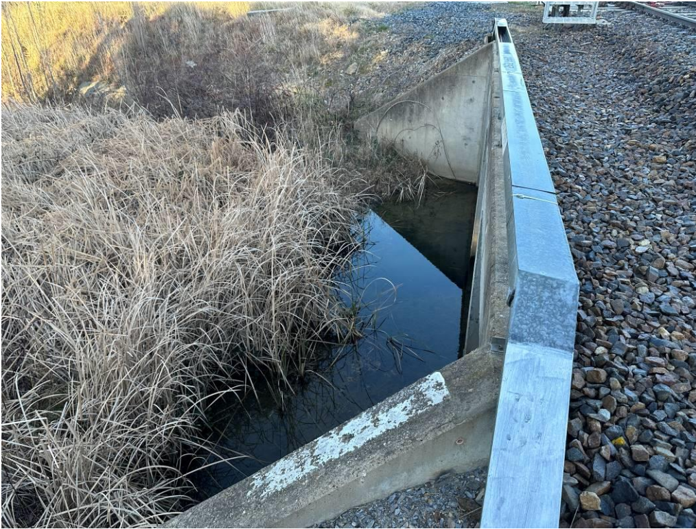
Photo 3: Southern most culvert downgradient of rail line, showing evidence of surface water run off on site. Water is clear, no turbidity, with no observable sediment, long grass and some algae present.
