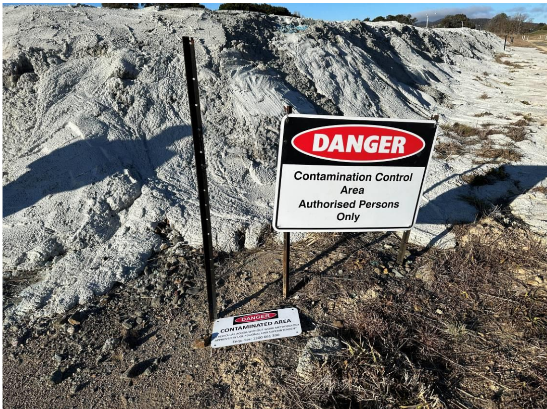
Photo 18: Damaged exclusion zone signage. UGL staff assisting on site reported it was fixed on the same day as site visit (19/07/2023).
