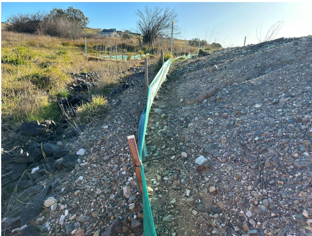
Photo 14: Upgradient of trainline culvert facing north, showing minimal pooling on site near rock checks. Silt fencing appears to have been recently cleared and no sediment was visible.
