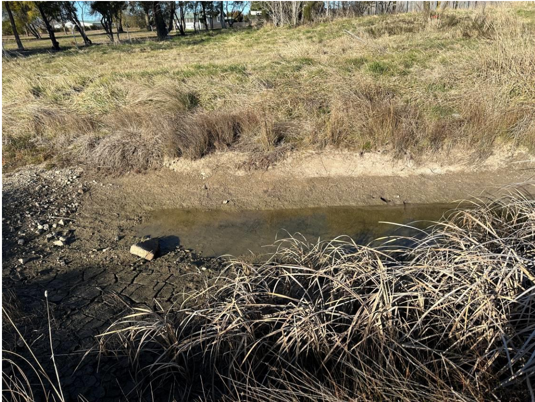
Photo 5: Downgradient of middle culvert. Dry beyond the pooled water and no evidence of current surface water run off on site.
