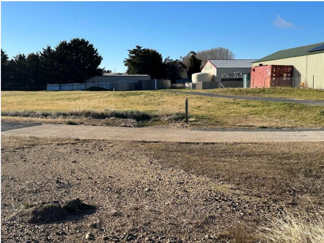
Photo 6: Causeway downgradient of middle culvert showing no evidence of current surface water run off on site. No visible sediment on road or vegetation nearby from sediment water was running off site in between inspections.
