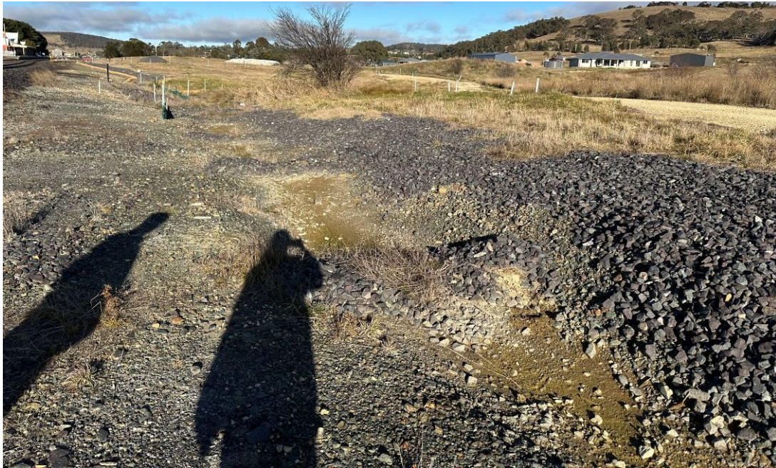
Photo 15: Rock armour upgradient of trainline running from the middle to the north culvert. Some sediment visible on rock armour. Facing South West.
