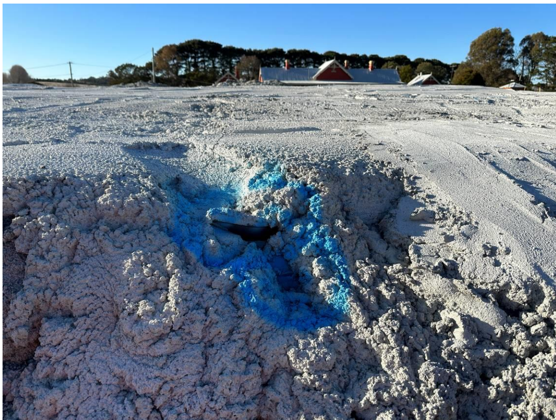
Photo 20. New Geofabric marker layer visible in stockpile capping, on western side, marked with blue paint. Approximately 4cm x 5cm.
