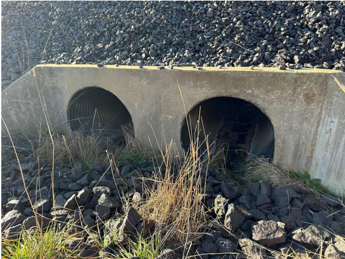
Photo 16: Upgradient of northernmost culvert. No evidence of surface water run off on site. No evidence of sediment buildup on rocks. Rock armour and natural vegetation allow for sediment control in surface water.
