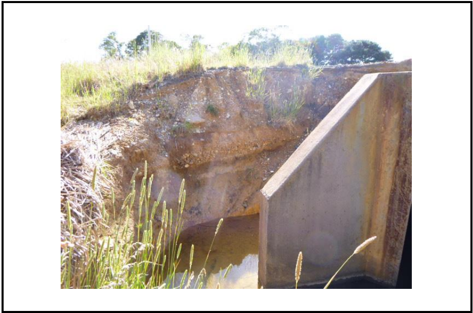
Photo 1: Image of embankment adjacent to monitoring location SW1. Signs of erosion from recent heavy rain events.
