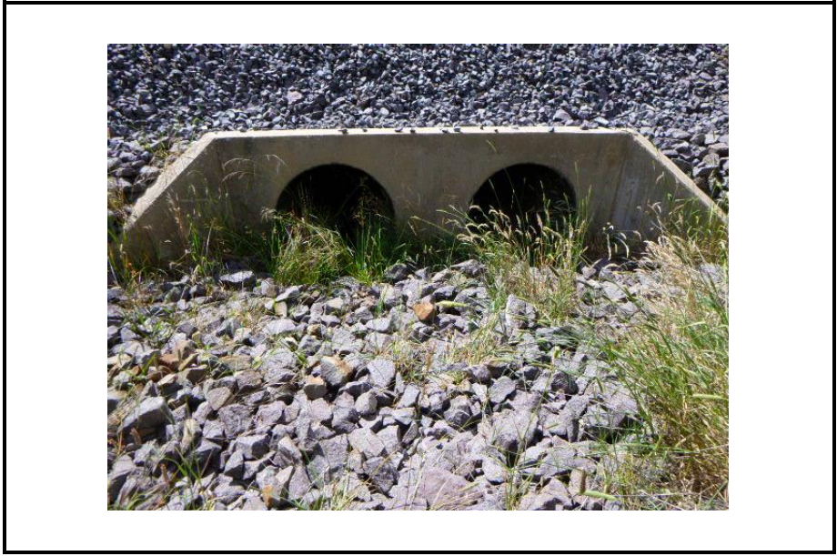
Photo 8: Image of monitoring location SW5. Both culverts and surrounding ballast were dry.
