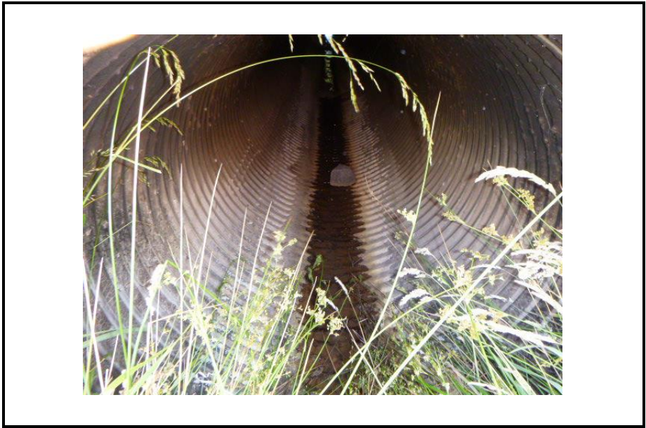
Photo 9: Image of right-side culvert of monitoring location SW5. Image shows staining and sediment build up from times of flowing water.
