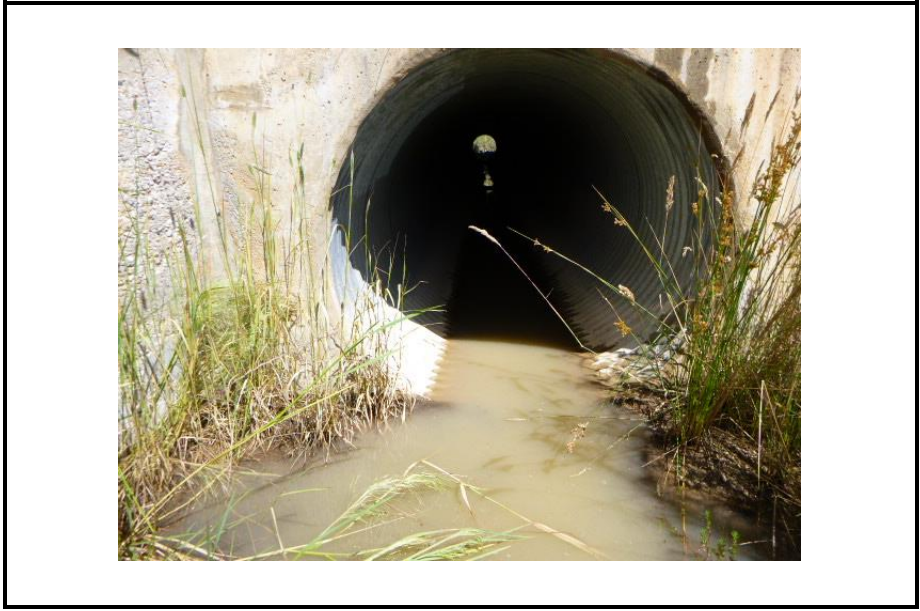
Photo 10: Image of culvert adjacent to monitoring location SW6. Water pools at this location and contains sediment colloids.
