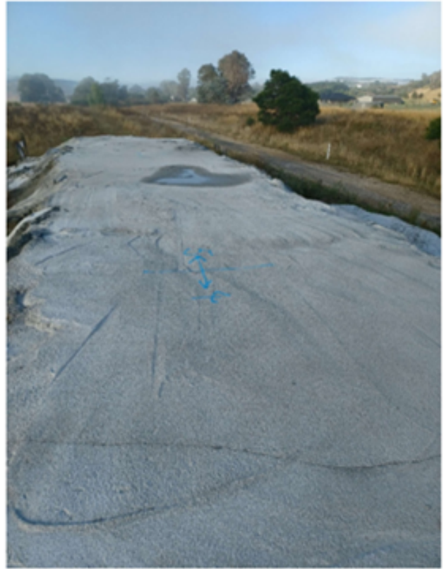
Minor Cracking In Section 4 Of Contaminated Stockpile
