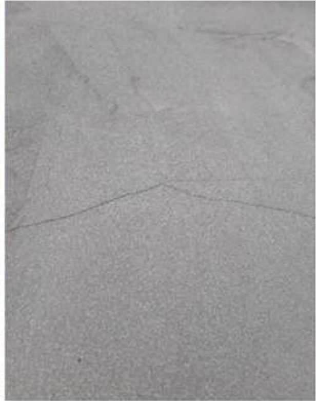
Example of hair line cracks in stockpile capping
