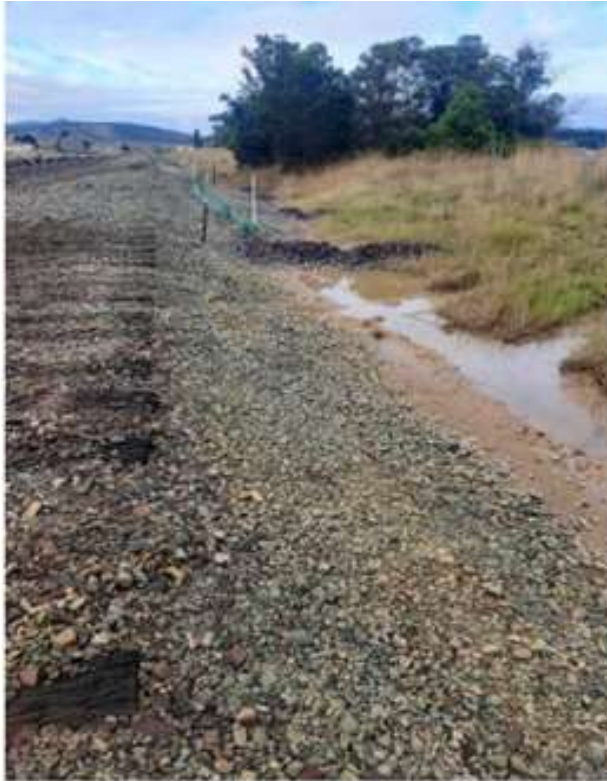
West side cess drain with sediment controls
