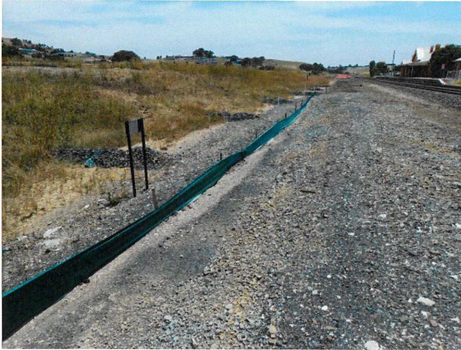
Figure 1: Sediment controls, west of railway line looking North.
