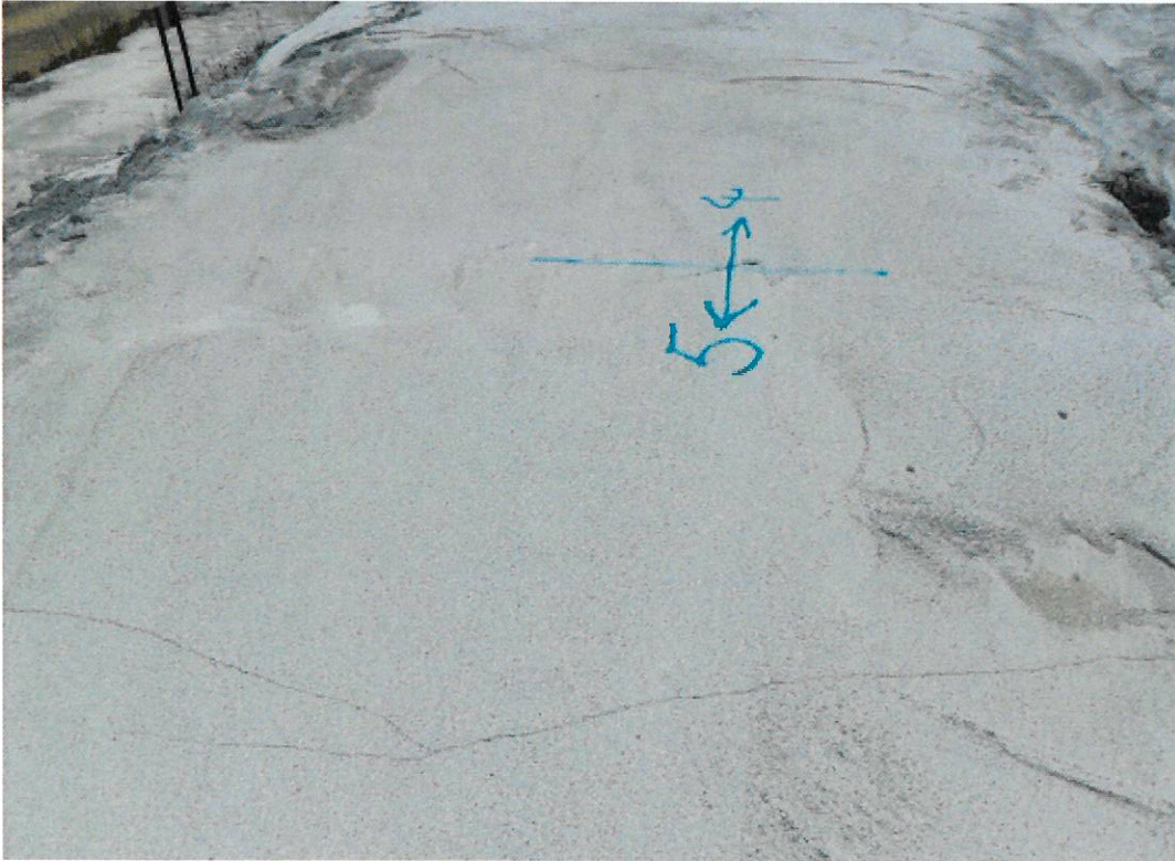
Figure 5: Stockpile Zone 5 – foreground of image gives an example of approximately 1mm cracking in stabilised sand cement cover. Future monitoring will focus on lateral cracking, width, and depth.
