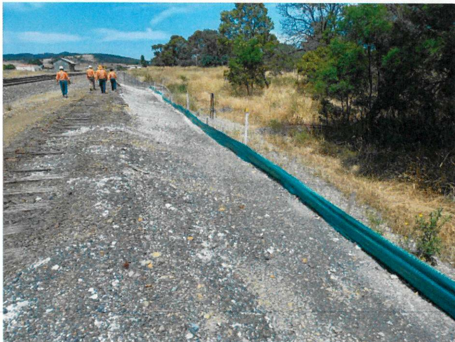
Figure 2: Sediment controls, west of railway line looking South towards Goulburn Street level crossing.
