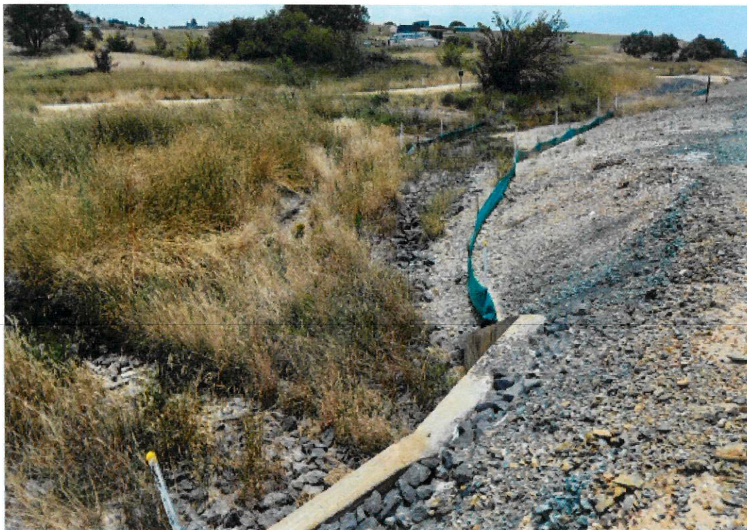
Figure 8: Sediment fences protecting site drainage, installed west of the railway line looking north (approximately opposite Boyd Street)
