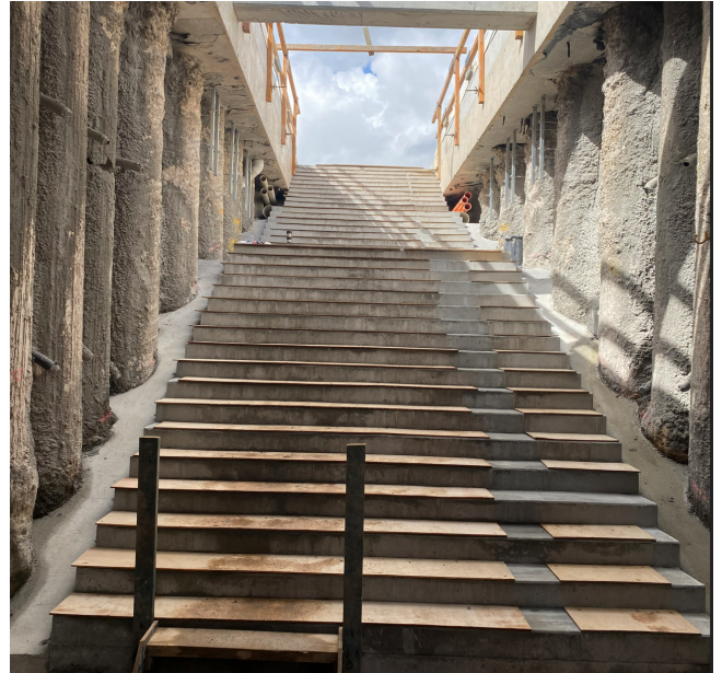
Above: New staircase under construction from underpass level to the island platform, April 2023.
