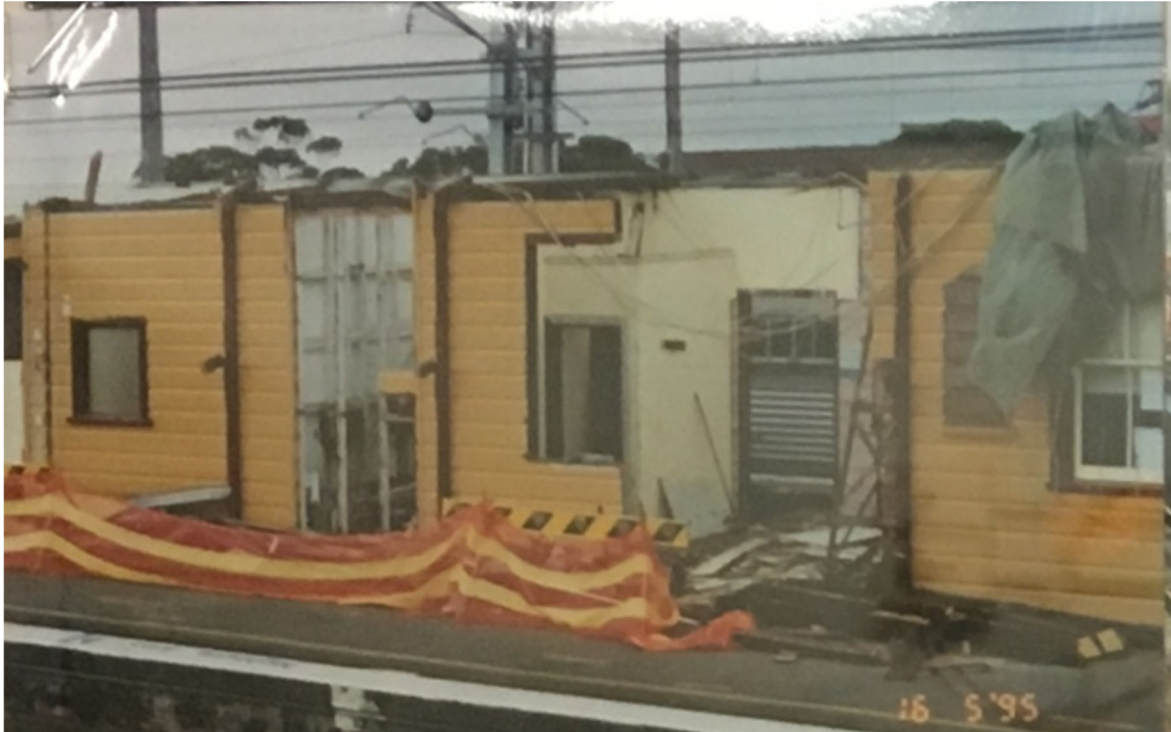
Plate 44 1995 replacement of the Waterfall Railway Station platform building (Source: Waterfall Railway Station – Station Masters Office Display, 2019)
