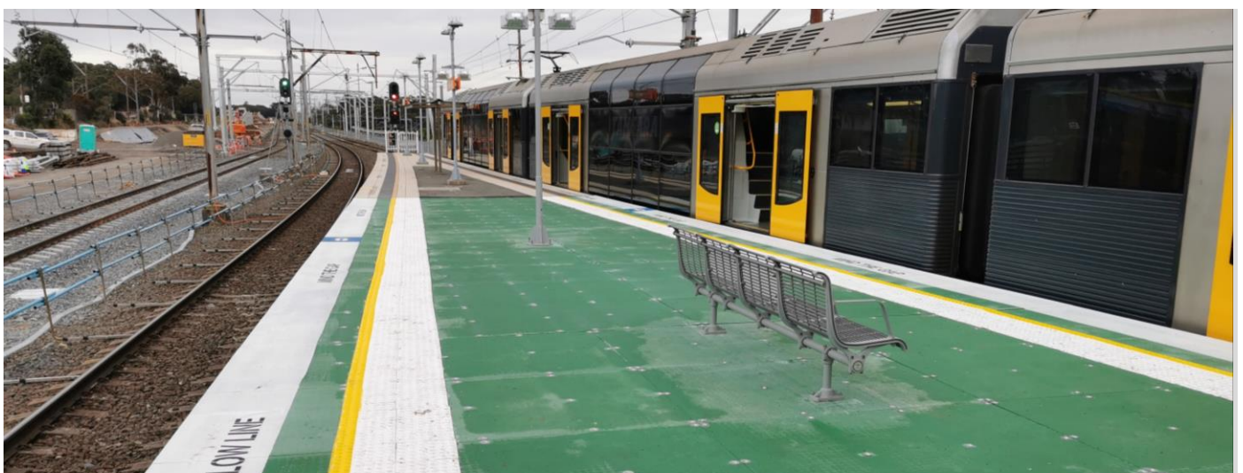
Photo of modular temporary platform (green) enabling simple and fast removal and reinstallation to facilitate upcoming work.
