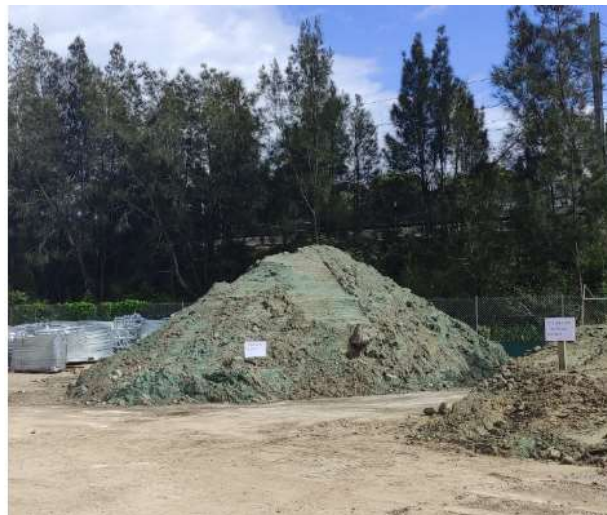
Image of stockpiles stabilised with polymer on a More Trains, More Services site
