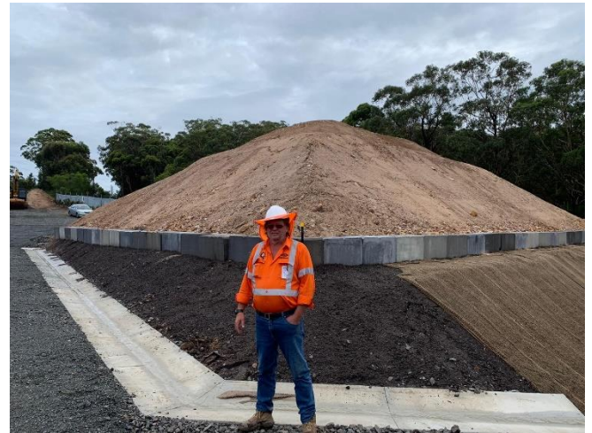
Waterfall Superintendent, 'Bullet' (Chris) on-site in front of crushed sandstone we are storing for re-purposing for Sydney Trains who will use the material to repair local access roads
