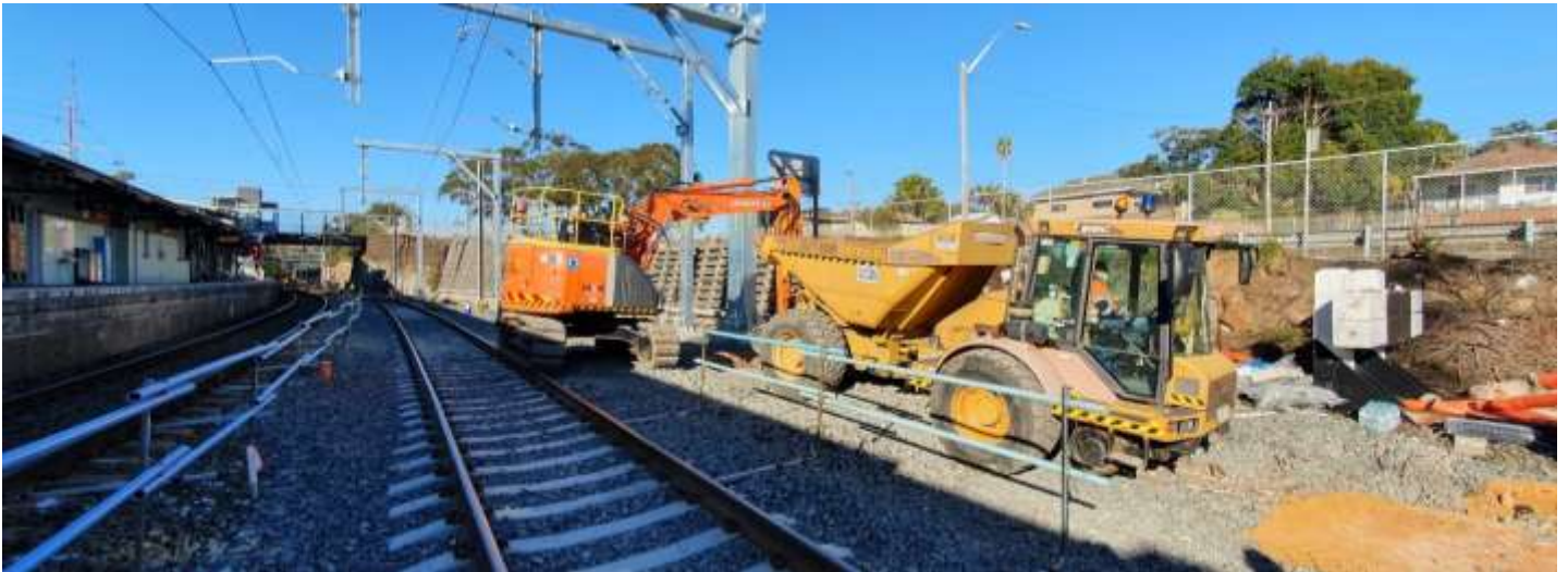
Photo taken of construction work inside the rail corridor at Waterfall – August 2021
