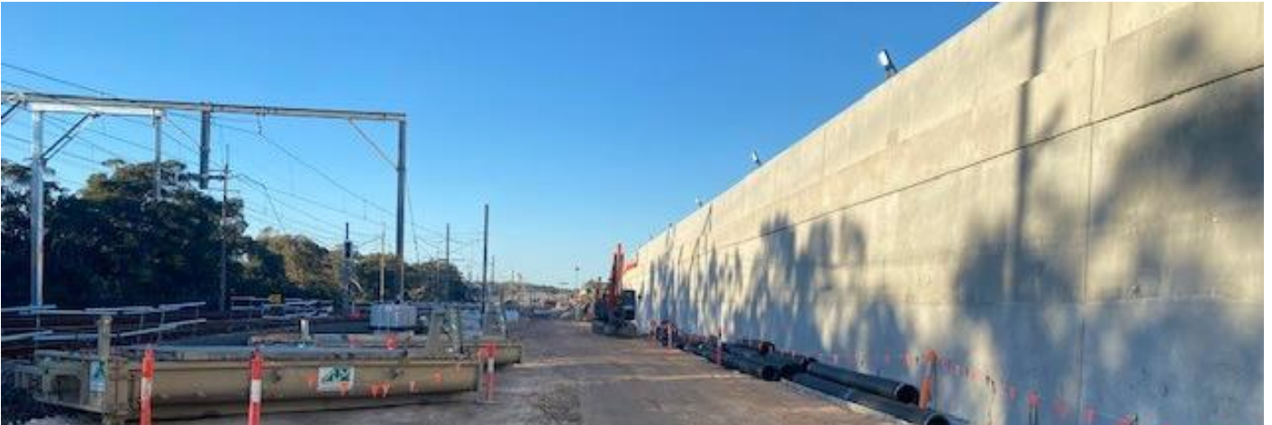
Photo taken inside the rail corridor - August 2021, showing the new retaining wall off the Princes Highway
