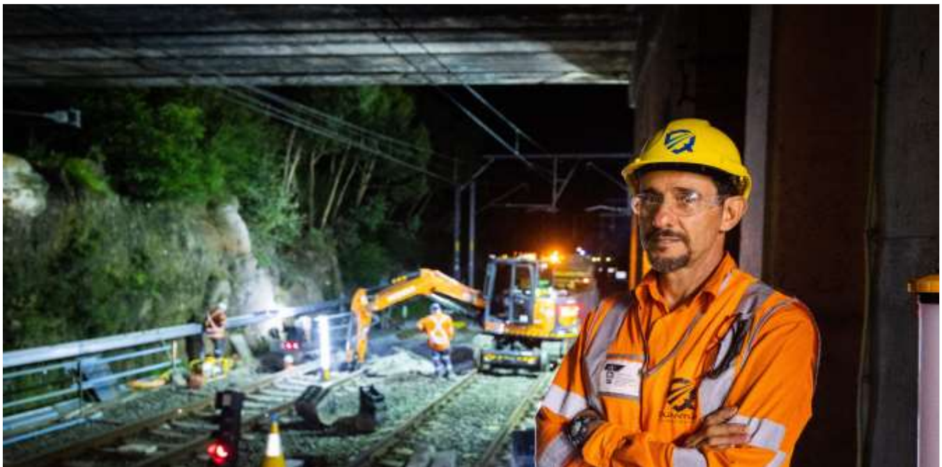
Construction work being undertaken as part of More Trains, More Services on the South Coast in 2021
