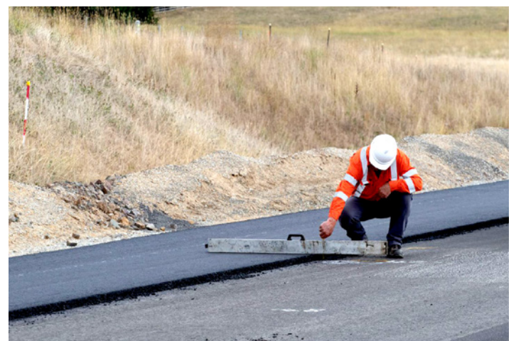
The paver is followed by a crew constantly checking levels, temperature and depth of the AC.
