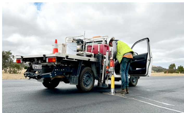
A coring machine drills out an AC sample from the first layer of the new road surface which is then sent off for density testing.
