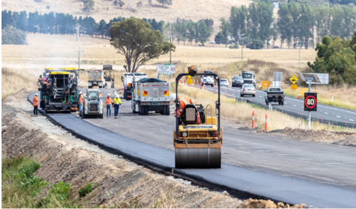
Trucks, a Material Transfer Vehicle, paver, steel drum rollers and the paving crew perform a well-orchestrated program carrying out AC work.
