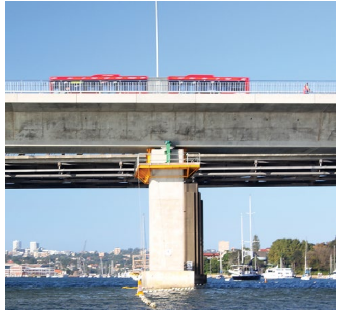
Even using high quality concrete and steel shuttering, concrete quality can be affected by admixtures from oil and curing compounds, as in this example of staining on the girder of the new Iron Cove Bridge.
