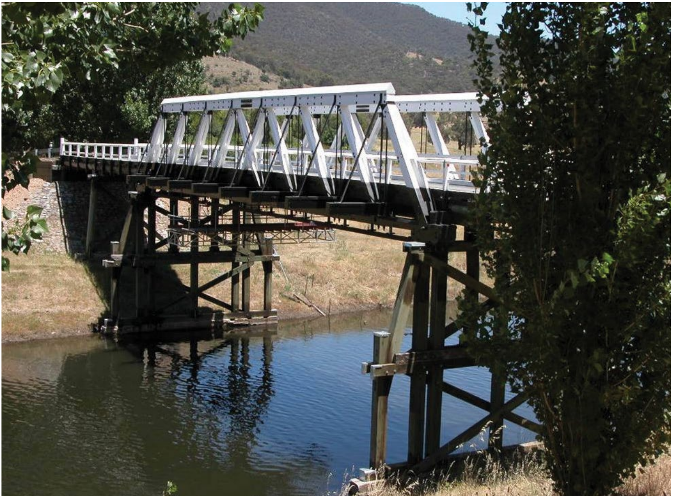
The Wee Jasper Bridge, refurbished in 2006, has a two-tone (black and white) colour scheme which is widely used in the ACT.
