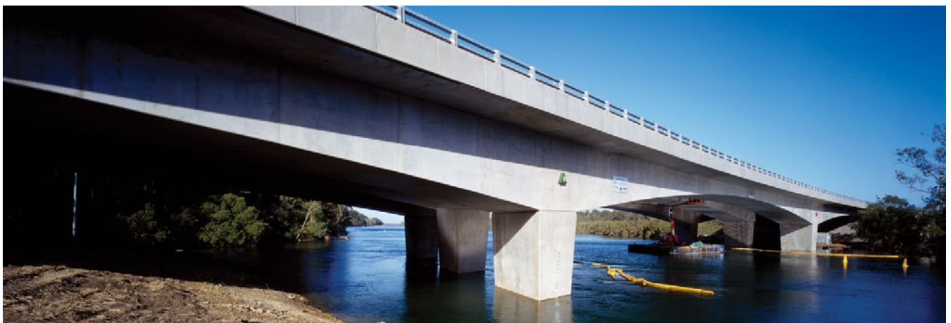
The Pacific Highway bridges over the Brunswick River at Brunswick Heads shows the application of the Cardiff University guideline.
