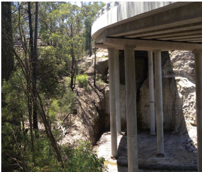
The pier widths used on this bridge next to the old wool road on Main Road 92 near Nerriga appear too thin and almost spindly in comparison to the depth of the girder and parapet.
