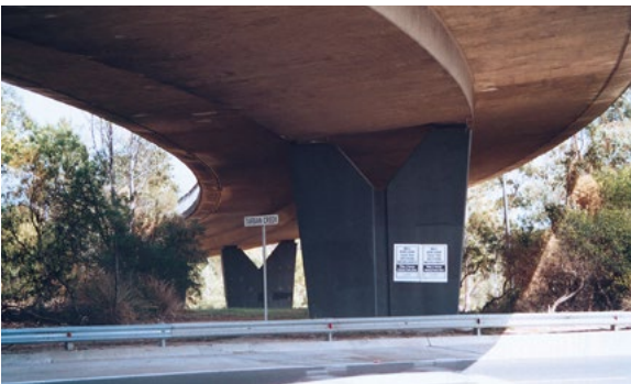
Deep overhang and acute angle of deck on this bridge on Victoria Road at Huntley's Point.
