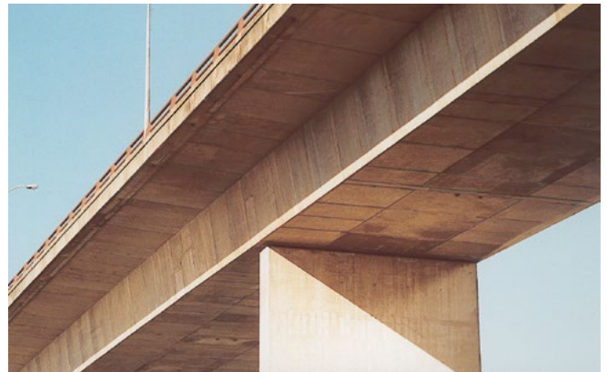
The bridge over the Hunter River at Stockton demonstrates that a generous deck overhang is important to consider as part of the bridge cross section.
