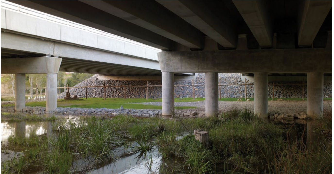
Where there is room, the space under the bridge can be used to create fauna corridors and help reconnect habitats. Bonville Bypass included many fauna connections, such as this example along the Bonville creek.
