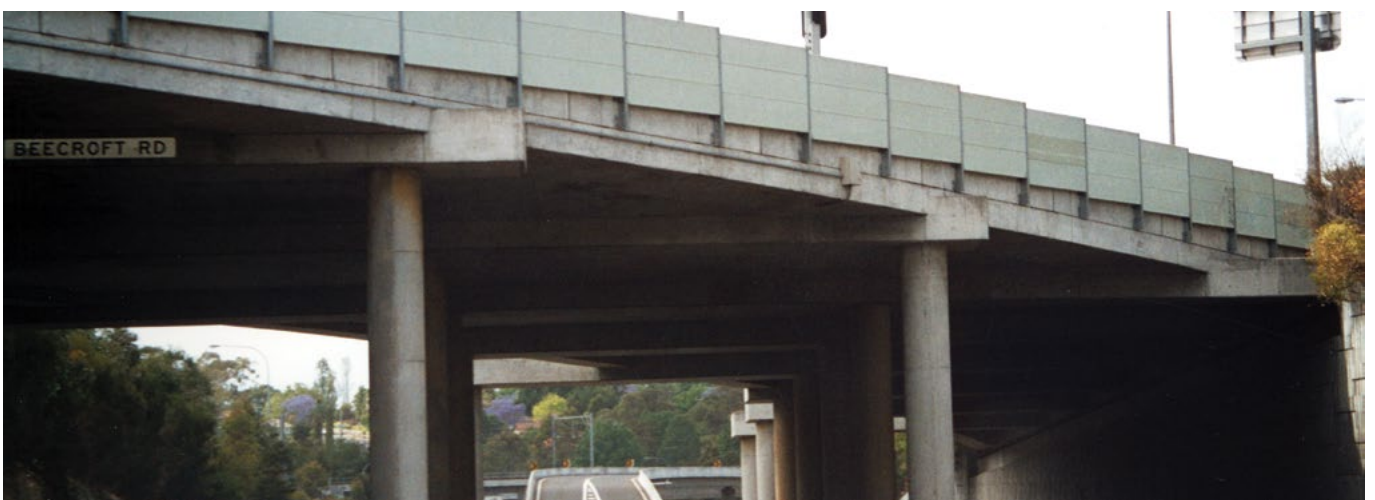
The lack of a well designed parapet creates a visually confusing superstructure as in this bridge over the M2 Motorway at Beecroft. This is an example of a poor aesthetic outcome.
