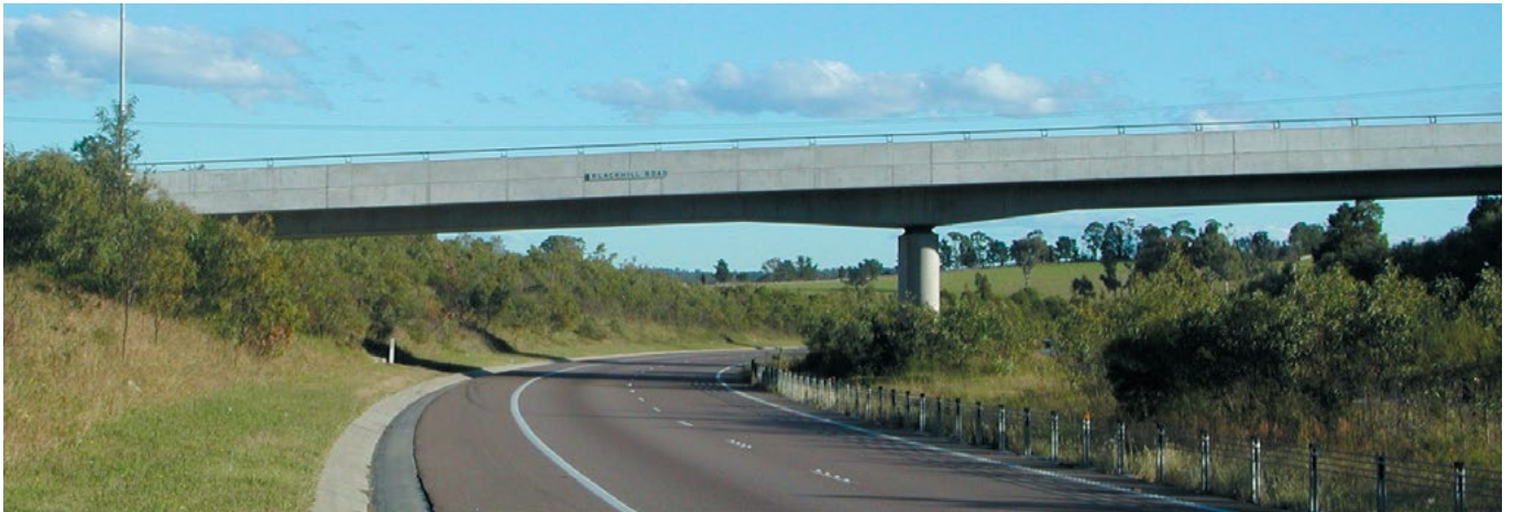
On the girder on the bridge over the F3 Freeway at Blackhill Road near Newcastle, the haunching is made less elegant by the angle of transition between haunched section and horizontal beam. (Also note how the solid parapet affects bridge slenderness).
