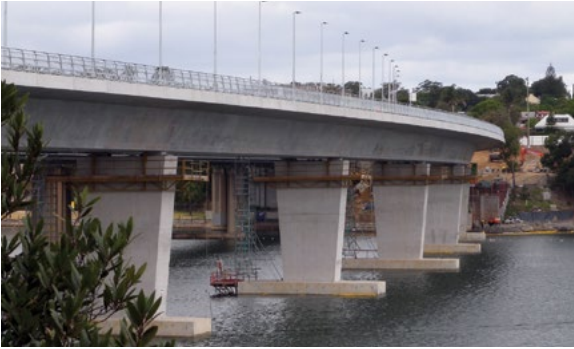
An angled girder can maximise shadow time on the girder and accentuate the parapet edge.
