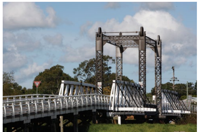
Hinton Bridge over the Paterson River near Maitland is one of the oldest Allan truss bridges in Australia built in 1901 with a lift span. Due to the deterioration of the bridge's trusses and lift span and the need to increase load carrying capacity, rehabilitation and strengthening works were undertaken in 2005. The bridge is an example of carrying out repair sensitively by using timber, steel and concrete composites so as to preserve its heritage character.
