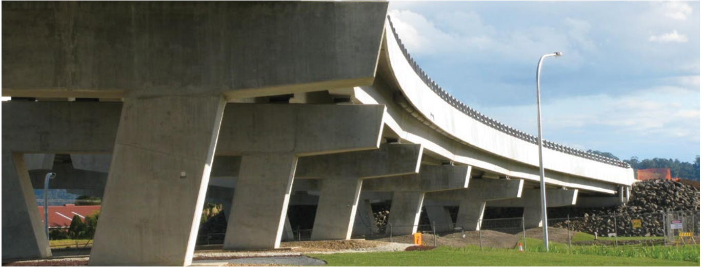
On land, as in this example on the Pacific Highway at Ballina, it is generally visually preferable to bury the pile caps below ground level. Note the curved parapet over the straight facet of the Super T girder.
