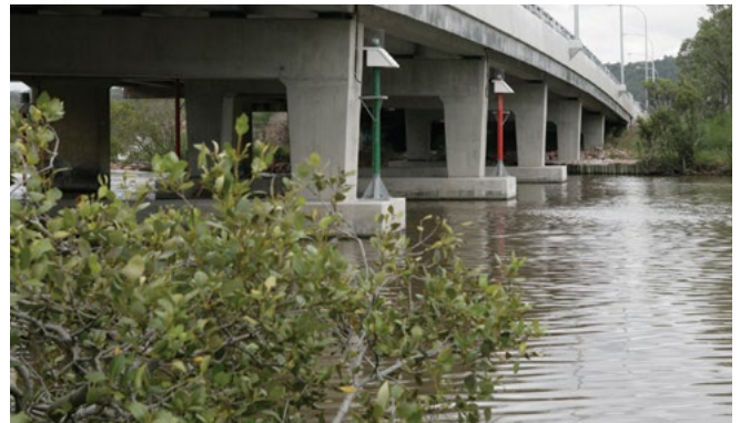
A concrete frame creates a simple attractive pier as used on the Herb Feint Bridge in Adelong and the Five Islands upgrade at Lake Macquarie.
