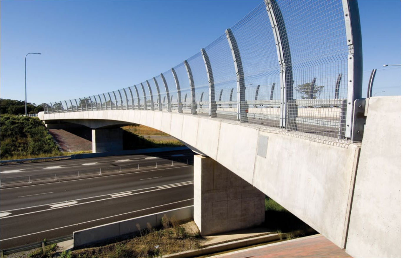
On this bridge over the Pacific Highway at Nabitac the bridge barrier piers and safety screen posts are aligned and integrated. The bridge parapet is expressed and not obscured. The shaped form of the barrier is considered as part of the whole structural design of the bridge to create a beautiful aesthetic outcome.
