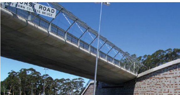
A curved soffit with a rounded edge can make even deep girders appear very slender because the curved section only catches the light in a thin line at any time of day. These girders can create very elegant and attractive bridges, such as this bridge over the great Western Highway at Shell Corner.
