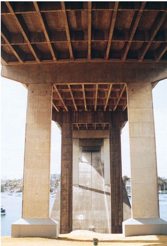
The pile caps on the Gladesville Bridge are also in keeping with the large piers and provide a suitable structural termination in the park. An alternative approach, generally preferable, would have been to bury the pile cap, but in this example the outcome is well considered.
