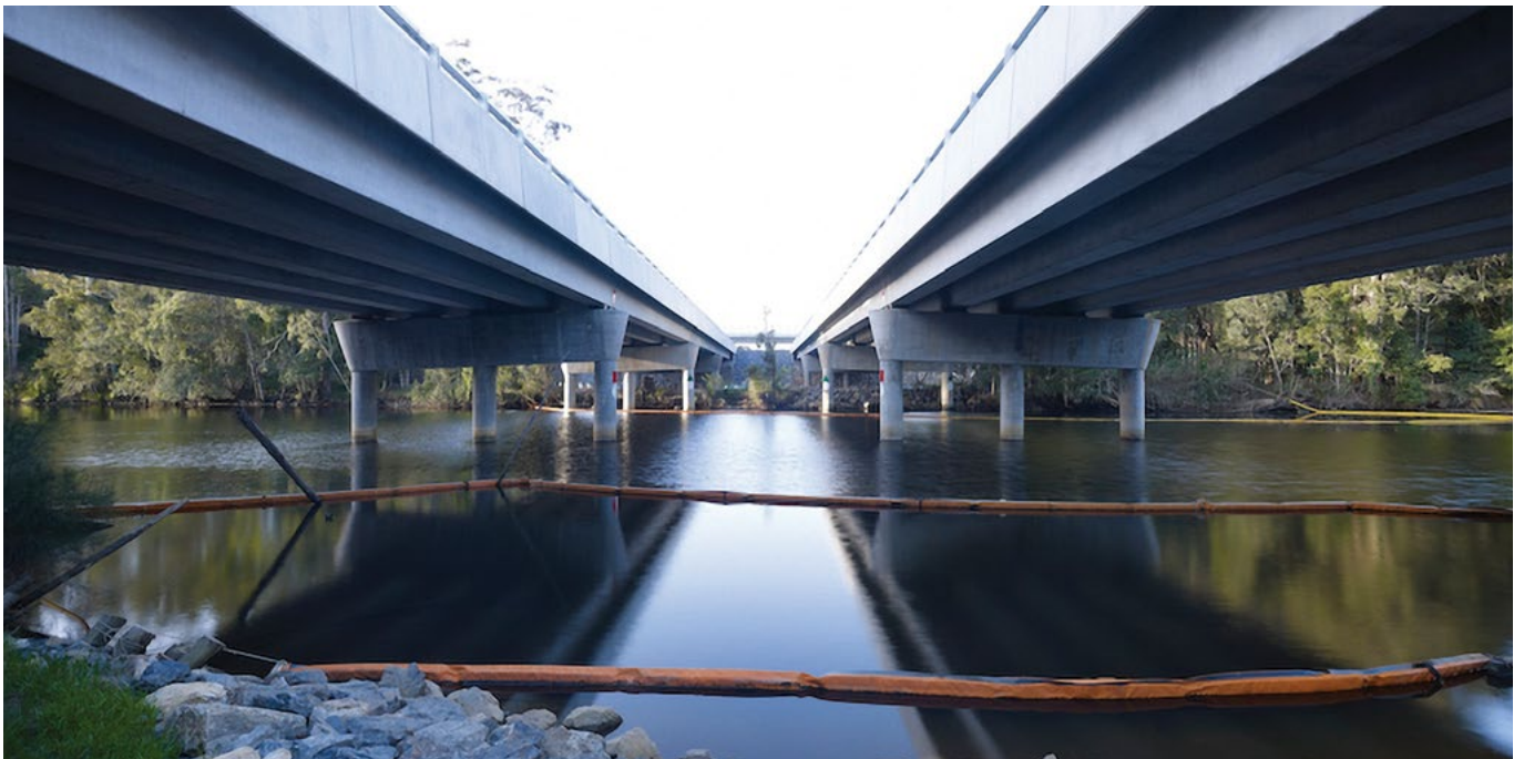
These Pacific Highway twin bridges at Bonville have a perfectly symmetrical composition.
