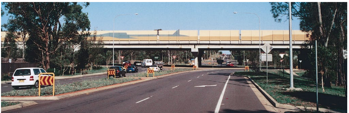
This bridge carrying the Pacific Highway at Raymond Terrace has a visual slenderness ratio of only 1:6 (taking into account the noise wall). Its chunky appearance is contributed to by the use of headstocks. Transparent noise walls would have resulted in a more slender appearance.
