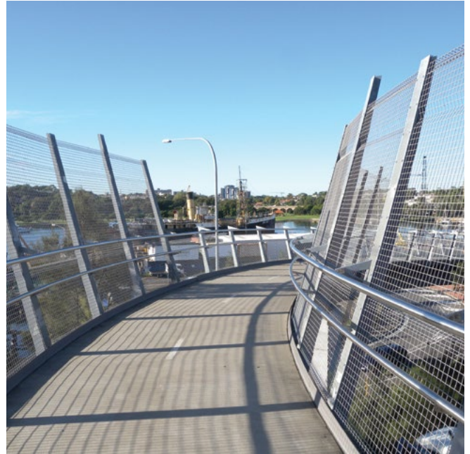
The absence of a cage creates a more open welcoming space as in this example on the Beatrice Bush Bridge, Rozelle.
