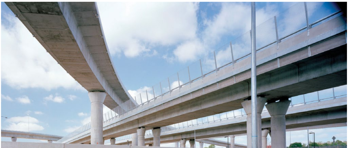
The circular piers and mushroom-type capitals form pivots that accommodate the multi-directional ramps on the M7 Motorway.
