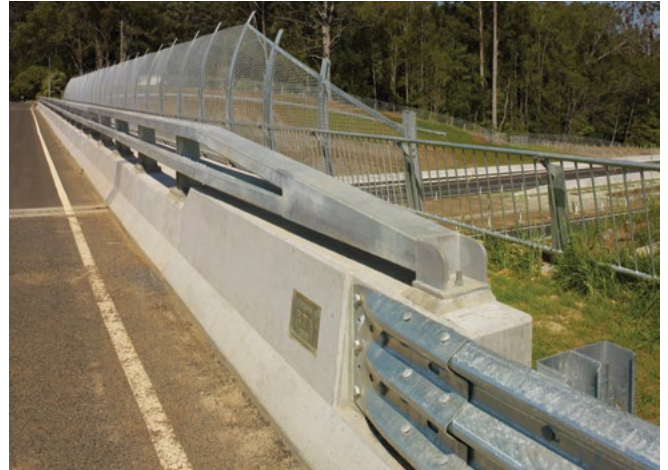
Tapering the barrier and parapet is a neat way of ending the bridge barrier.
