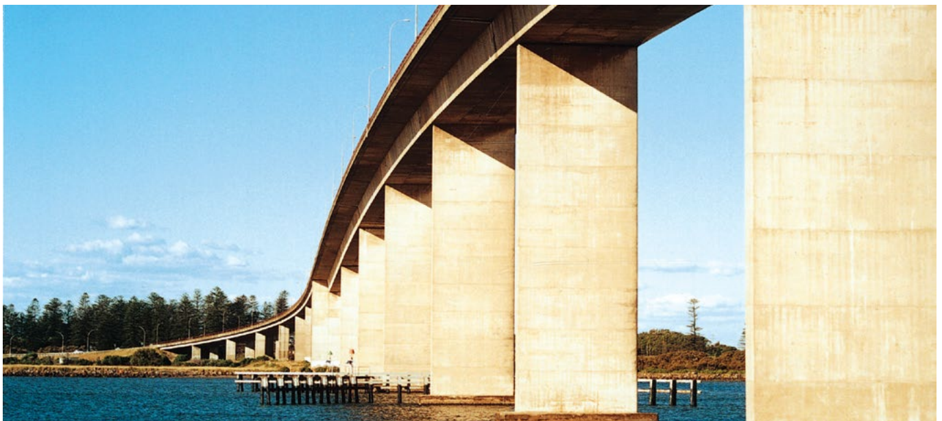
Bridge over the Hunter River at Stockton shows the effect of a right angled girder shape in afternoon sunlight.
