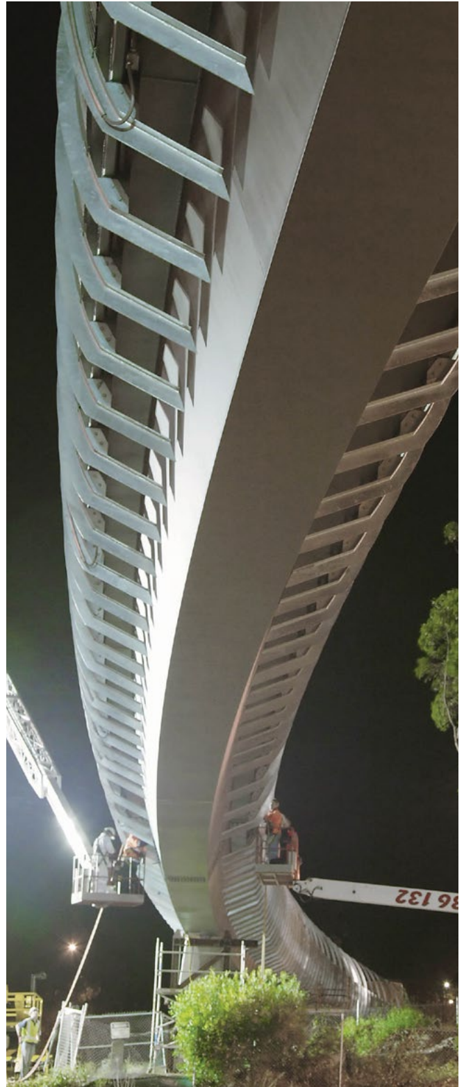
Falcon Street pedestrian bridge under construction. A slender, steel box girder spans 220m over the Warringah Freeway.
