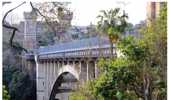
Suspension Bridge, Northbridge: Inside and outside views of the retrofitted safety screen. This is a new expressive form which complements the character of the old bridge.
