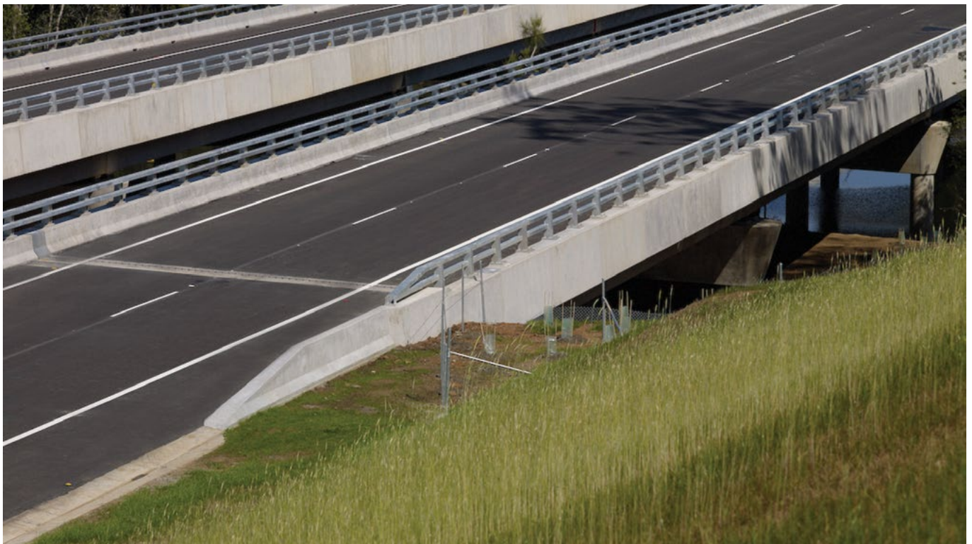
Neat tapered terminations to the bridge barriers on the Pacific Highway at Bonville
