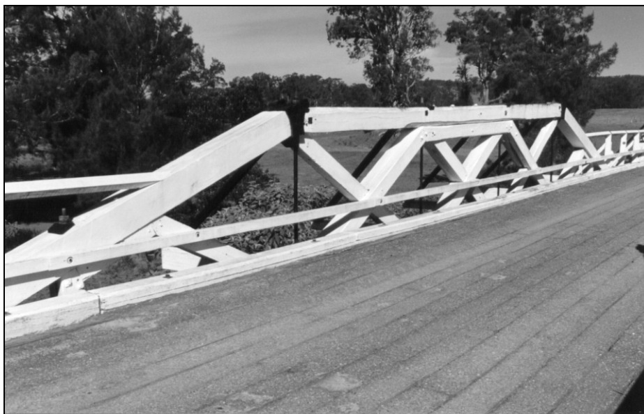
Figure I.3.2e – Typical interior view of an Old PWD Truss with an inner truss at mid-span.
