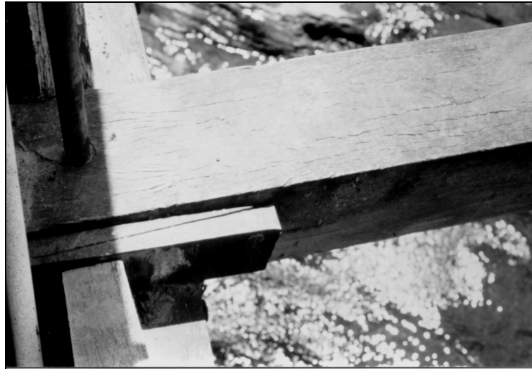
Figure I.3.3f – Steel fox wedges were used to counter shrinkage effects and provided a simple means for regular adjustments.
