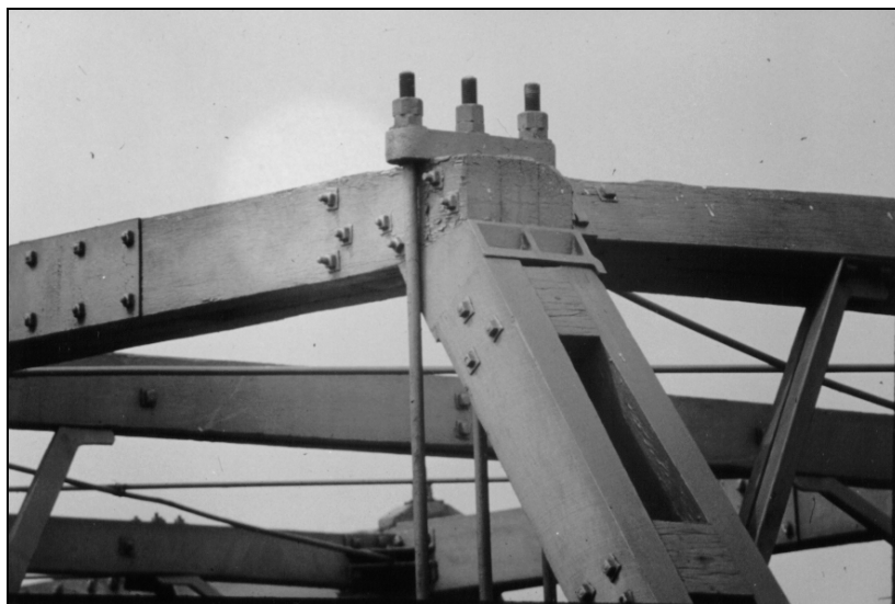
Figure 1.3.4d – The simple truss shape allows tightening via the nuts on the top chord to combat shrinkage effects. One, two, or even three vertical rods were possible due to the separated members. The cast iron shoes allowed good transfer of forces at truss joints.
