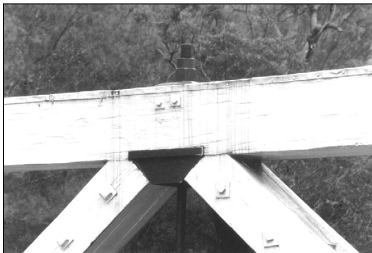
Figure 1.3.3e – Connection of diagonals to top chord via cast iron plates provided a superior transfer of force.
