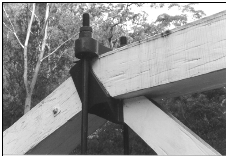
Figure I.3.3d – Vertical rods placed outside the truss faces eliminated the need to drill through the top chord.
