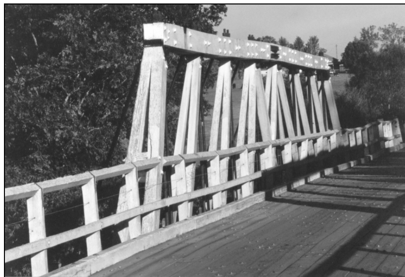
Figure I.3.4c – Parallel pairs of members held apart by timber spacers were used to improve load characteristics, aid painting and prevent the collection of water.
