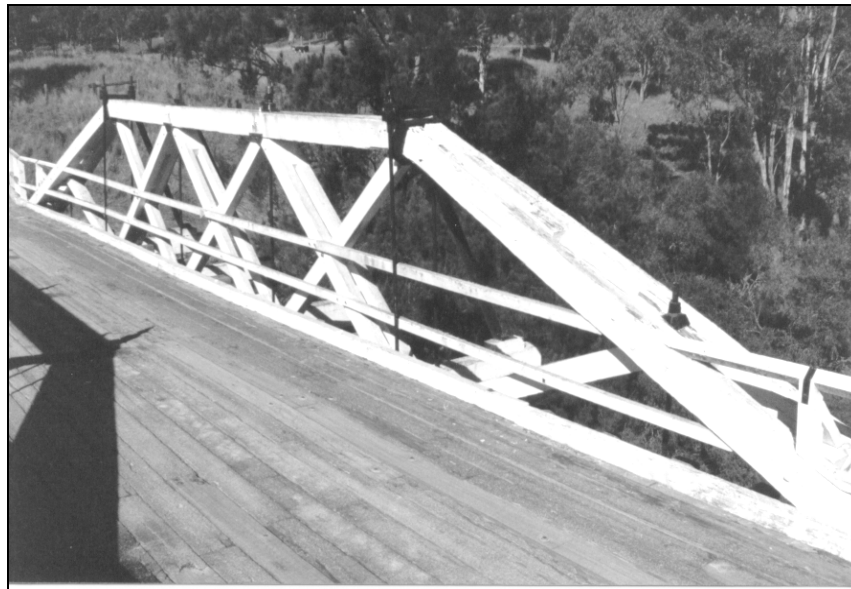
Figure 1.3.3b – The single thickness top chord was part of McDonald's improvement to the OLD PWD trusses.
