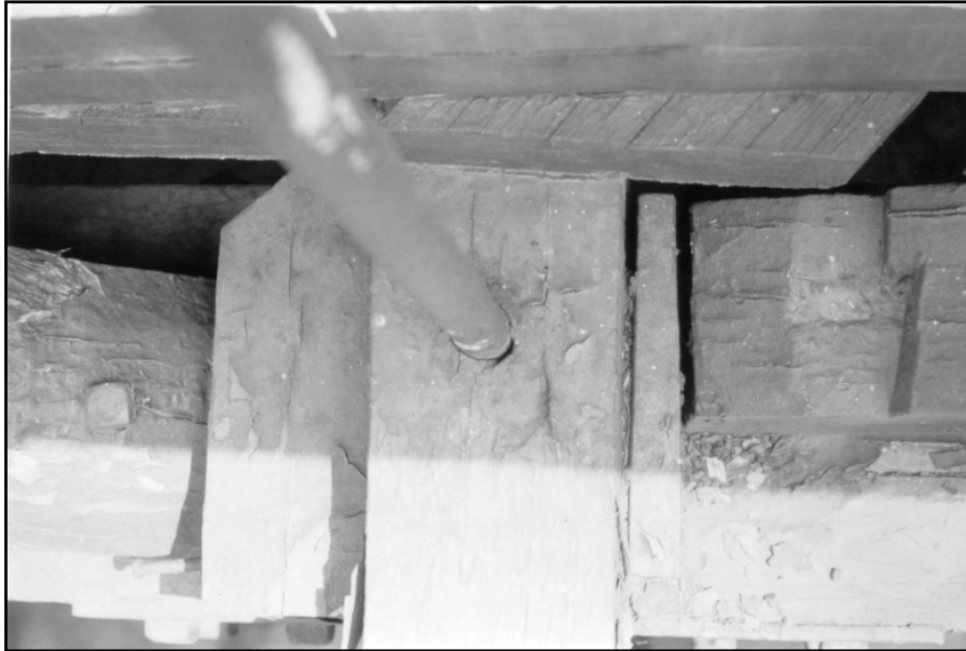
Figure 1.3.2h – Packing at bottom chord was used to help counter the effects of shrinkage.
