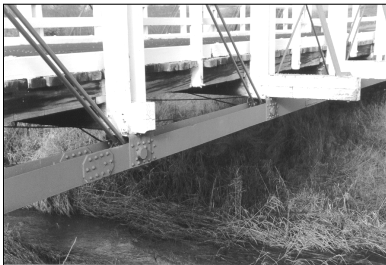
Figure 1.3.5e – Pins along the bottom chord facilitated speedier construction but later lost favour due to the difficulties experienced in maintenance and strengthening works.
