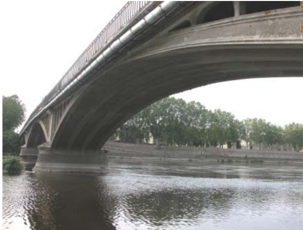
Pont Camille de Hogues (Pont de Châtelleraut) 1899-1900 First notable reinforced concrete bridge.
