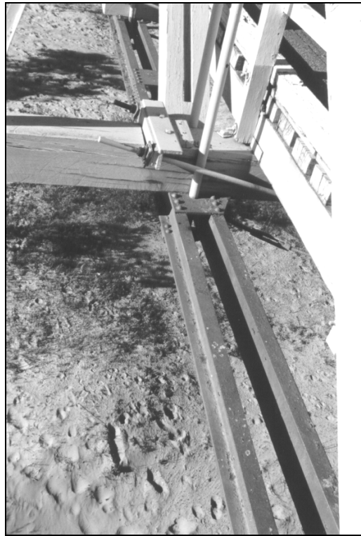
Figure 1.3.6b – The pair of steel channels that made up the bottom chord utilised the tension characteristics of steel along with the compression characteristics of the timber.
