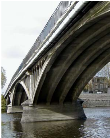
Pont Camille de Hogues (Pont de Châtelleraut) 1900 First Heritage ranked reinforced concrete bridge. (source www.structurae.de )
