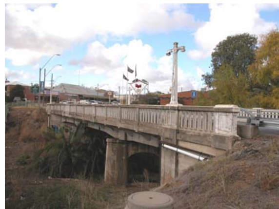
Burrangong Creek Bridge, Young (RTA Bridge No 6427). Shopping precinct in background and Information Centre on right
