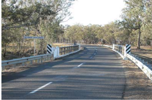
Mulyandry Creek Cowra ( Bridge No 4282) Note curved deck with crossfall to suit
