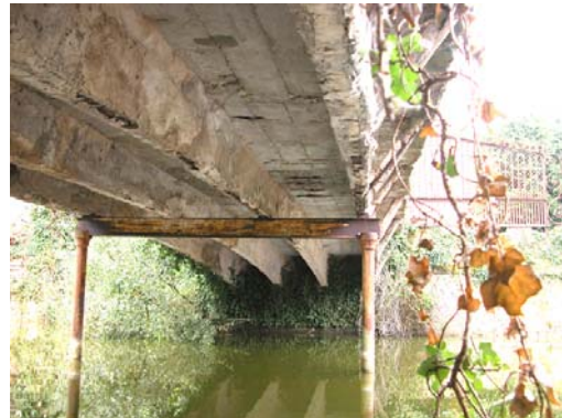
Underside of bridge showing four curved beams and retrofitted central prop to allow tractors to cross the bridge
