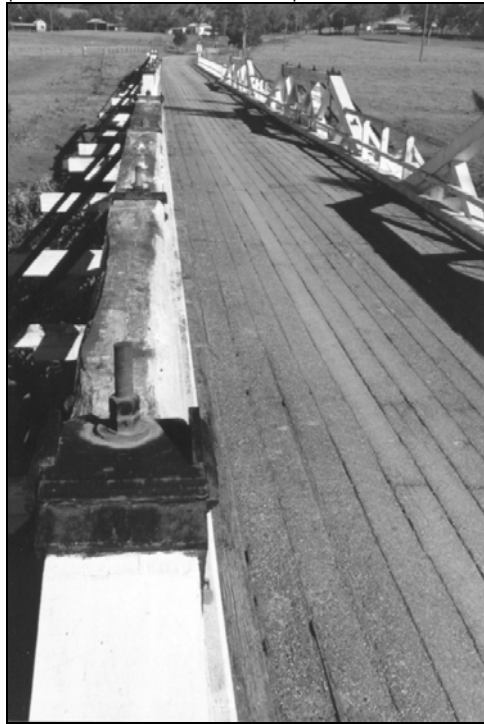
Figure 1.3.2f – View of truss showing single rods all of which are the same size
