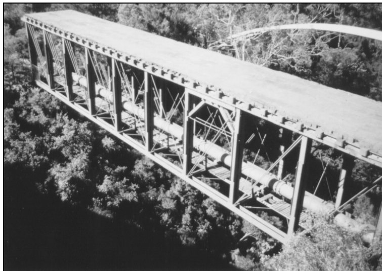
Figure 1.3.5d – The 1901 DeBurgh Bridge over Lane Cove River. DeBurgh's greatest achievement with a 165ft (50.3m) deck span was damaged in the 1994 bush fires.
