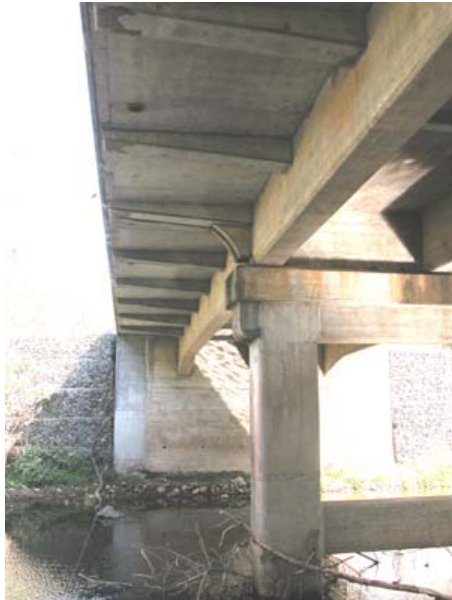
Broughton Creek Bridge (RTA Bridge No 704) Widened two span bridge composite with abutment
