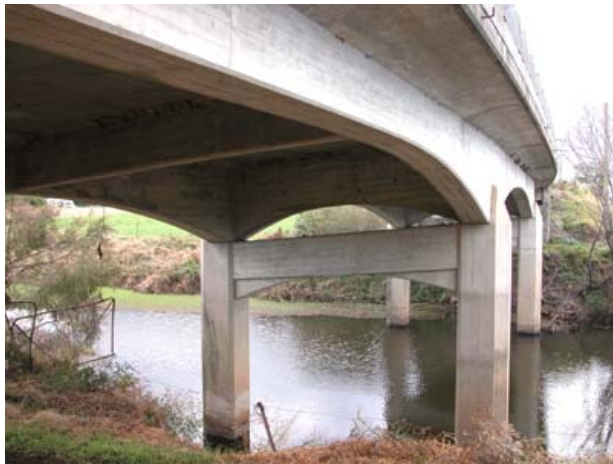
Croobyar Creek Bridge ( Bridge No 730) Note curved deck with crossfall to suit high speed curve
