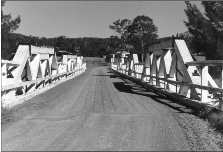
Figure I.3.2d - Deck view of the Monkerai Bridge over the Karuah River which has large timber sections typical of the Old PWD design
