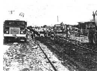
The ready mixed concrete is tipped onto the subgrade and spread by hand ahead of the spreader-finisher (right).
