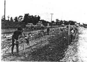
Steel formwork rails are accurately positioned for the spreading of the mass concrete base.
