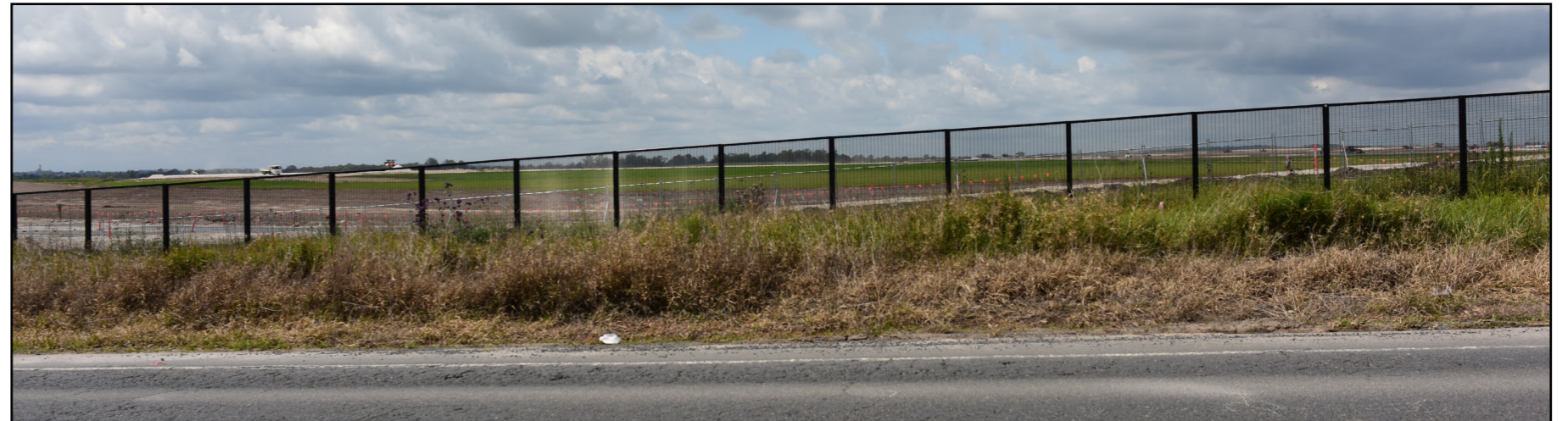
Figure 31: The LCZ comprises a large, open construction site which is fenced around the perimeter
