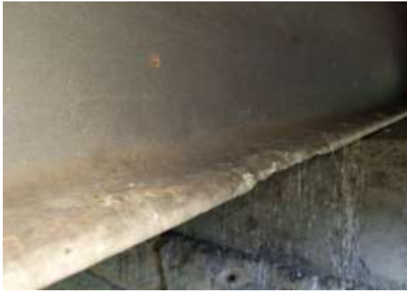
Photo 3-1: Example of section loss on edge of flange
