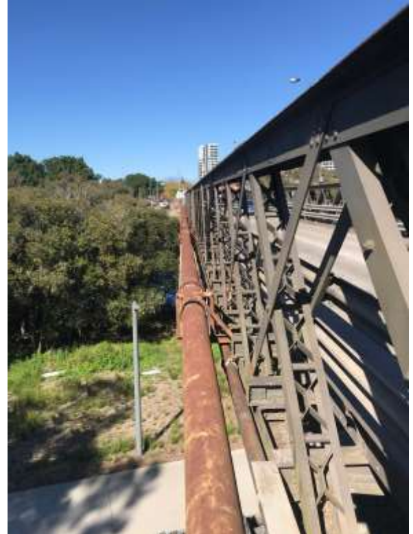
Photo 3-4: Water main facing south (smaller pipe)
