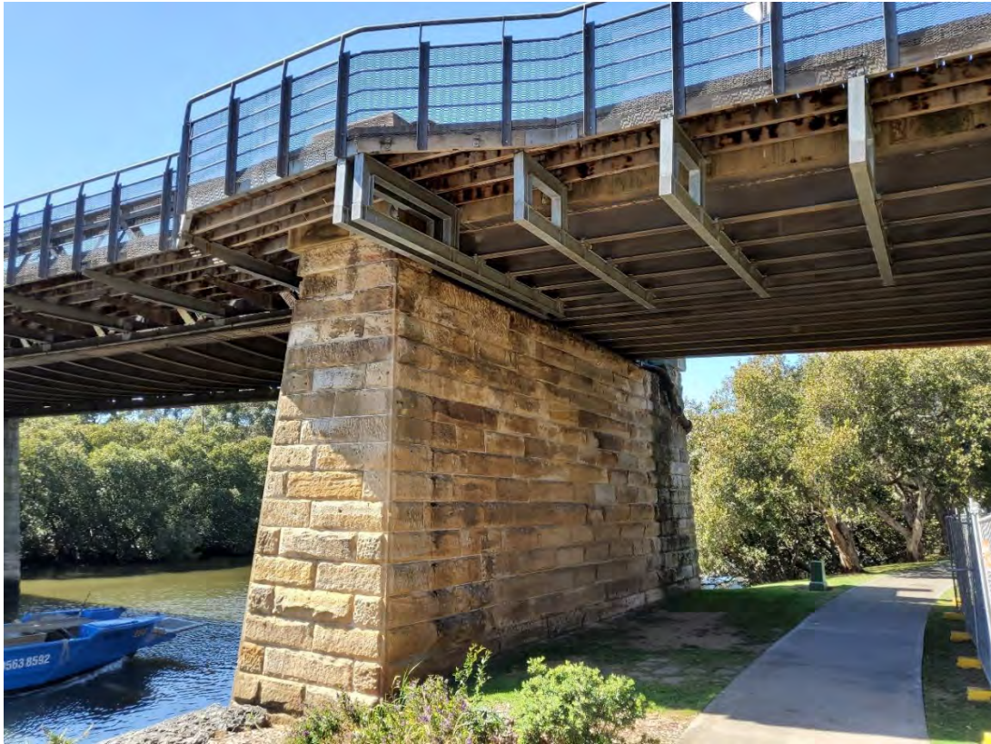
Figure 5.18 East facing view showing pier at the southern end of the bridge.
