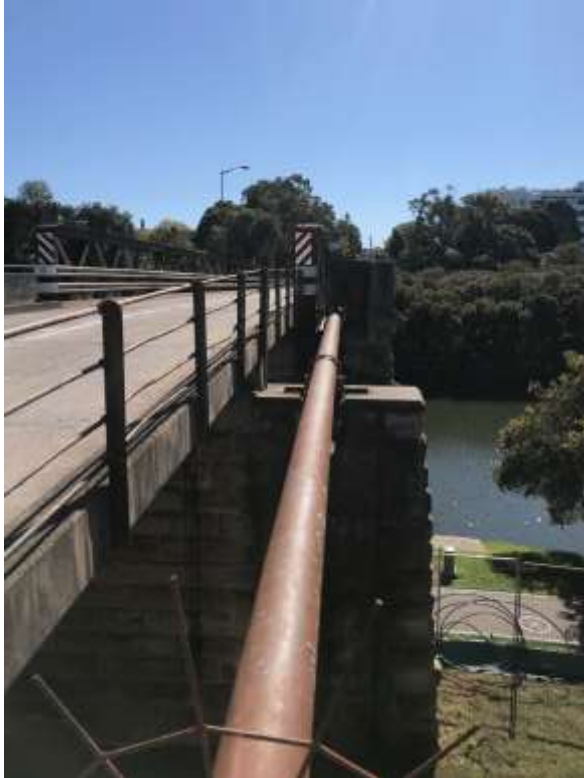
Photo 3-3: Redundant Jemena Gas main facing north
