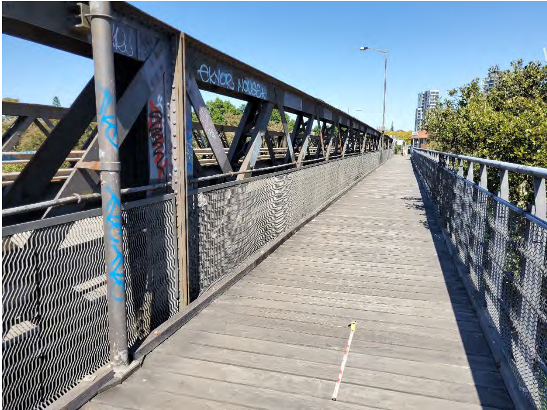
Figure 5.20 South facing view showing examples of graffiti present along bridge.
