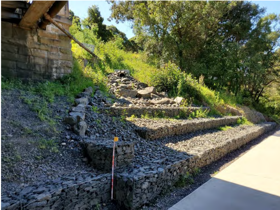
Figure 5.7 North-east facing view showing modern retaining wall and storm drain below bridge.
