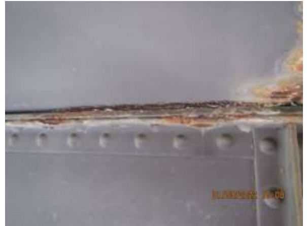
Photo 3-2: Example of section loss on cross girder
