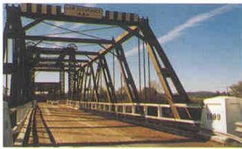
This large 1899 timber truss bridge at Woodville (A3) is one of only 2 overhead braced Allen trusses in service, the other is the nearby Morpeth Bridge (A1)
