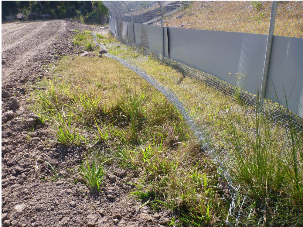
Photograph 3.4 Complete Fauna Fencing At Boat Harbour Creek with Floppy Top Grid Mesh, Fine Mesh and Metal Panels
