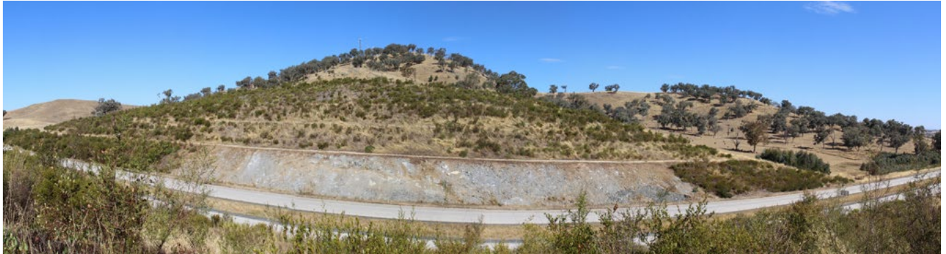
Revegetation on this cutting at Woomargama Bypass includes the cutting face, edges along the drains, rollover the bench hinges, and dense tree copses at the base of the leading and trailing slope transitions.
