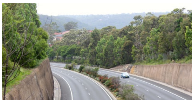
This part of the corridor had trees planted in a steep batter above a vertical cutting face with a long drop onto the carriageway. Particularly during establishment this was a maintenance problem and safe access to maintain the landscape works required ropes for safety. More space at the base to allow access by a platform, a lower height cutting or a railing would have improved the inherent safety of workers needing to access this site.
