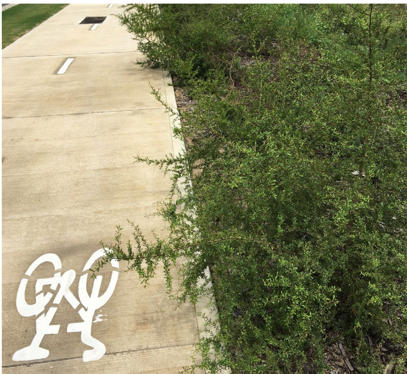
Do not use vegetation with spikes or thorns along paths, cycleways, near bus stops, along maintenance access ways or other locations where they could cause injury, such as this Bursaria spinosa along a shared use path.
