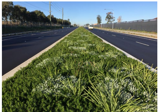
On narrow medians, generally less than seven metre, a higher density of ground cover planting is required to minimise maintenance and provide an attractive weed free appearance.
