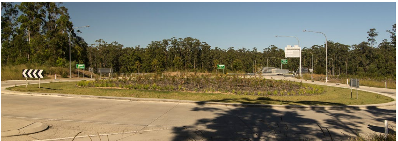
Roundabout showing layout which maintains good sight lines, well considered drainage and a surface treatment which is self-recovering catering for large vehicles.
