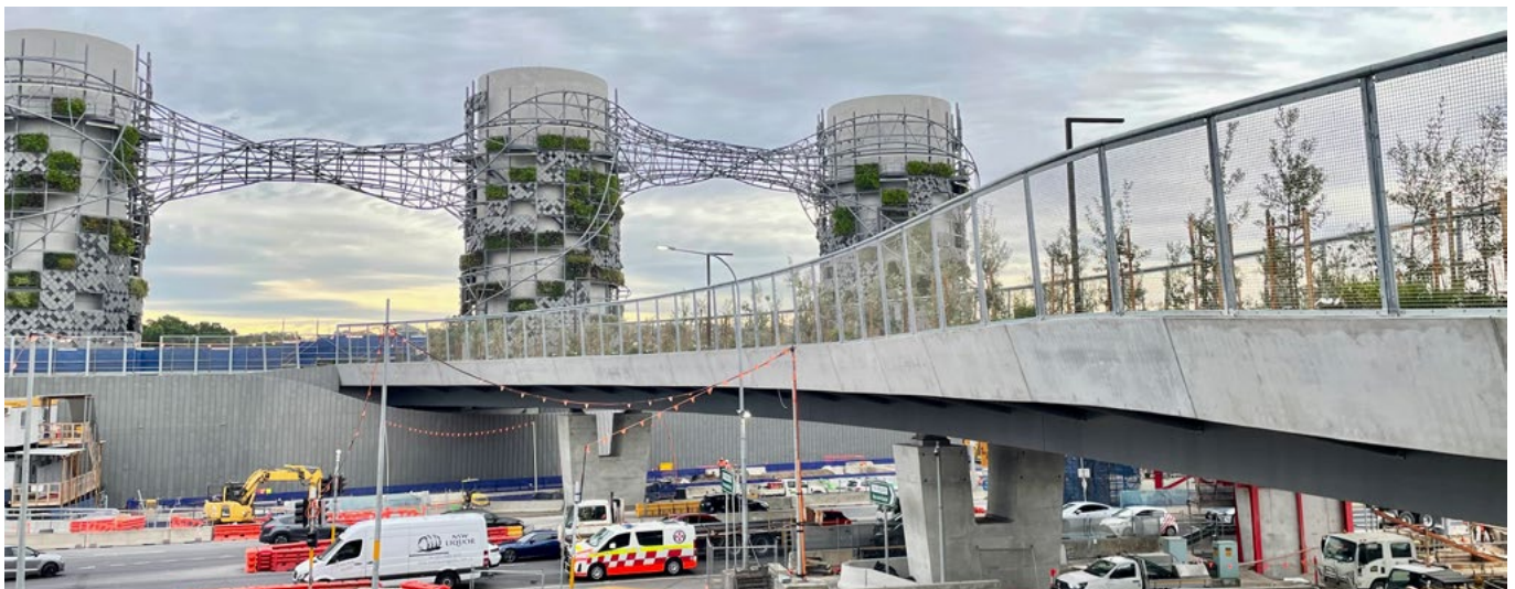
Landscape on walls, buildings and bridge structures at Rozelle (unfinished project as at May 2023). Green panels have been used as part of the design of the ventilation outlets to visually break down the structure and integrate it into the parklands. Trees and shrubs have been planted into deep soils on the bridges and buildings to extrude the parkland landscape and character across the wide and busy road, linking suburbs.
