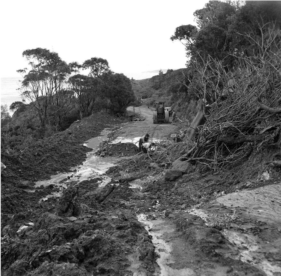
Cleaning up damage after the 1950 storm
