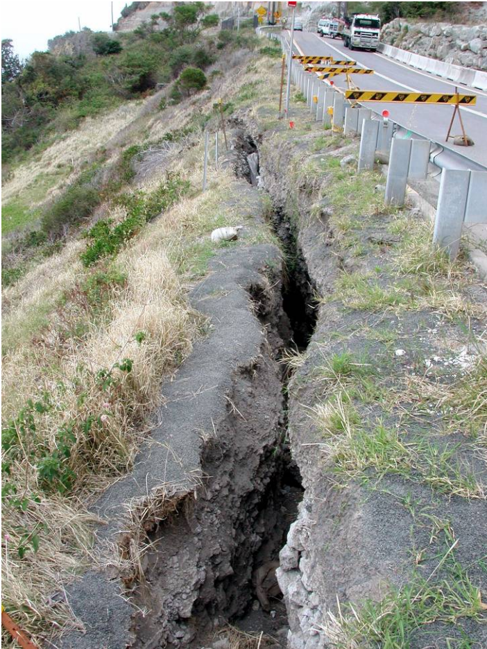
Crack in embankment, November 2003
