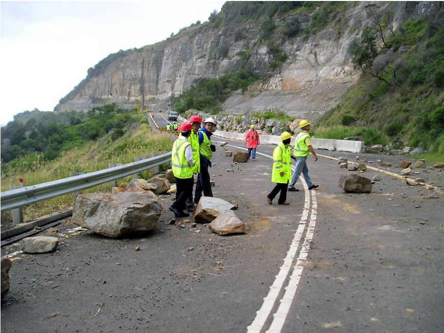
Rock fall, March 2004
