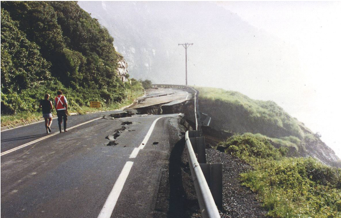
Damage to Lawrence Hargrave Drive after 1988 storm (Photo by Ron Draper)
