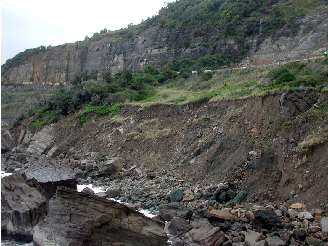
Embankment collapse, June 2003
