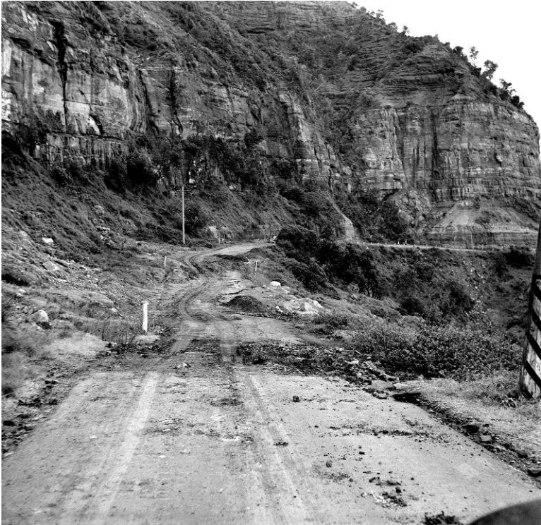
Ruined section of road, 1965
