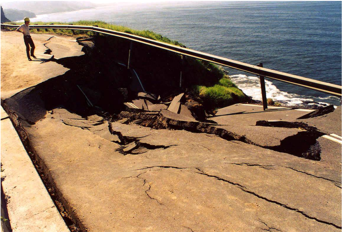
Close up photo of road slippage
