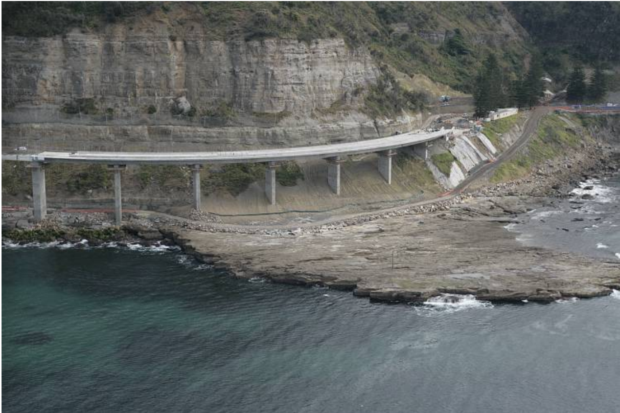
Northern incrementally launched bridge (casting area on right; launching nose on left)
