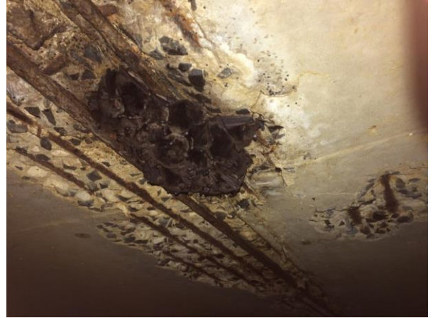
Southern Myotis roosting on exposed reinforcement on the obvert of a culvert. Credit: Kate Dallimore.
