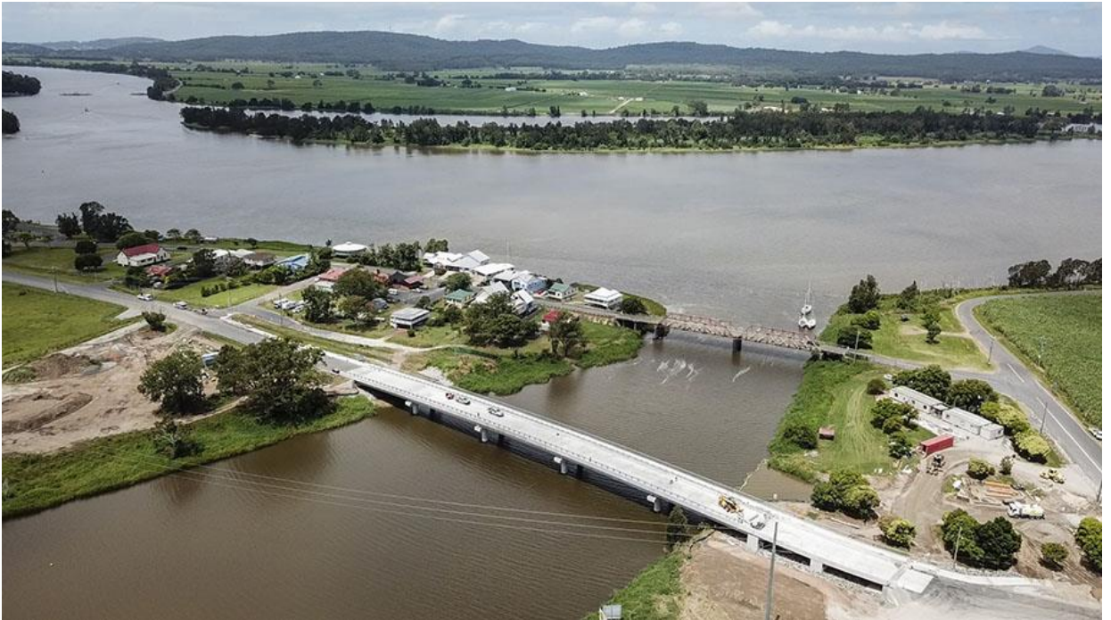
Sportsmans Creek bridges old (top) and new (bottom) prior to demolition of the old bridge. Credit: Transport
