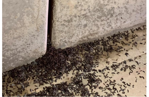
Guano at the base of a culvert join, indicating bat presence. Credit: Kris Le Mottee
