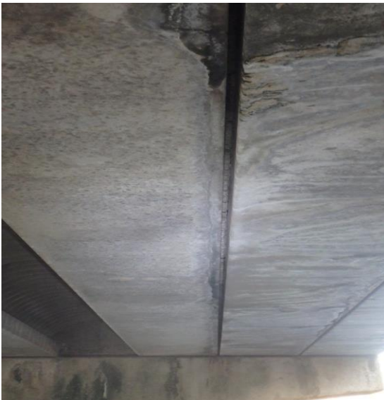
Expansion joint with staining from water leakage or microbat usage. Credit: Eco Logical
