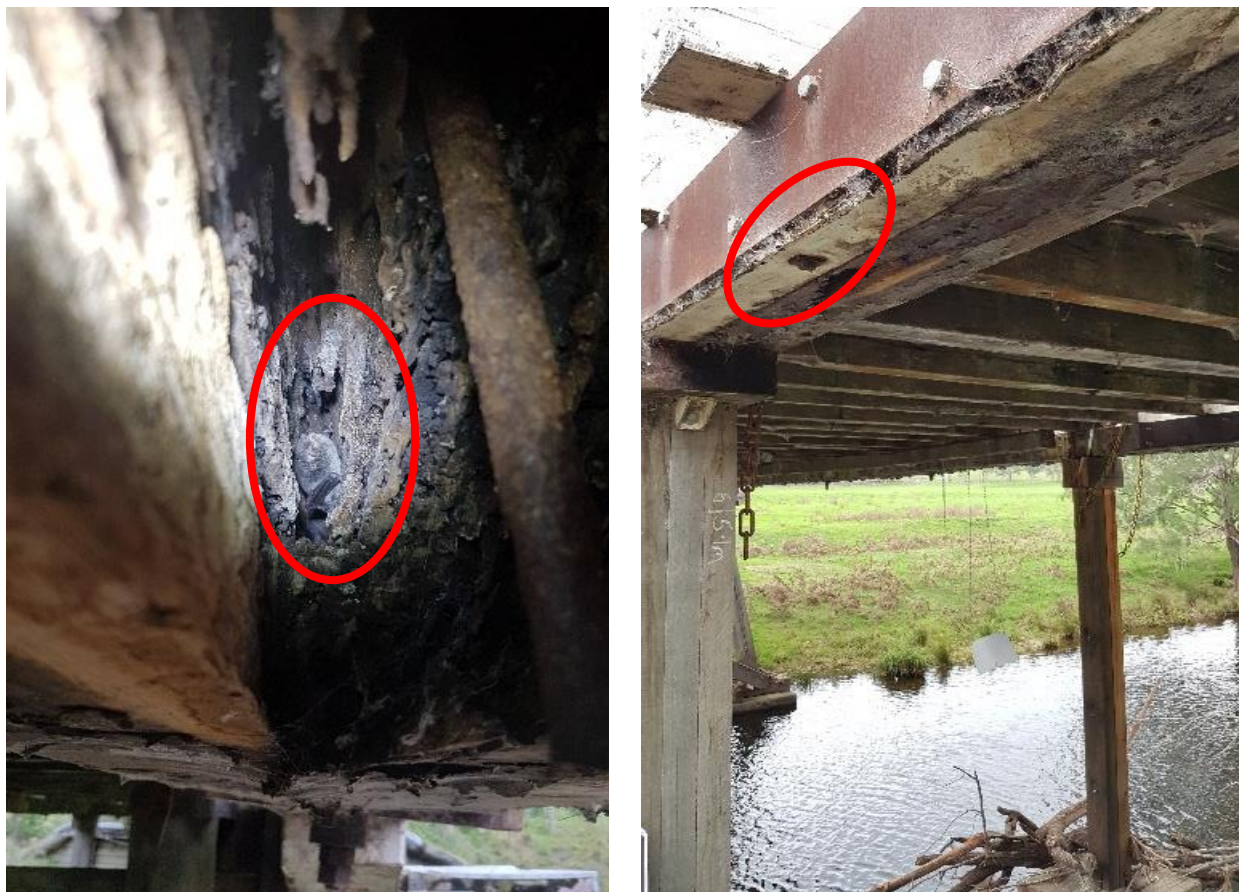
Figure 3: Southern Myotis roosting in rotted timber in Monkerai Bridge. Credit: Transport
