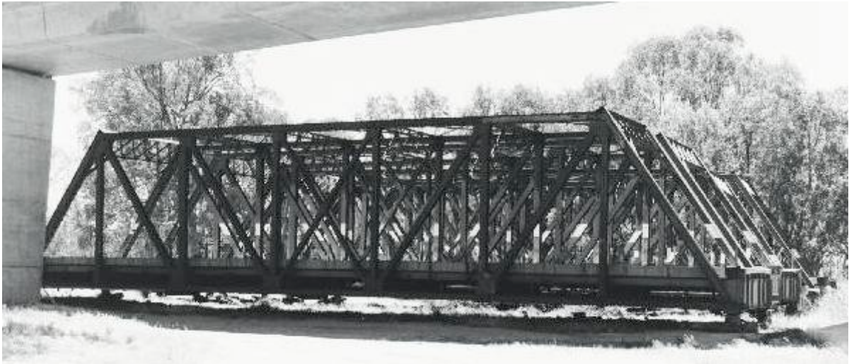
Figure 4.21 The four steel Warren trusses of the former Mildura Bridge after dismantling in 1986
