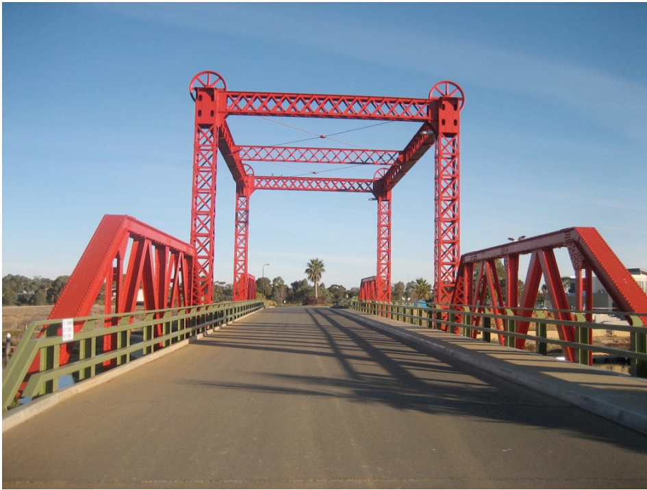
Figure 4.22 The lift tower and two heavily modified truss spans instated on a fixed span concrete bridge at the Mildura Marina (Source: GHD)
