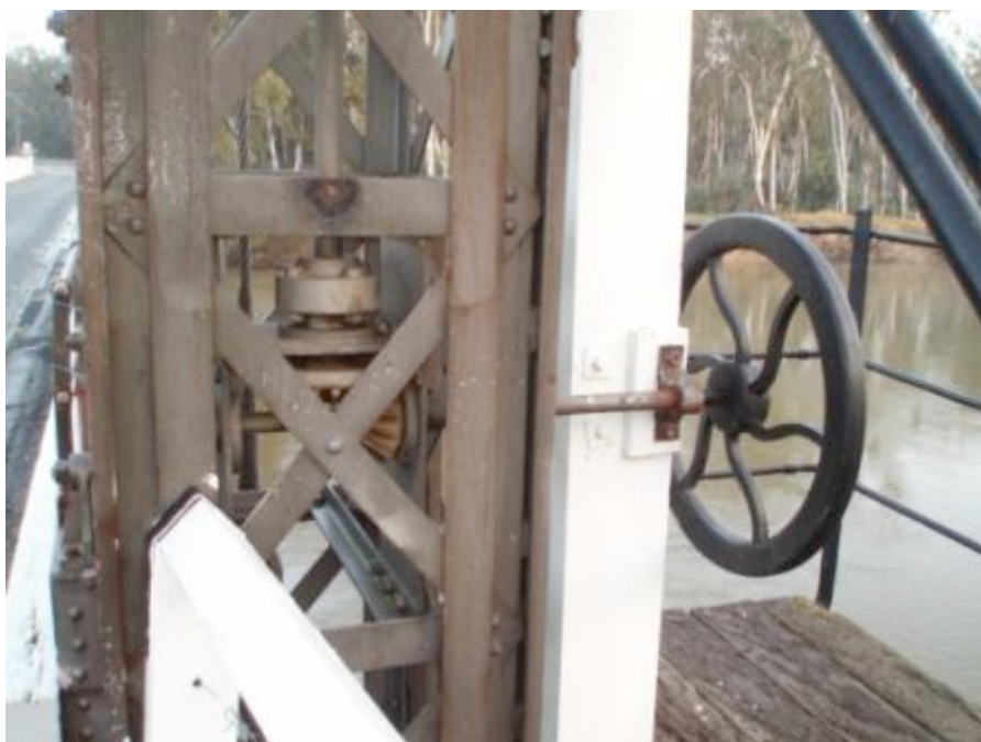
Figure 5.54 Cobram Bridge winch mechanism (Source: RMS)
