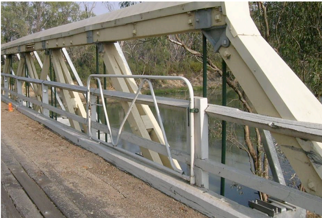
Figure 5.90 Pedestrian barrier attached to timber railing when not in use
