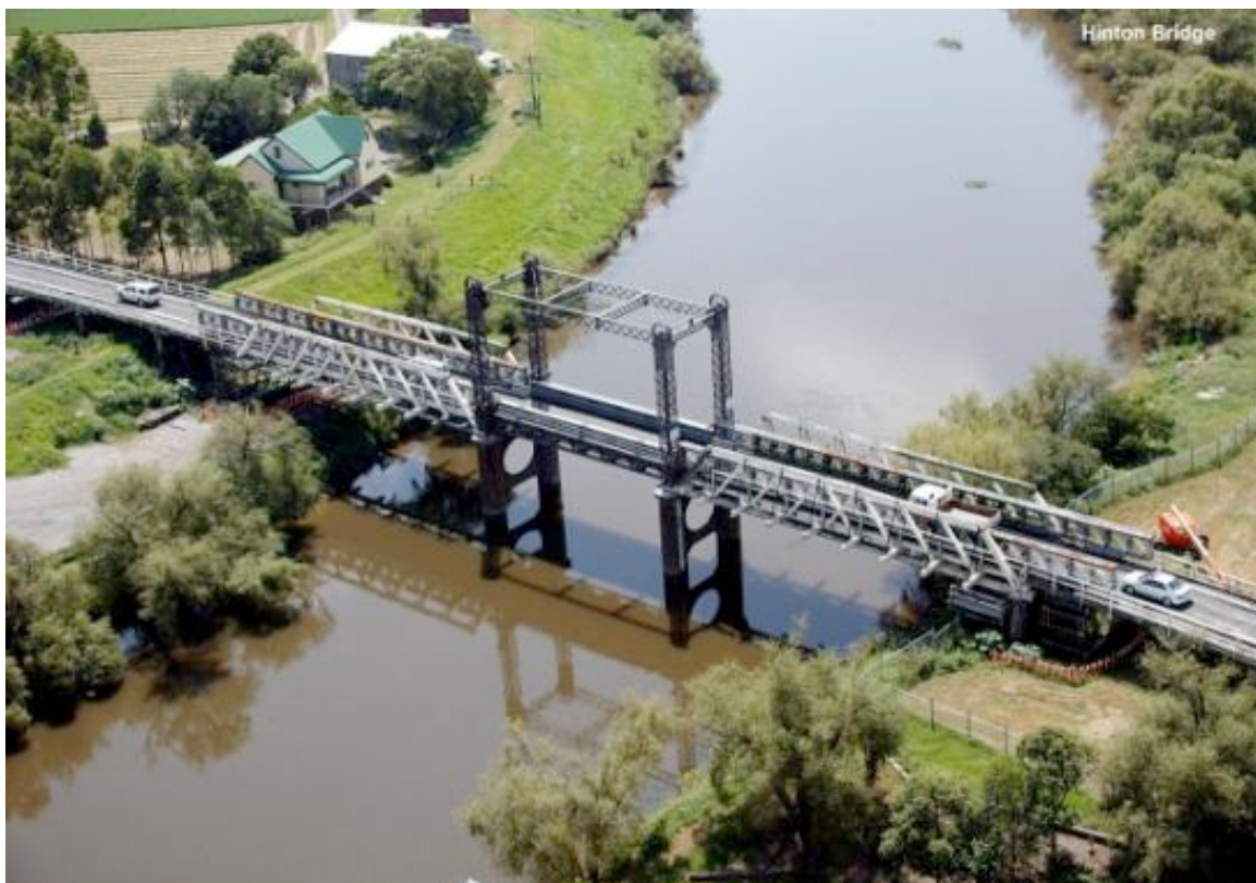
Figure 5.37 View of Hinton Bridge with Bailey support structures on truss spans in 2004
