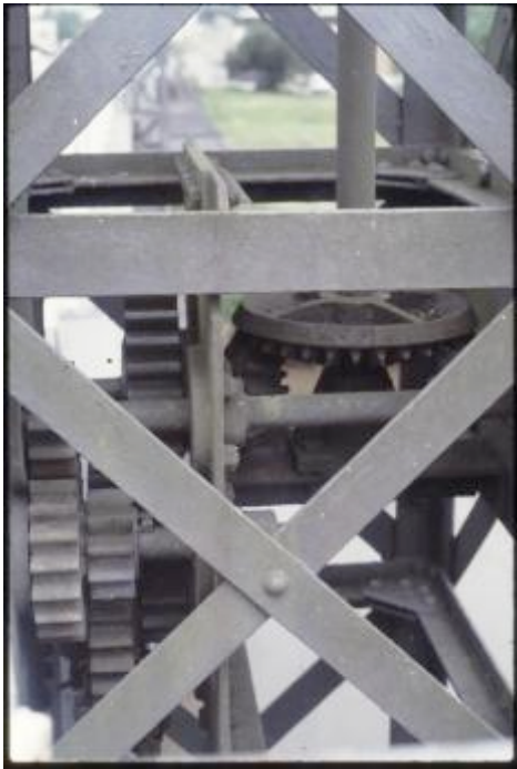
Figure 5.43 Hand operated winch mechanism (Source: RMS)
