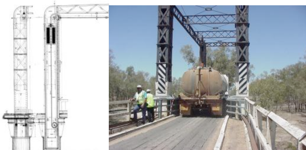
Figure 5.5 Drawing and image of lattice towers and Warren type longitudinal bracing girders on Brewarrina Bridge (Source: RMS)
