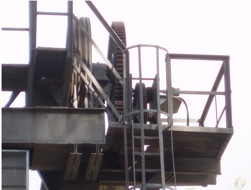
Figure 5.100 Winch and sheave mechanism for Gonn Crossing (Source: RMS)
