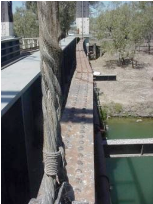
Figure 5.4 Steel girder supporting damaged movable span (Source: RMS)
