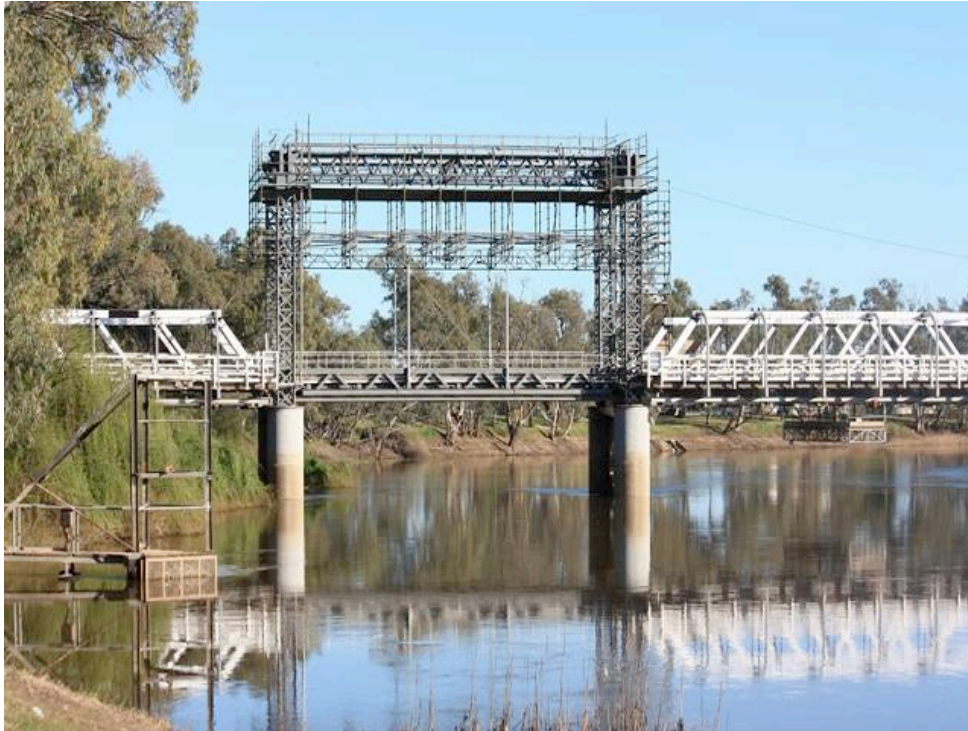
Figure 5.19 View of the scaffolding in place on the bridge between 2009 and 2012 to facilitate repainting of lift tower and replacement of mechanical components
