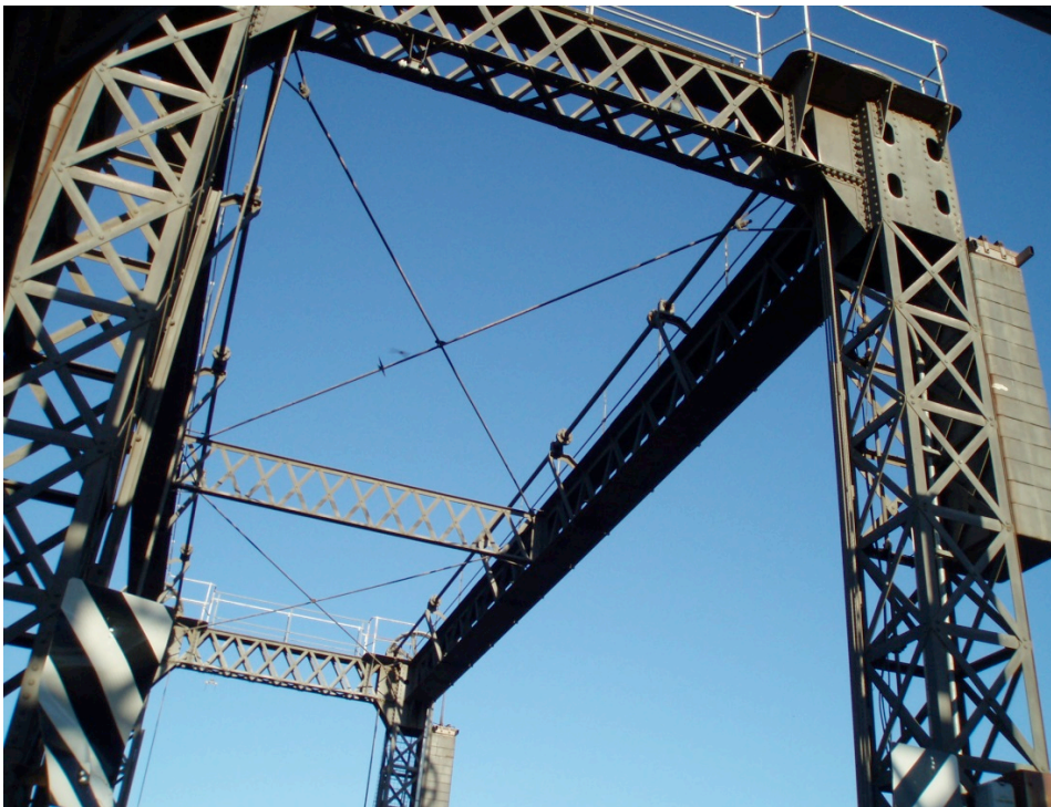
Figure 5.106 Abbotsford lift towers (Source: GHD)
