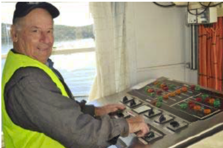
Figure 5.162 George Merceica at the control panel within the engine house of the bridge (Source: Bay Post, May 2, 2012)
