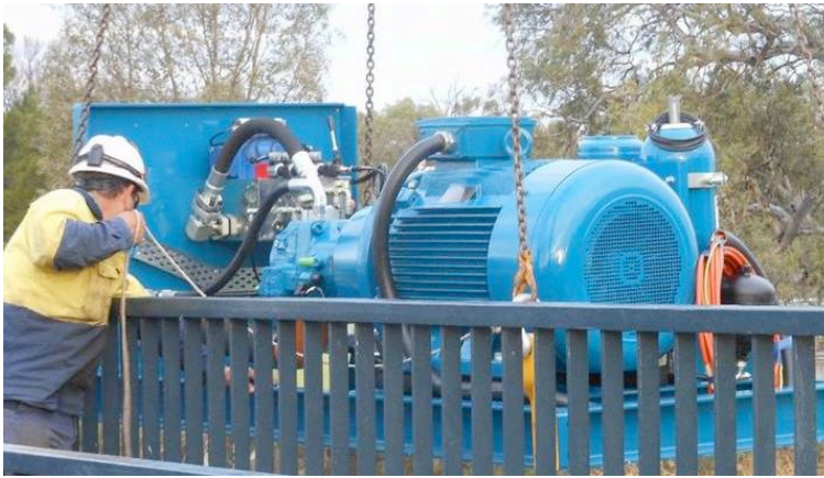
Figure 5.214 New motor installed to power hydraulic cylinders and electrical components on bridge
