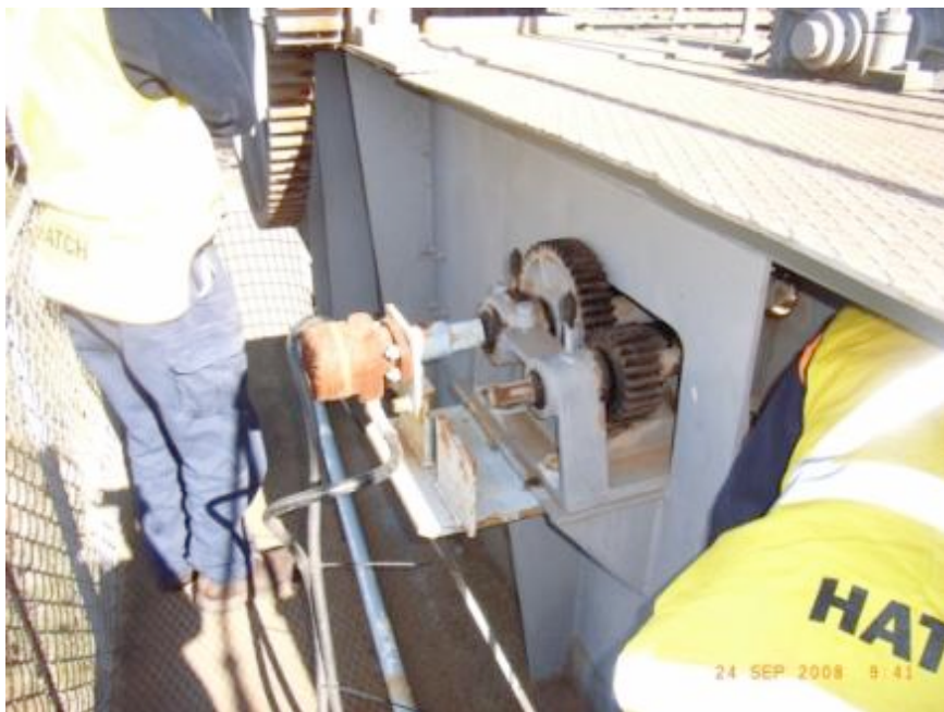
Figure 5.145 Hydraulic motor on Nyah Bridge (Source: RMS)
