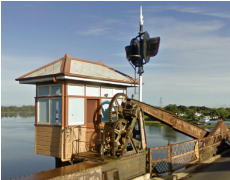
Figure 7.53 Image of Grafton Bridge control cabin
