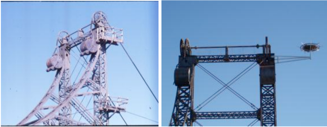
Figure 7.4 Top of tower span of Glebe Bridge with Osprey nesting basket shown at right
