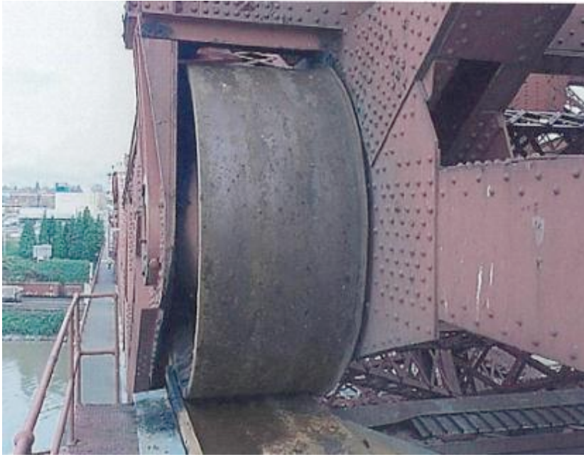
Figure 7.60 One of the Roll wheels on Broadway Bridge (Source: Tilly). The deck is suspended from this wheel
