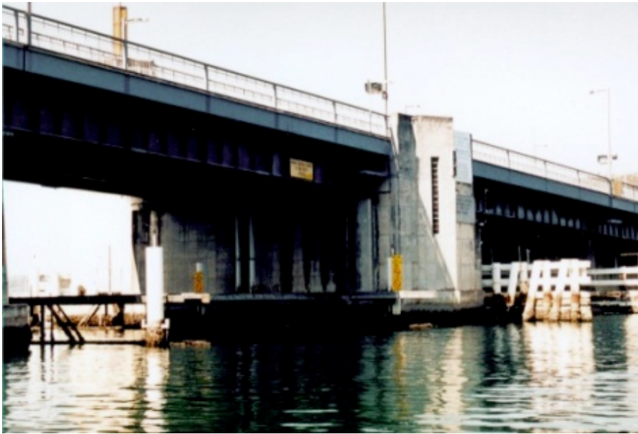
Figure 7.75 Pier 4 – Western end – This is the main pier that supports the Bascule Span (Source: Austral Archaeology Pty Ltd 2002)
