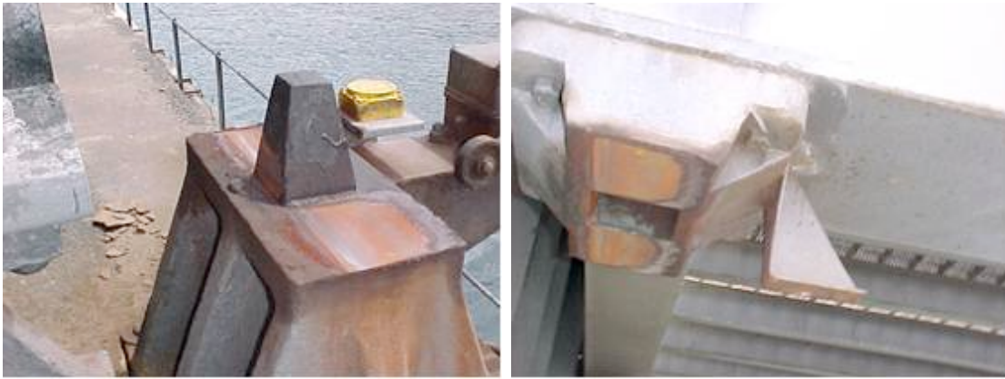
Figure 7.89 Detailed view of tapered wedge and opening on underside of bascule span (Source: 2006 Spit Bridge SOHI)
