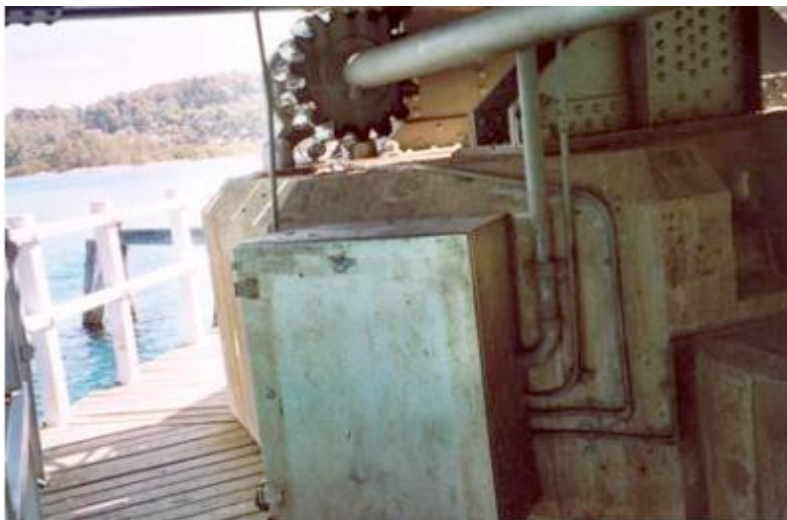
Figure 7.46 View of electric motor in steel casing located on the operating platform. The intermediate machinery drive can be seen above
