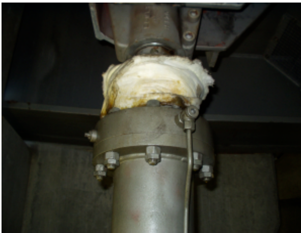
Figure 7.101 Hydraulic luffing cylinder on Swansea Bridge (1989) in poor condition (Source: Jenkins and Tilley, 2011)
