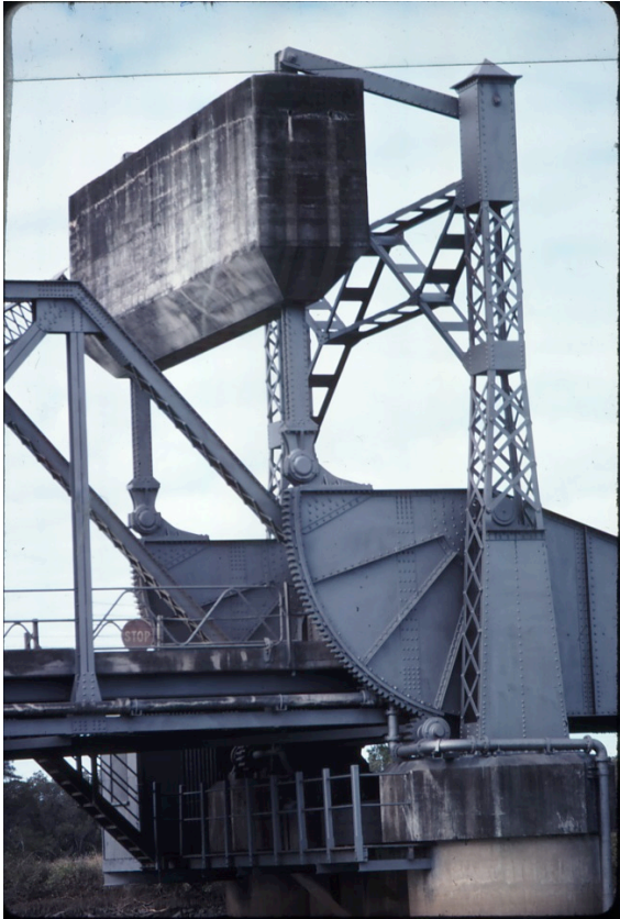
Figure 7.42 View of the trunnion end of the bascule span detailing the machine-cut racks on the curved ends of the plate girders
