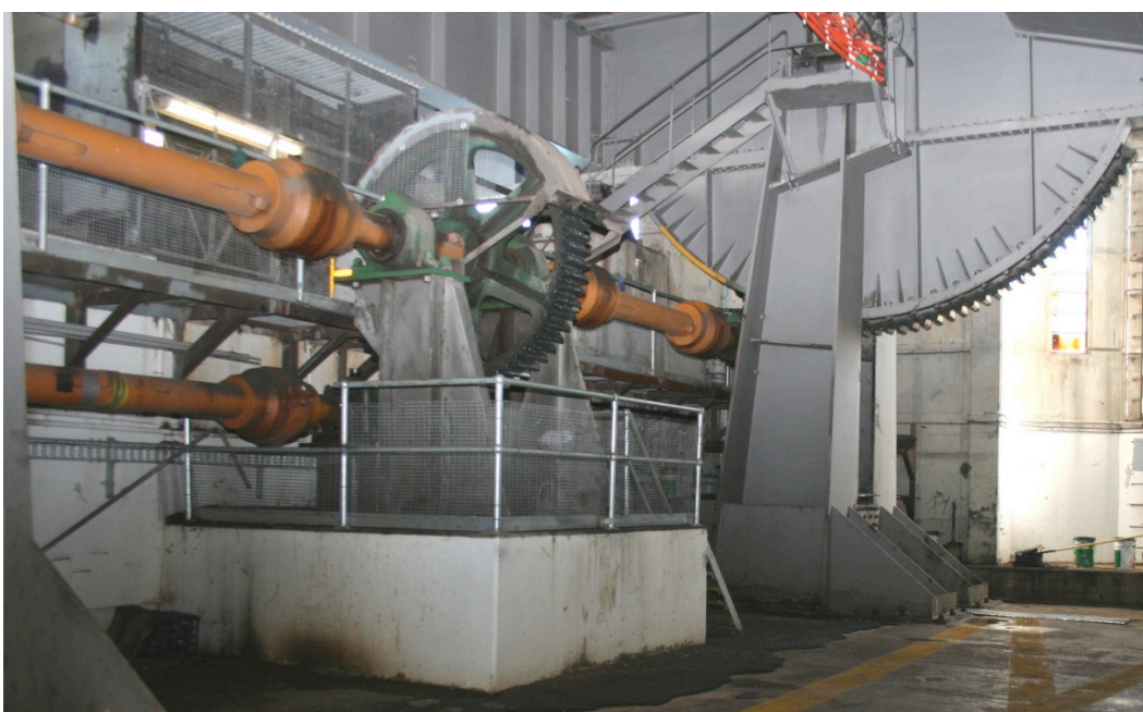
Figure 7.88 Centre gear, shafts and trunnion prior to 2012 upgrade
