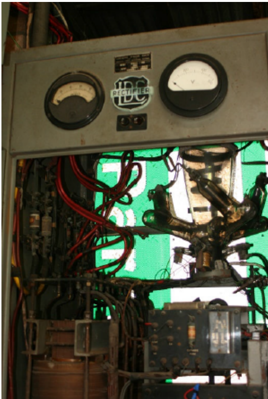
Figure 9.24 The Mercury Arc Rectifier Cabinet, with the door open and the glass bulb upper right with reactors, wiring and relays at the base. Manufactured by Lancashire Dynamo Coates Pty Ltd, of Goodwin Street, Richmond, Victoria. A silicon rectifier unit is mounted on the wall adjacent (Source: Brassil, 2011)
