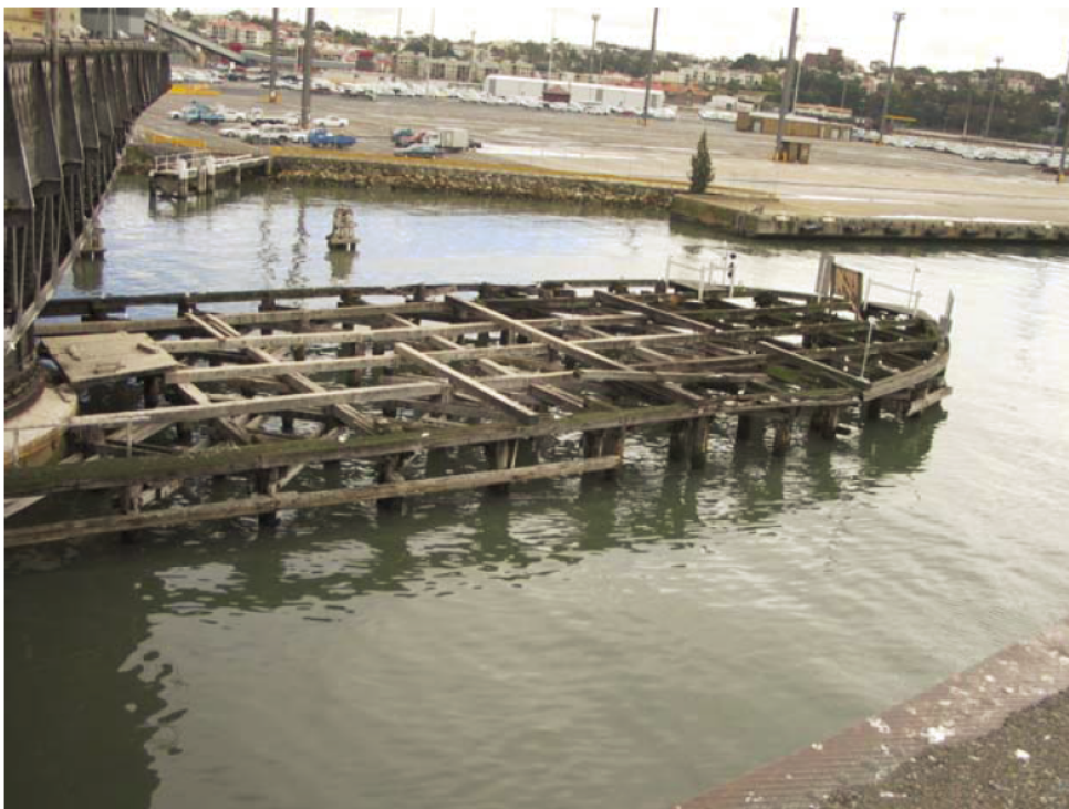
Figure 9.21 View of the southern end of the fender in 2012 prior to repair works
