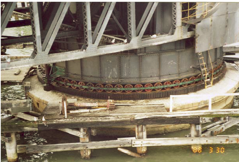
Figure 9.17 Glebe Island Bridge swing span drum. The main girders rest on the distributing girders and the drum pivots on the cast steel rollers
