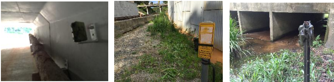
Plate 18: Underpass cameras were mounted on steel brackets & orientated to capture fauna moving along either the floor or rail (if present) of the culvert (L). Cameras were positioned either side of the rail track and inside the retaining walls during summer underpass monitoring (M). Underpass cameras needed to be positioned outside of the McGrath's creek culverts due to risk of inundation (R).
