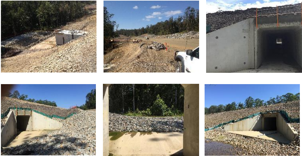
Plate 12: Design features and construction progress for Martells Road south fauna underpass. Photos on top row were taken during spring 2014 sampling and photos on the bottom row taken during summer/autumn 2015 sampling.
