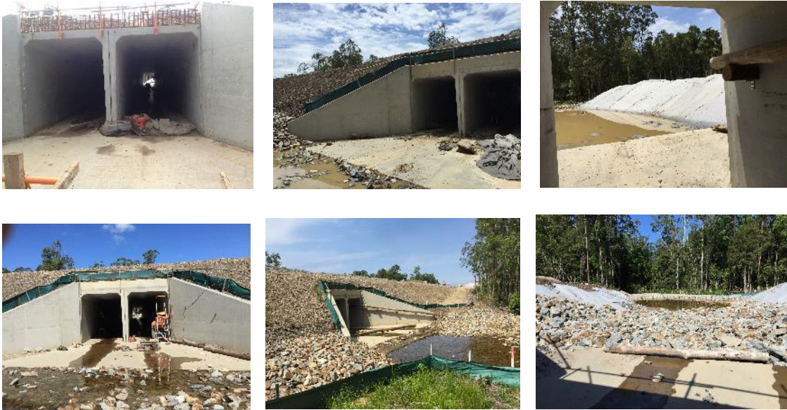
Plate 14: Design features and construction progress for Access Road G fauna underpass. Photos on top row were taken during spring 2014 sampling and photos on the bottom row taken during summer/autumn 2015 sampling.
