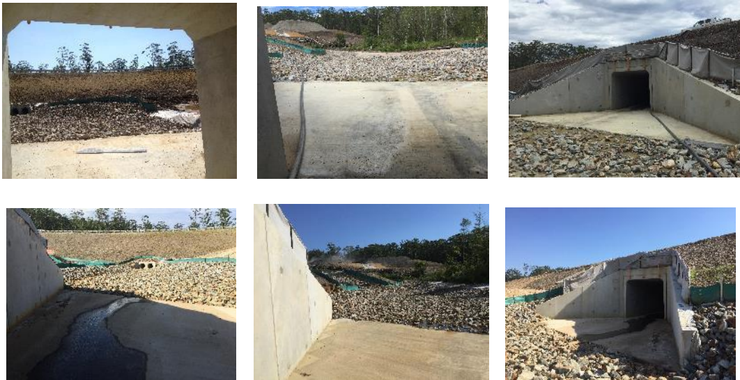
Plate 13: Design features and construction progress for Martells Road north fauna underpass. Photos on top row were taken during spring 2014 sampling and photos on the bottom row taken during summer/autumn 2015 sampling.
