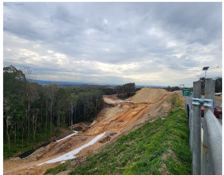
Image 8: Southern works at the cnr of McCaffery Drive and Lookout Road. All earthworks. View is to the north.
