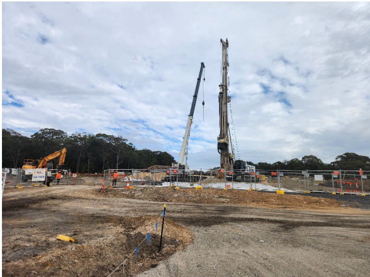
Image 1: Bridge pilling at the northern end, Jesmond Park. View to the south.
