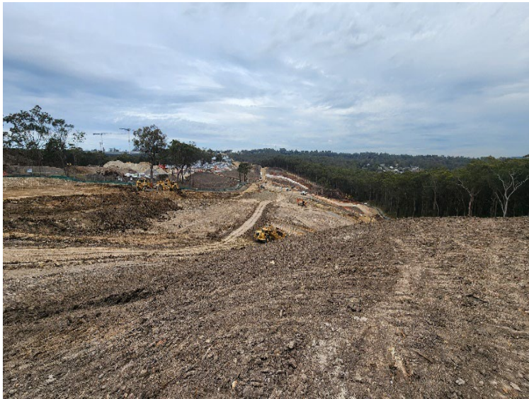
Image 5: Main line, eastern boundary (JHH) – general view of earthworks. View is to the south.
