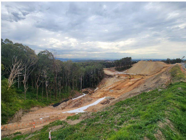
Image 7: Southern works at the cnr of McCaffery Drive and Lookout Road. All earthworks. View is to the north.
