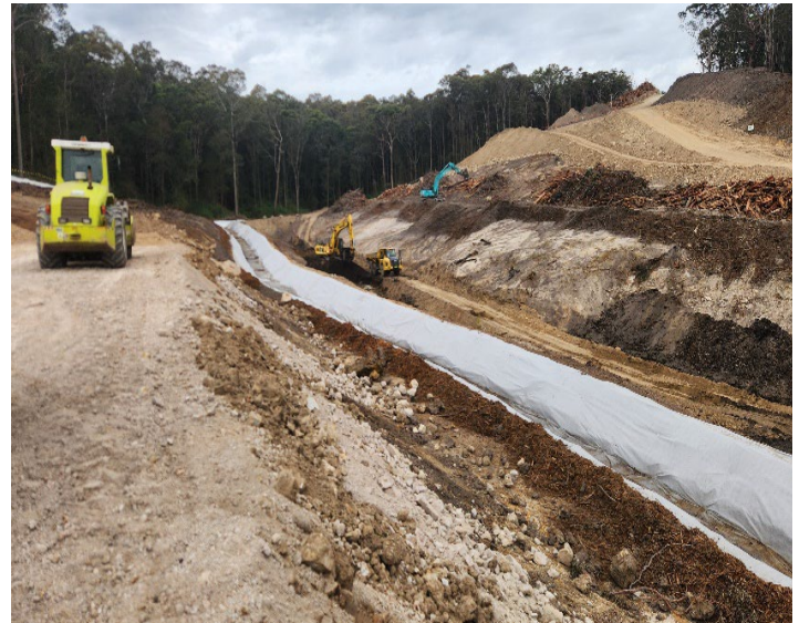
Image 6: Main line. Clean water drain collecting the eastern boundary perimeter water and taking it off site to the west, while a culvert is installed. View is to the southeast.
