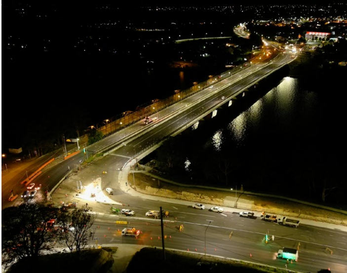
Crews worked at night to prepare for the traffic switch onto the new bridge.
