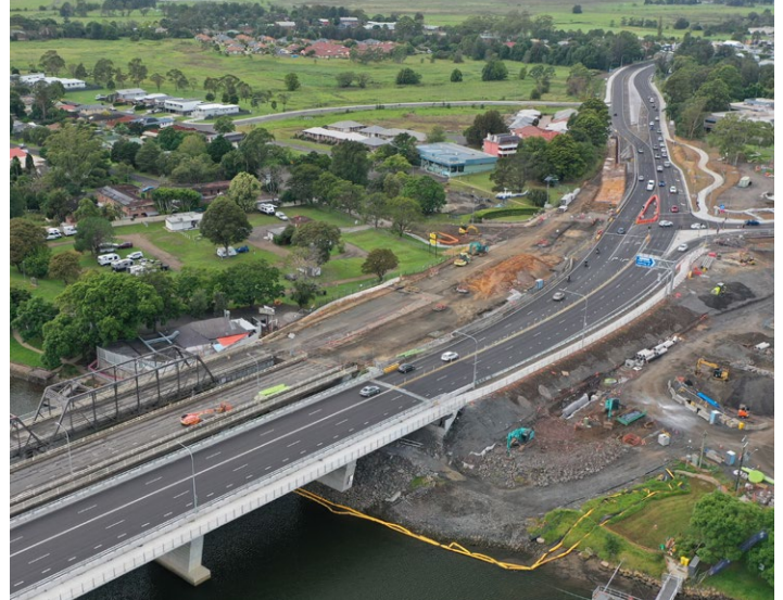
All traffic is on the new bridge while work is under way to replace road pavement south of the existing bridges.
